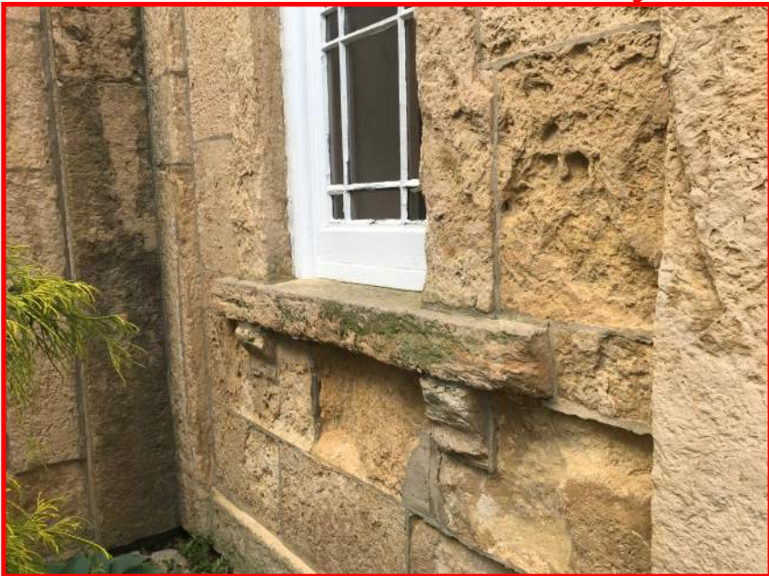
Gates of Heaven detail of stone condition and appearance. Also note window condition.
