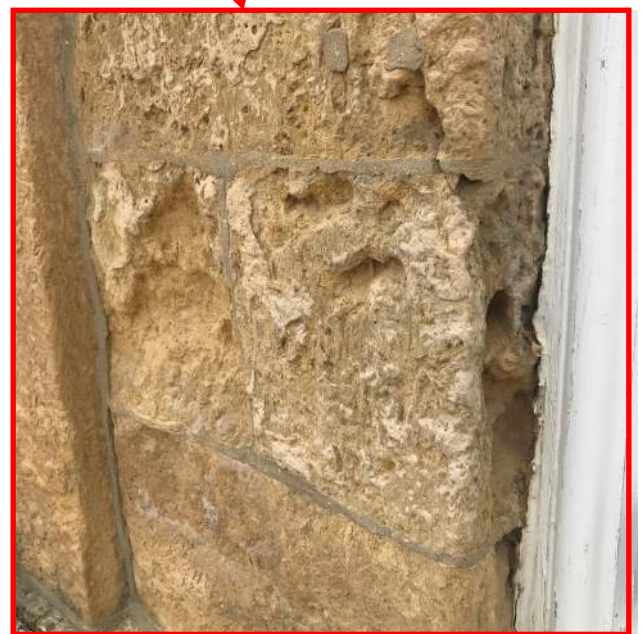
Gates of Heaven detail of stone condition and appearance at the front entrance.
