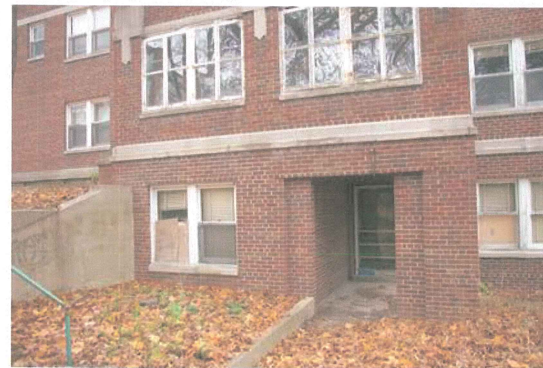
Image 5 Dormitory for Help - exterior wall to be retained below water table and window opening infilled with salvaged and interpretive materials.
