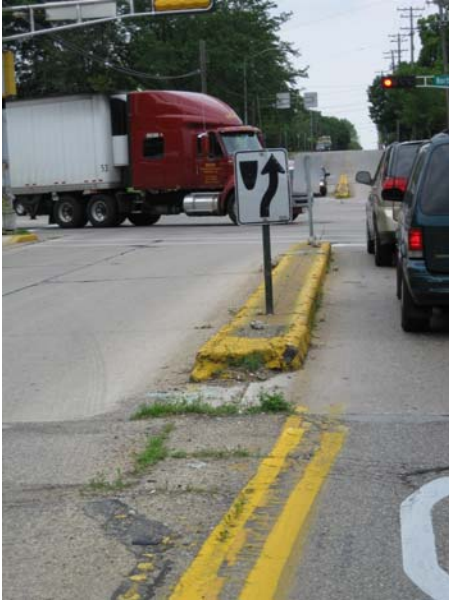
Crumbling median, Sherman Ave at Northport
