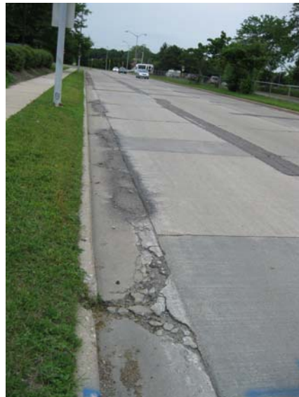
Patched and crumbling pavement, Northport Drive near Dryden Drive
