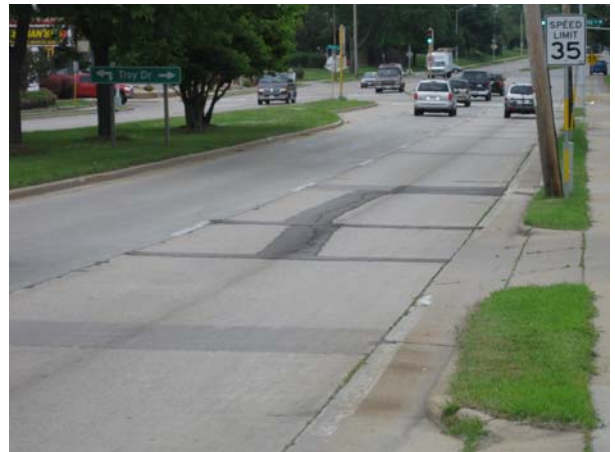
Cracked, patched pavement and leaning utility pole, Northport Drive near Troy
