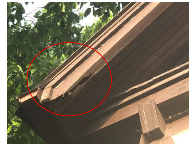
ROTTING FASCIA BOARDS
