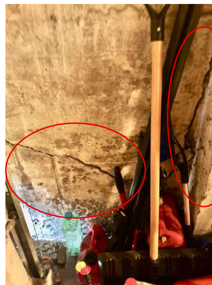
CRACKED FOUNDATION INSIDE GARAGE
