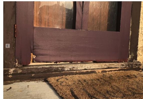
ROTTED SILL AND BASE OF STORM DOOR
