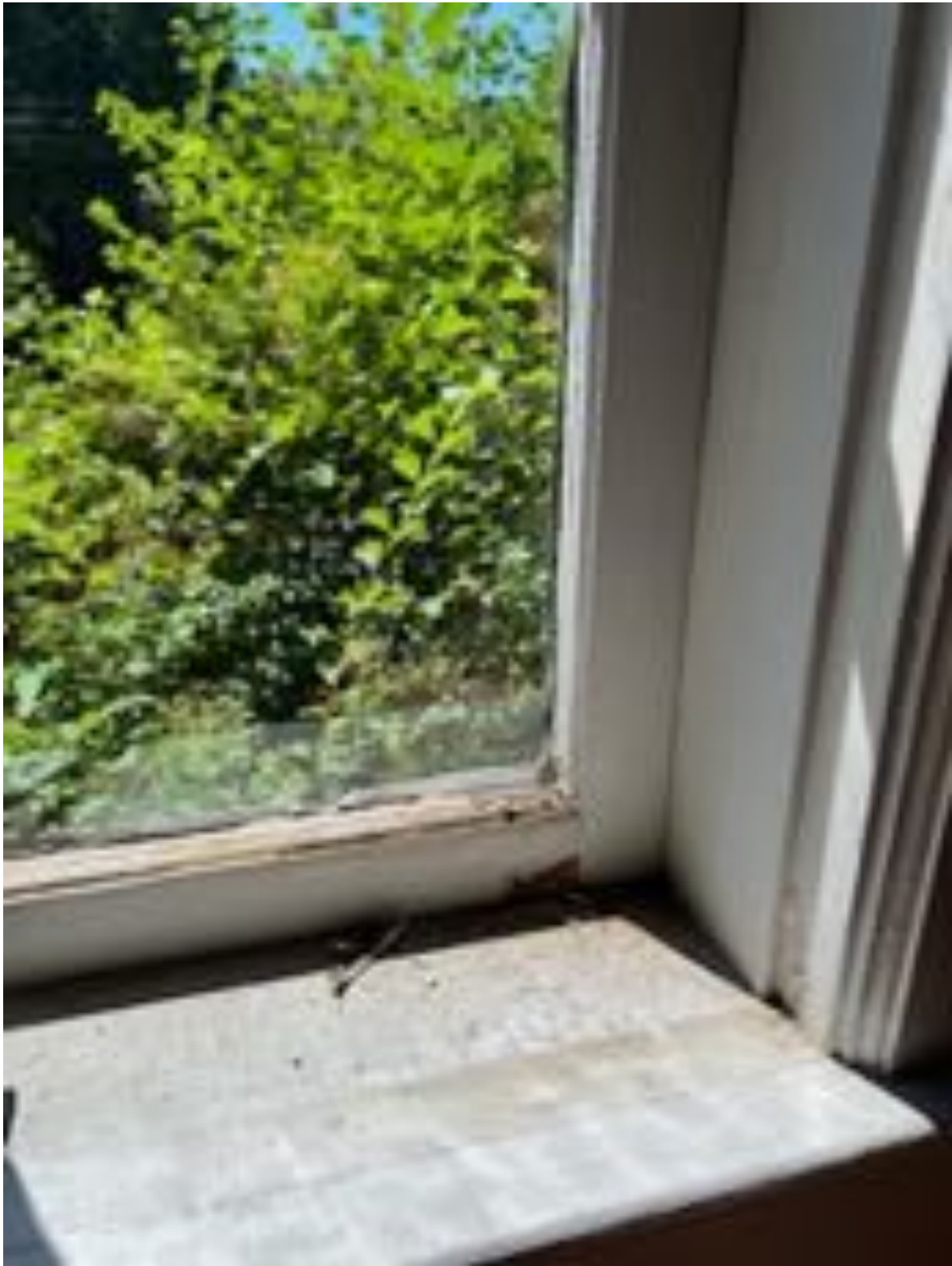
Window #2 – Deterioration of lower rail and rail/stile joinery evident.
