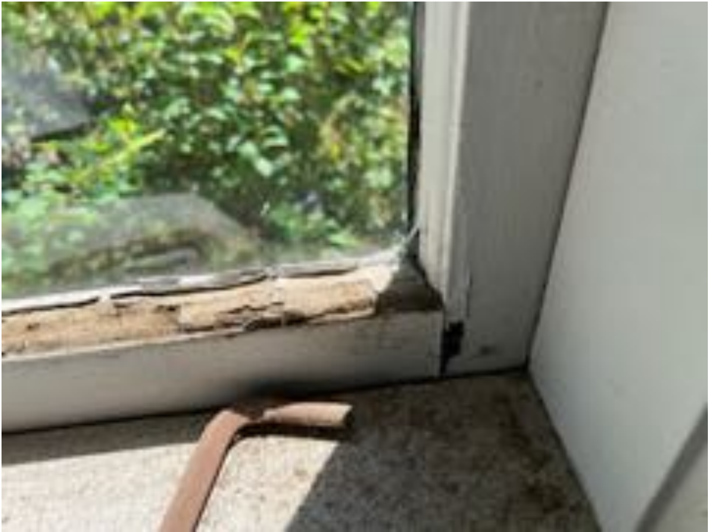
Window #3 – Interior view documents the sticking deterioration along with sash joinery failure.
