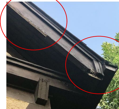
ROTTING FASCIA BOARDS
