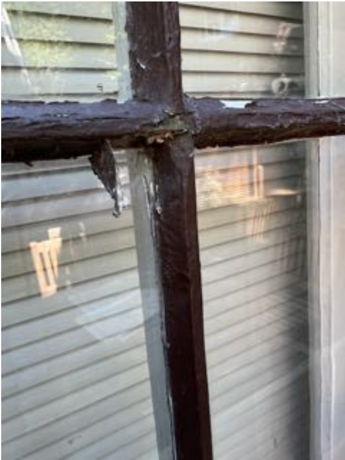
Window #3 – Exterior muntins & glazing needs complete replacement. Deterioration of underlying wood requires more aggressive rehab to get to suitable paint substrate.
