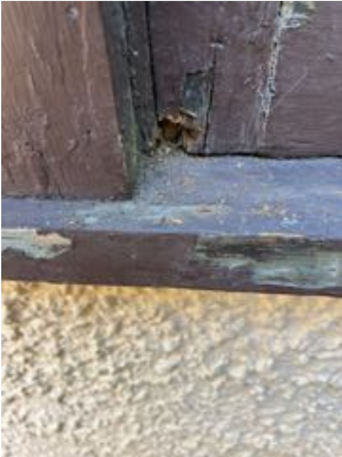
Window #3 – Exterior view of the 2-wide casement. Note exterior sill has lost thickness to deterioration. Lower end of stile has rotted away all the way back to the rail tenon compromising joinery strength.
