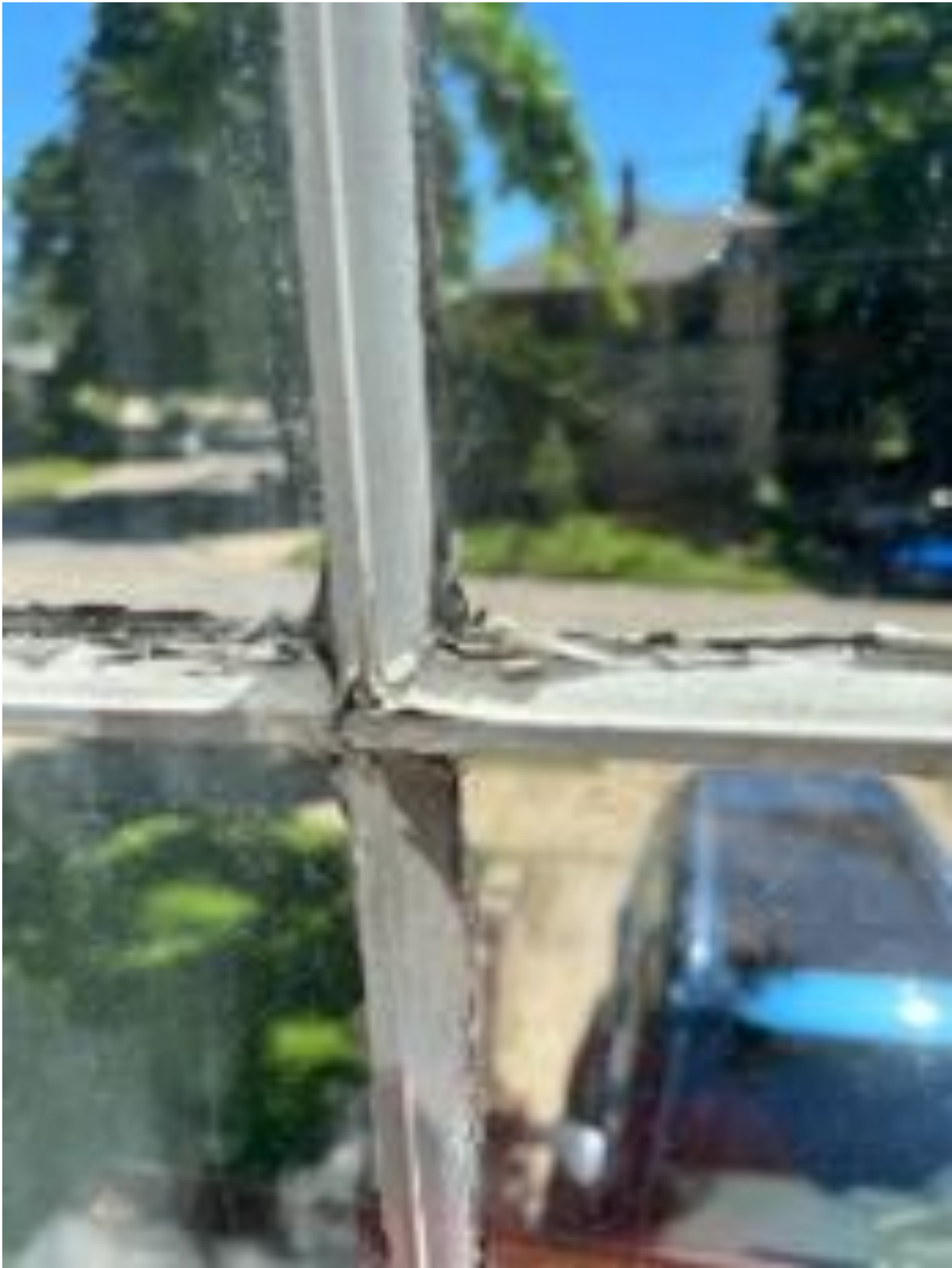
Window #2 – Interior paint deterioration.
