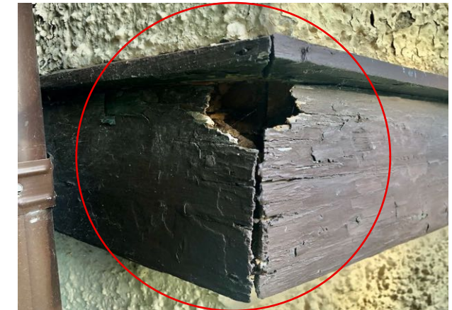
ROTTING DRIP EDGE AND BRAND BOARD AT WATER TABLE DETAIL
