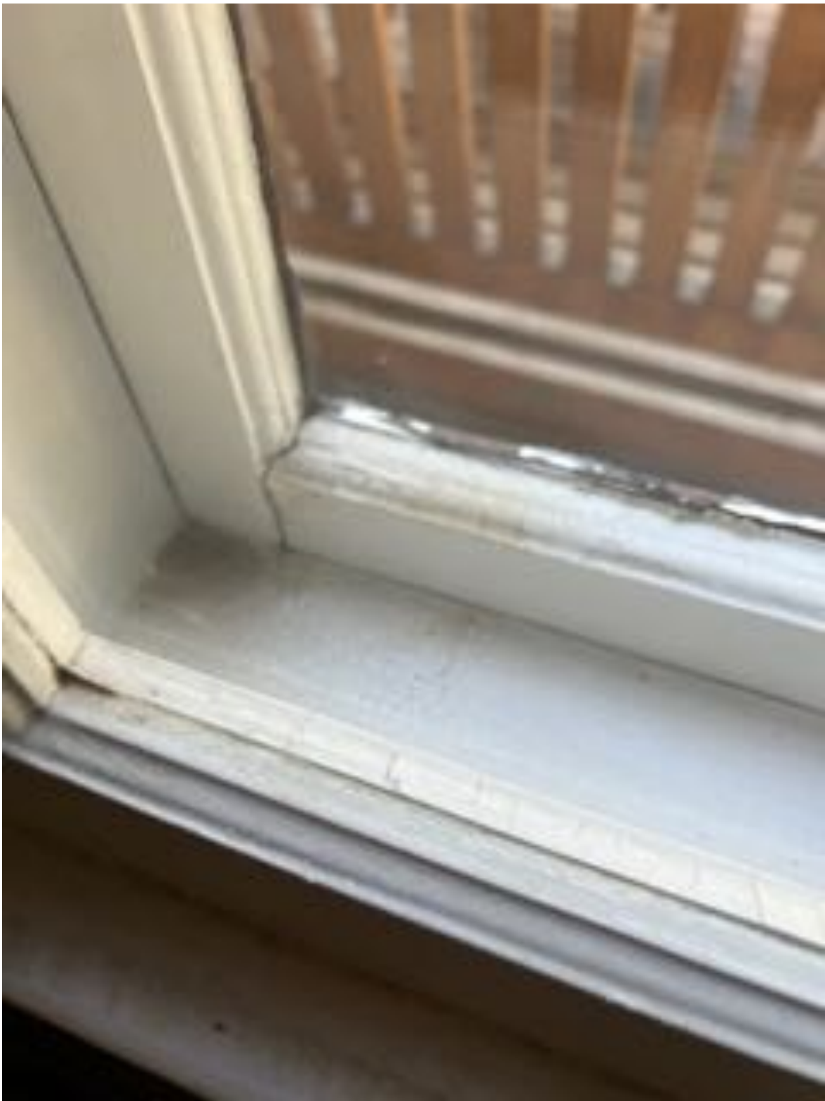
Window #3 – Interior view also suggest rail/stile joinery failure.
