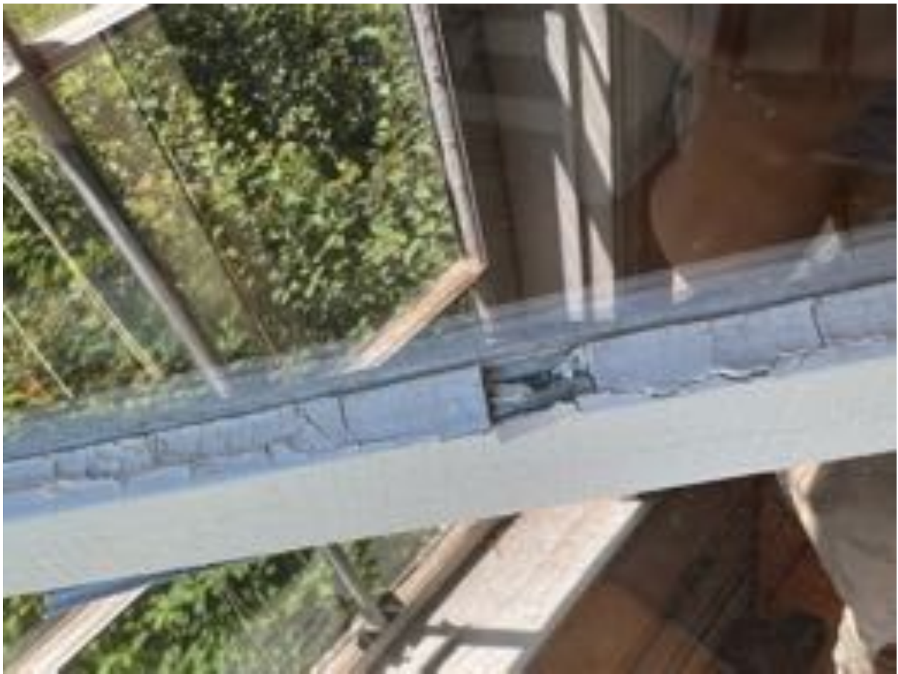
Window #2 – Exterior glazing deterioration.
