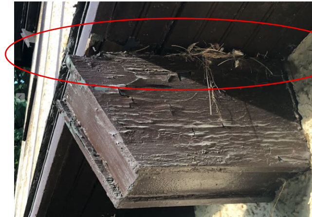
EXAMPLE OF CORBEL FALLING OFF HOUSE (BIRD'S NEST IN THE GAP)
