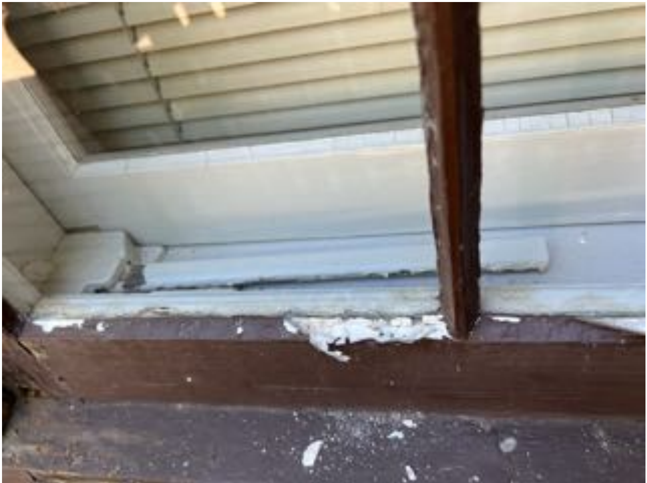
Window #3 – Another exterior showing glazing failure and, in the lower left, degradation of the rail/stile joinery.
