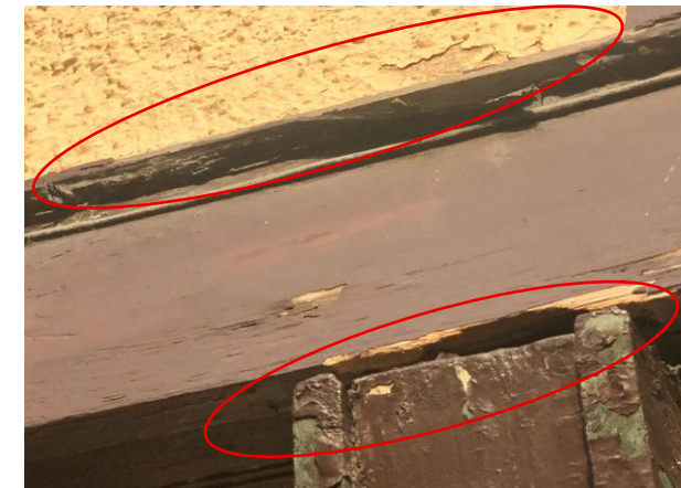
ROTTING DRIP EDGE AND FASCIA OVER BRACKETS
