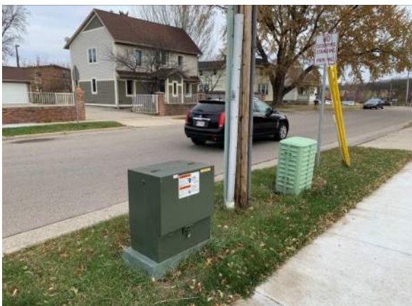
Photo 5: Pad-mounted transformer along Hughes Place north of the Site and residence beyond. Photo facing northeast.
