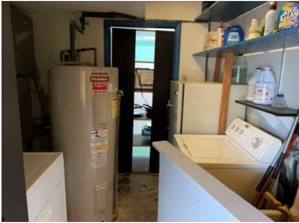
Photo 15: Laundry and mechanical room along the western interior wall of the building.
