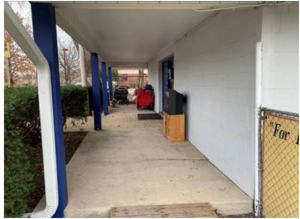
Photo 8: Entrance to the building with various items stored under the overhang. Photo facing east.
