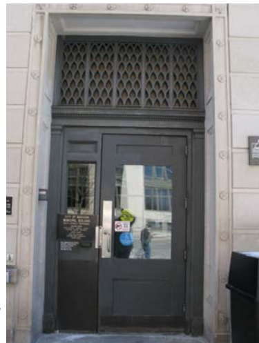
Figure 17 – Modified for Accessibility, the West Entrance still retains much of the Original Cast Iron Framing
