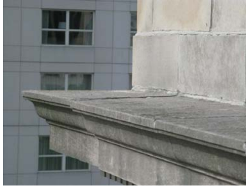
Figure 20 – All Four Major, Outside Parapet and Cornice Corners Show Slight Movement.
