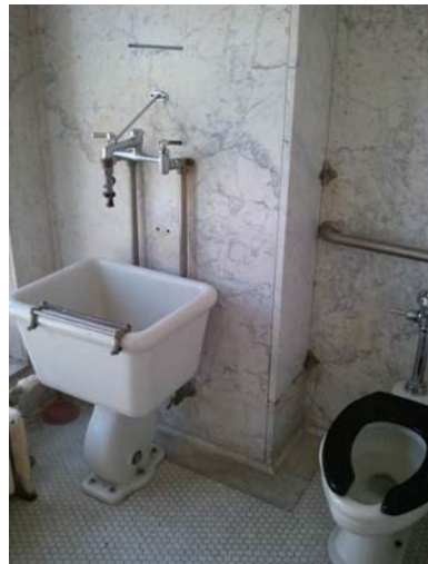
Figure 42 – Antiquated Plumbing Fixtures
