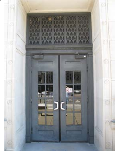
Figure 16 – Original Cast Iron and Steel Double Door and Transom Openings remain Intact
