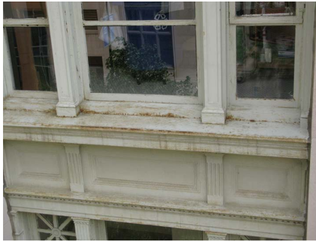
Figure 24 – Rust is Developing at Window Sills
