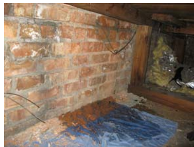
Figure 19 – Water Infiltration is occurring at the Raised Wood Roof Level.
