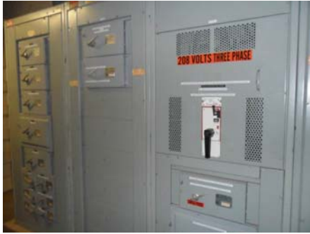
Figure 48 – Current Electrical Service
