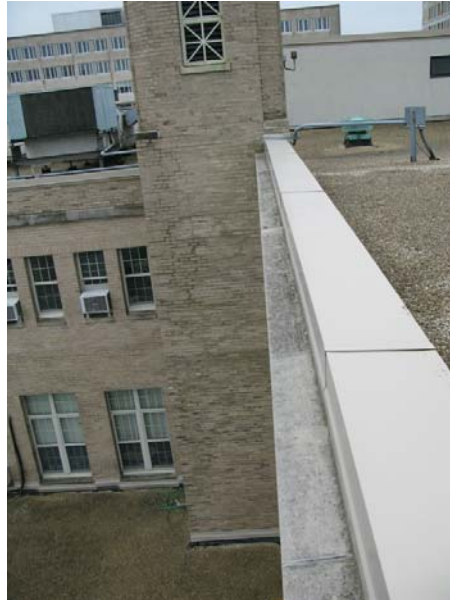
Figure 23 – Outside Corner of the Brick Chimney is Cracking Vertically on Both Sides
