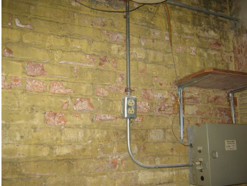
Figure 58 – Existing Brick Basement Wall Water Damage
