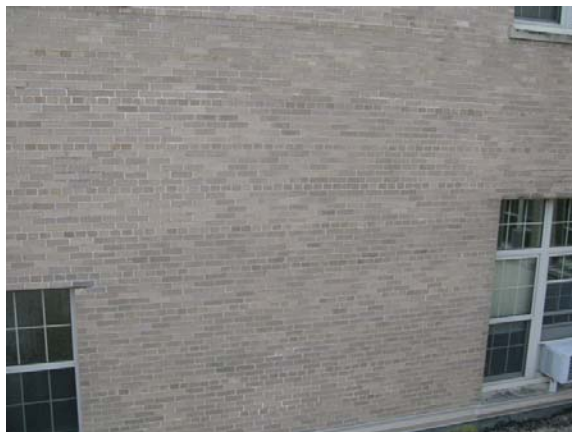
Figure 22 – Discoloration and Shifting of Brick indicates Rusting is occurring at the Hidden Relief Angles
