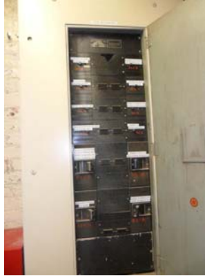
Figure 49 – Electrical Branch Panels
