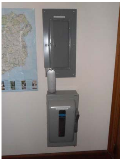
Figure 50 – Exposed Disconnect Electrical Device
