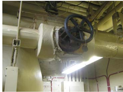
Figure 34 – Leaking Valve and Damaged Insulation
