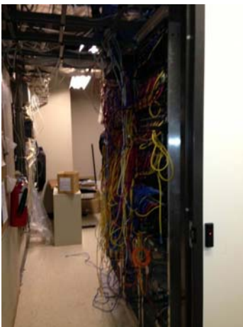
Figure 45 – First Floor Telecommunications Room
