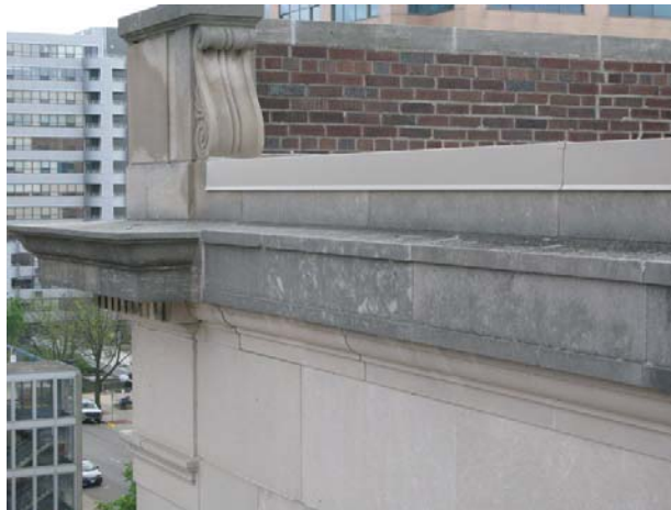
Figure 21 – Darkening of the Stone below the Metal Coping indicates Water Saturation
