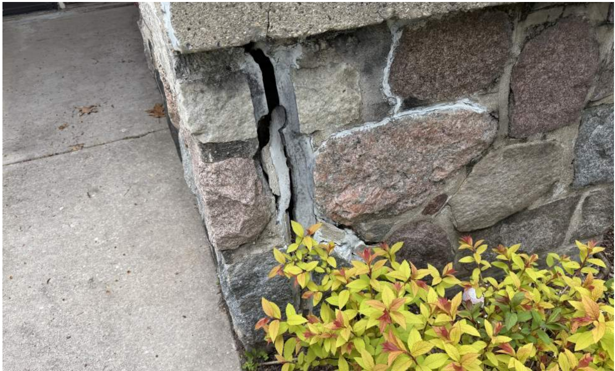
Detail of stone condition at entrance planter.
