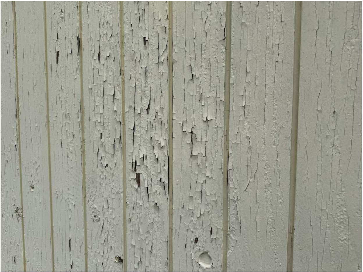
Detail of siding condition.
