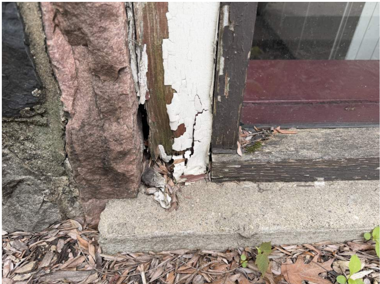
Detail of wall condition at entrance planter.
