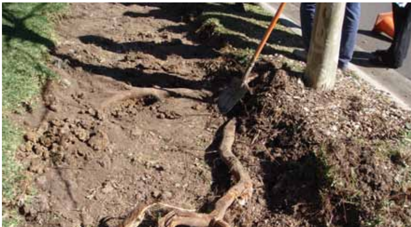
Fig 2.1.5 - Insufficient soil volumes produce damaging, shallow roots.
