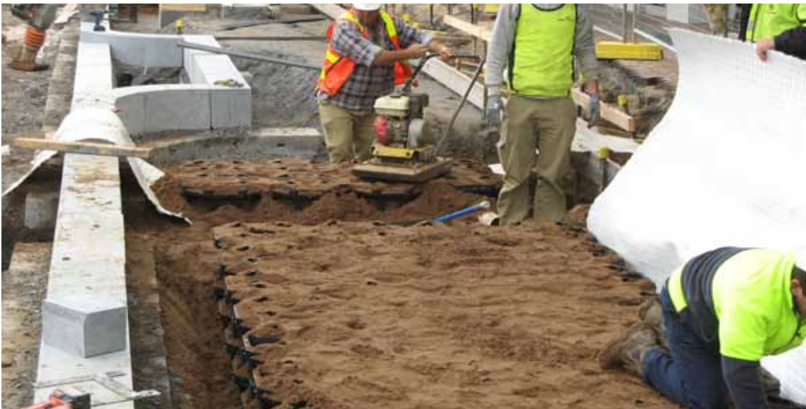
Continuous, linked soil trenches provide ultimate growth opportunities.
