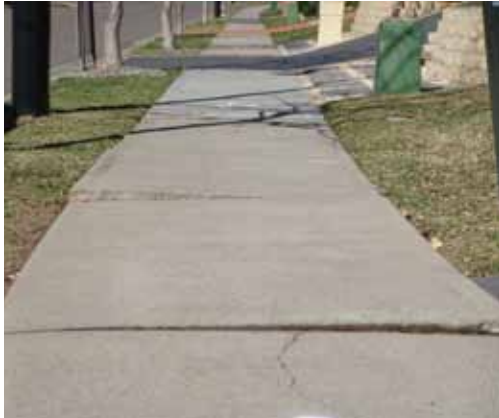
Fig 2.1.4 - Pavement damage caused by shallow rooting.
