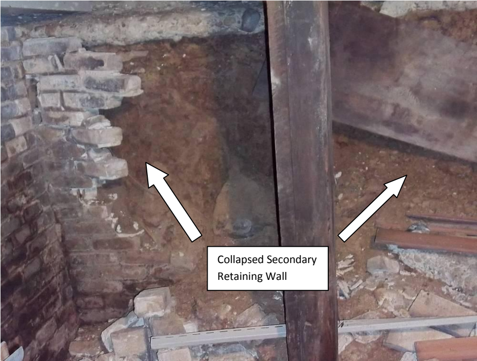
Figure 3 - Collapsed Secondary Retaining Wall along North End
