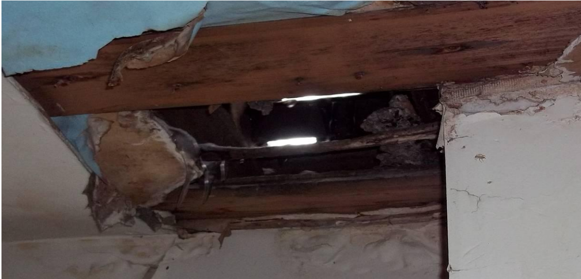
Figure 13 - Hole in the West Side of the Building
