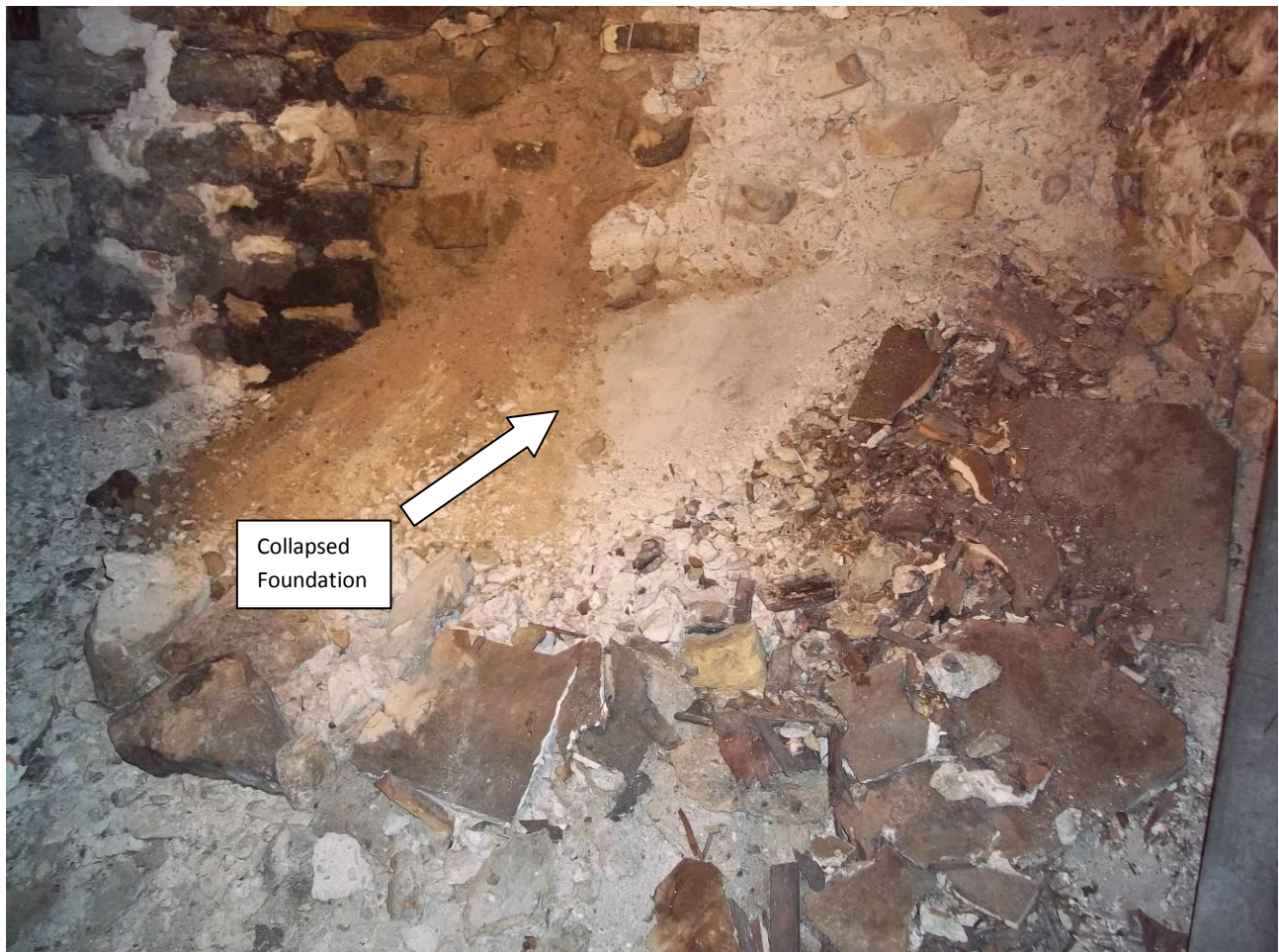
Figure 1 - Collapsed Foundation along East Wall
