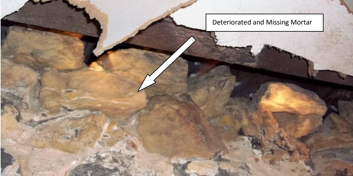
Figure 5 - Deteriorated and Missing Mortar
