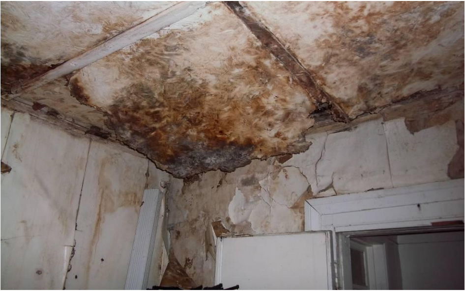
Figure 11 - Ceiling Collapse and Wall Damage on the Main Level
