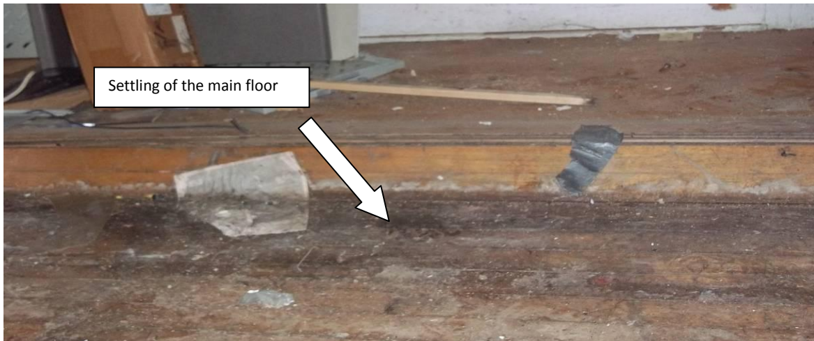
Figure 10 - Unevenness and Settling of the Flooring because of Inadequate Support
