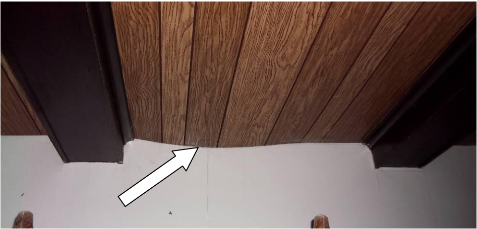
Figure 12 - Sagging In the Ceiling
