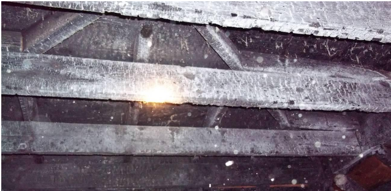
Figure 14 - Fire Damaged Trusses and Roof System
