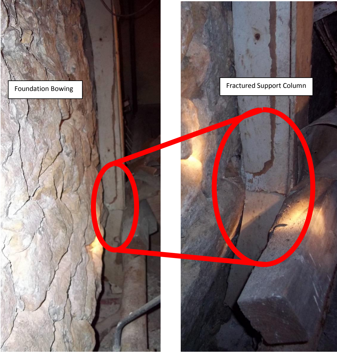
Figure 4 - East Foundation Wall Bowing Excessively and Fracture of a Wood Column
