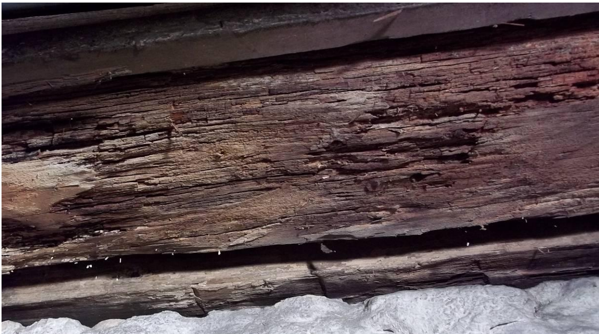
Figure 8 – Additional Example of Rotted Wood in Basement
