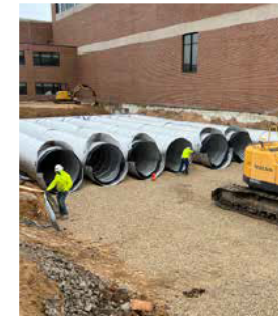
An underground stormwater detention system at West High in Madison.
