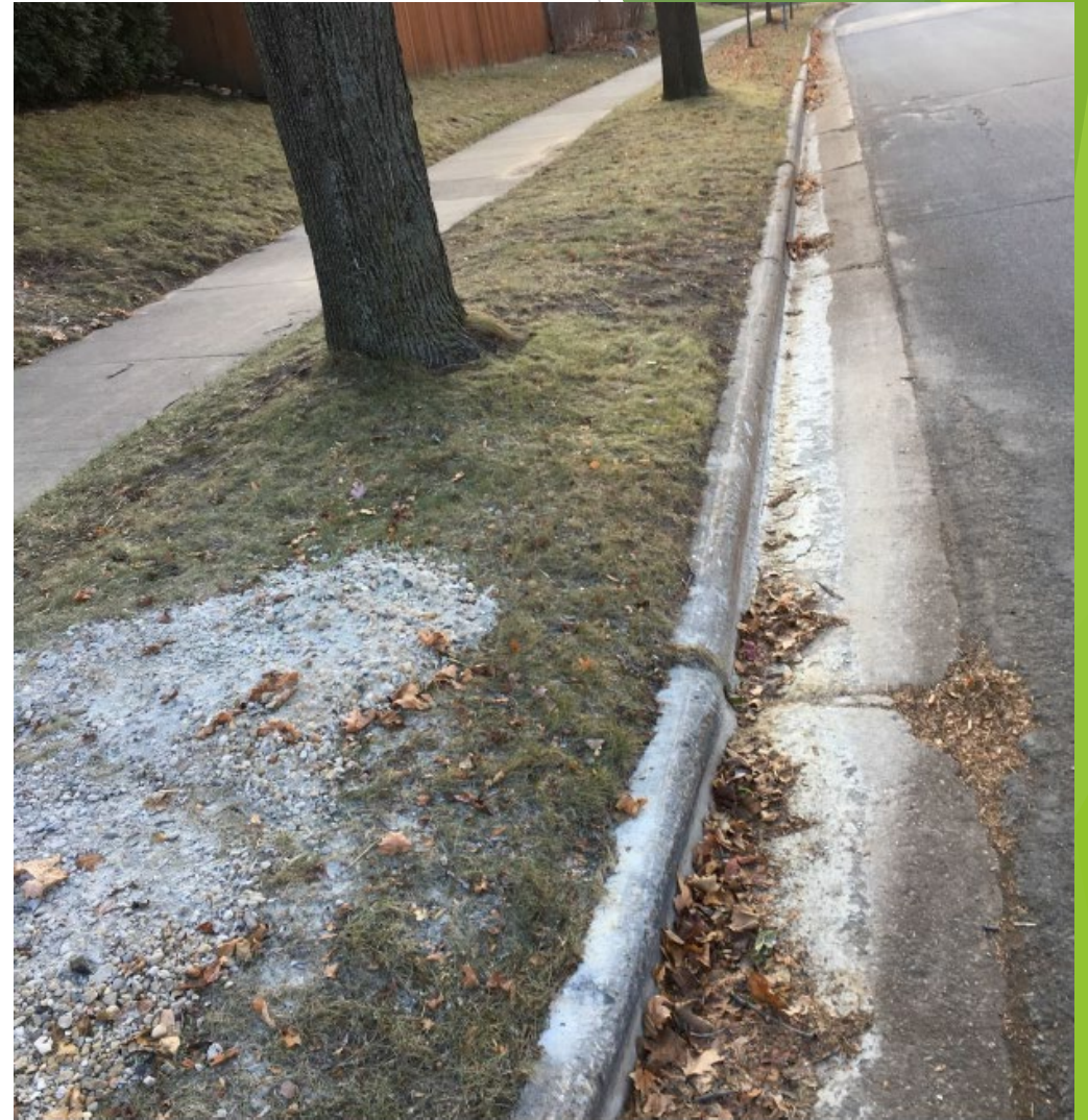
Concrete washout in curb
