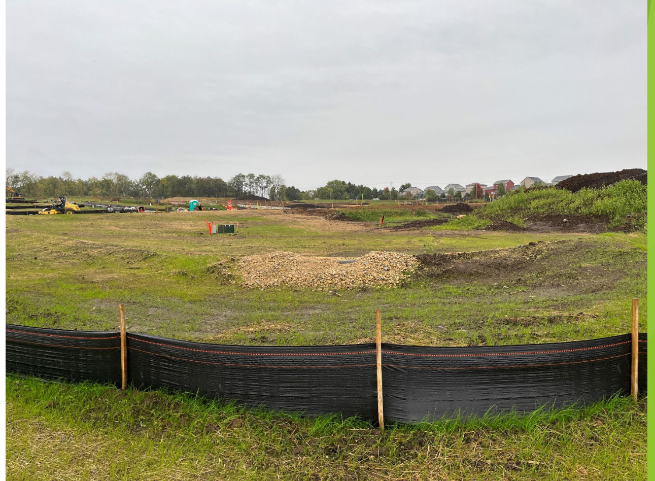
Acacia Ridge Erosion Control
