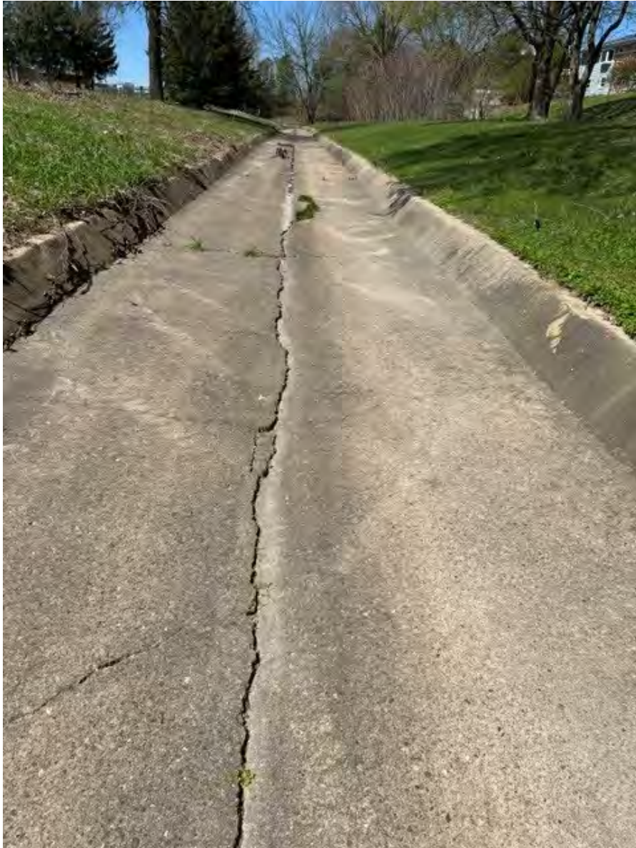
Typical West Section Crack to Repair
