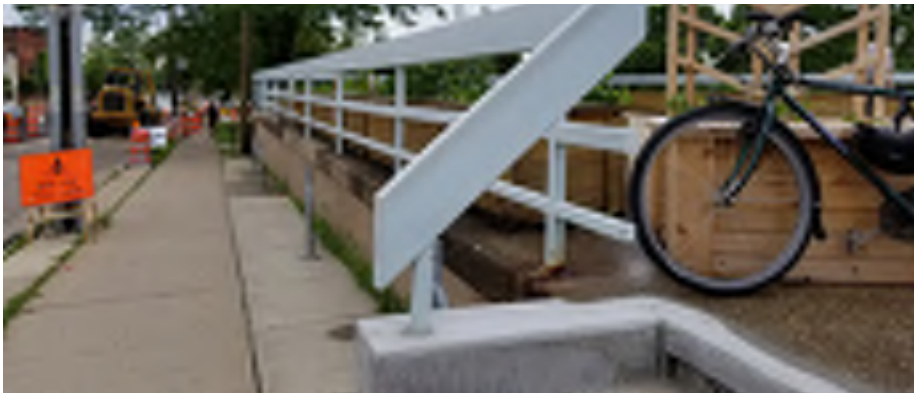
Figure B.16 MWU Water Reservoir Building Interfacing with East Wilson St Sidewalk
