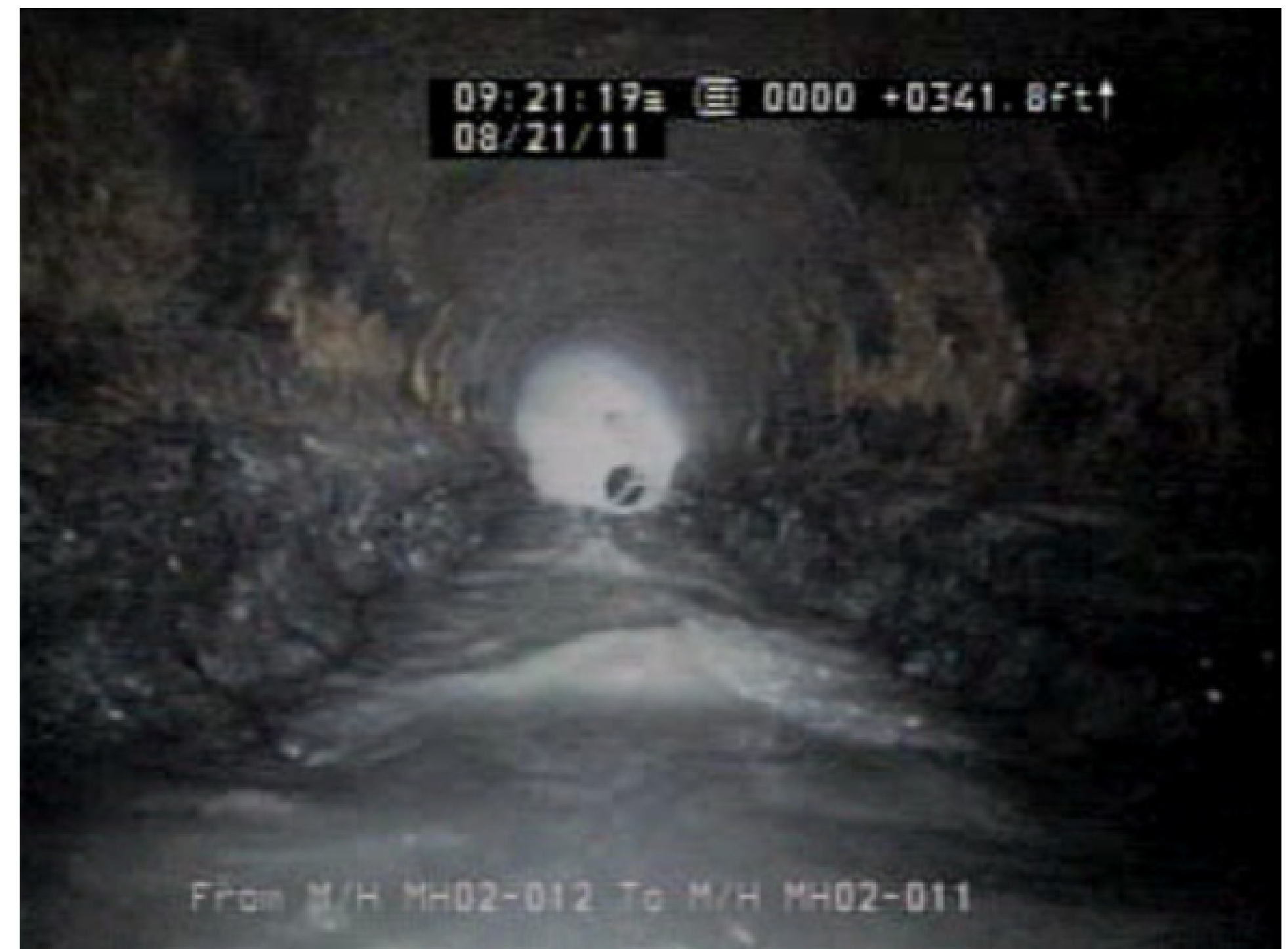
tuberculation (mineral desposits) inside the interceptor
