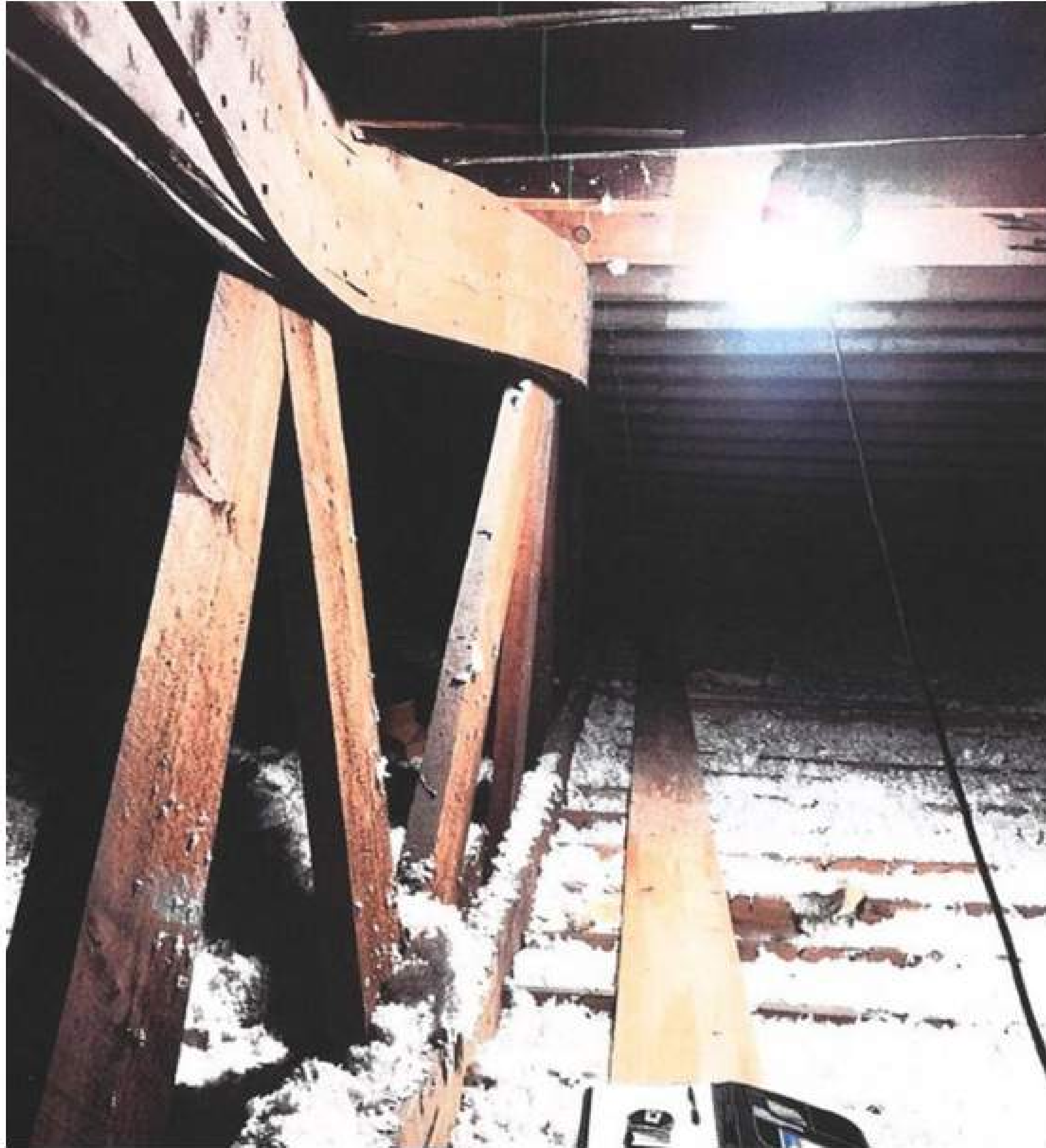
ROOF TRUSS FAILURE
