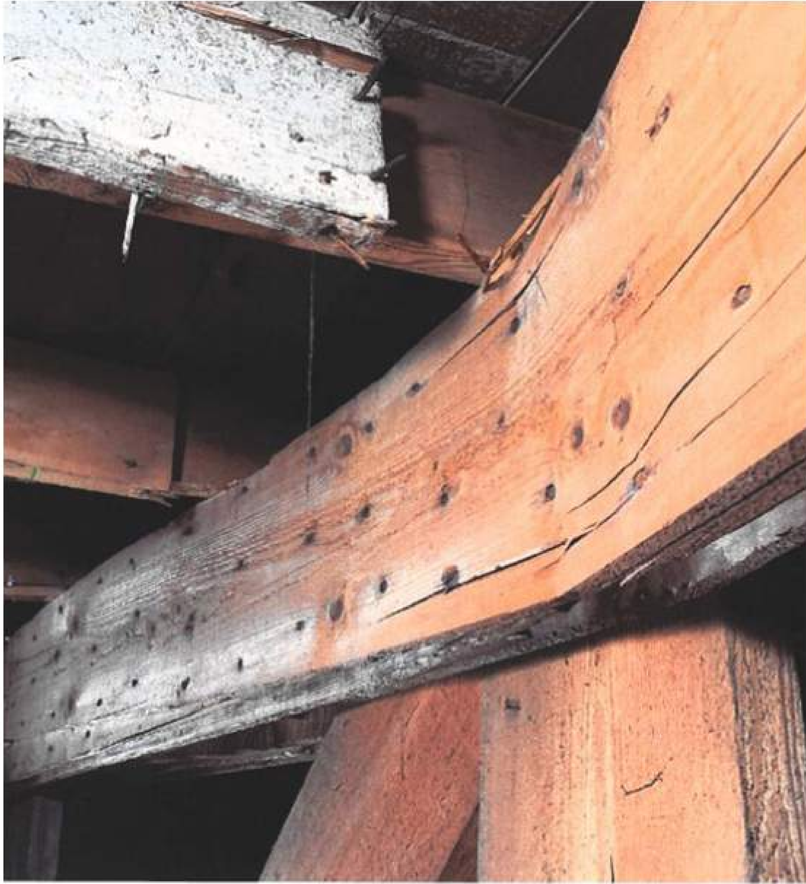
ROOF TRUSS & PURLIN FAILURE
