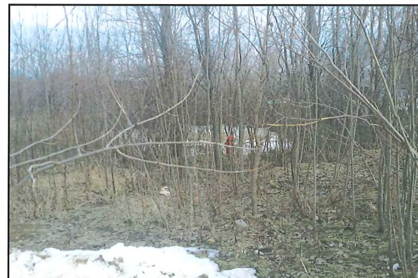
IMAGE 9: EXISTING FIRE HYDRANT
