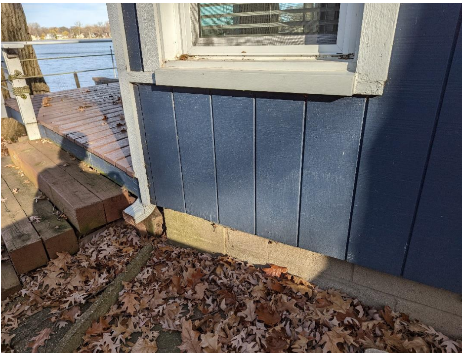
Foundation – The foundation of the building has significant settling and is contributing to floor canting and roof sagging. There is dampness at the crawl space.
