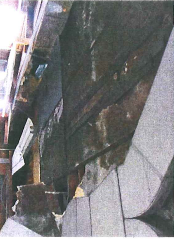
Existing Ceiling Condition
