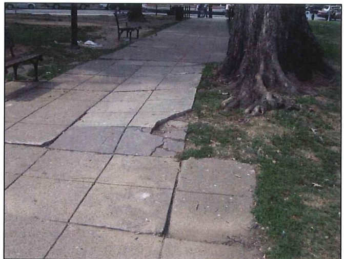
In compacted soil, tree roots often grow in the small void space just beneath the pavement, causing sidewalk heaving.
