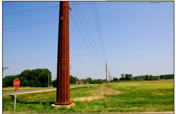
Overhead electric transmission lines along Reiner Road
