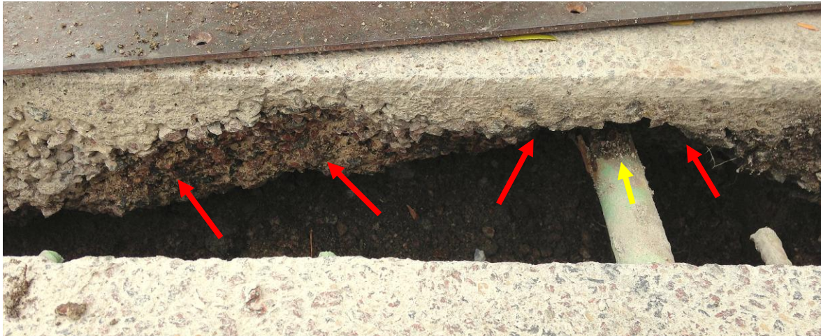
Figure 2. Oblique view of the slab showing deterioration of the slab bottom (red arrows) and corrosion of a dowel bar (yellow arrow).
