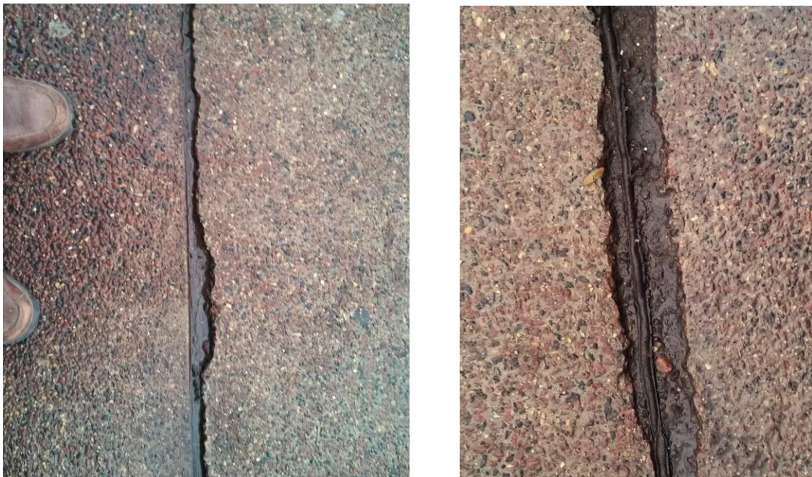
Figure 3. Cracking, spalling and raveling along joints
