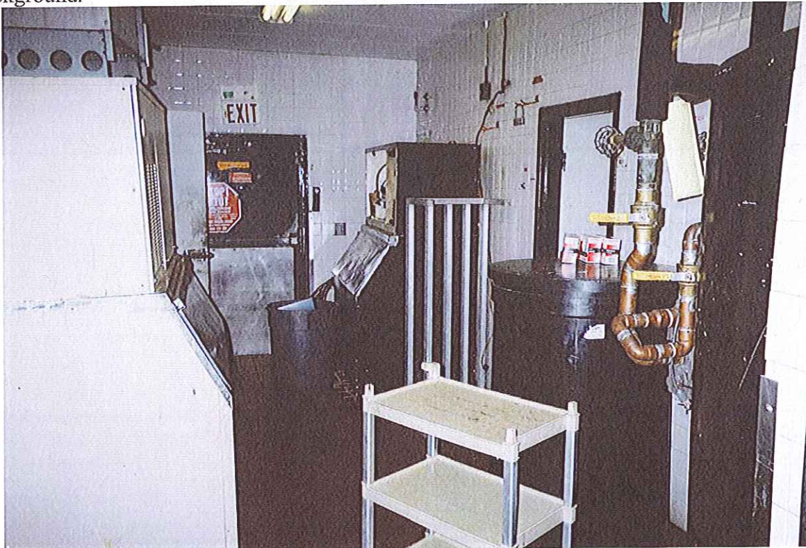
Figure 20 - Ice machines and water softener showing back door leading to dumpster storage area in the southwest corner of Chi Chi's Restaurant building. Door to utility room on right.
