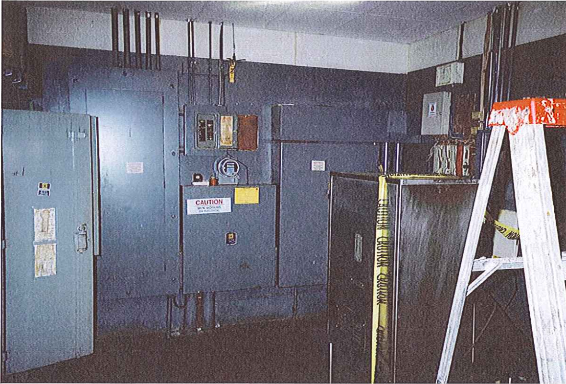
Figure 21 - Electric control panels in utility/storage room.
