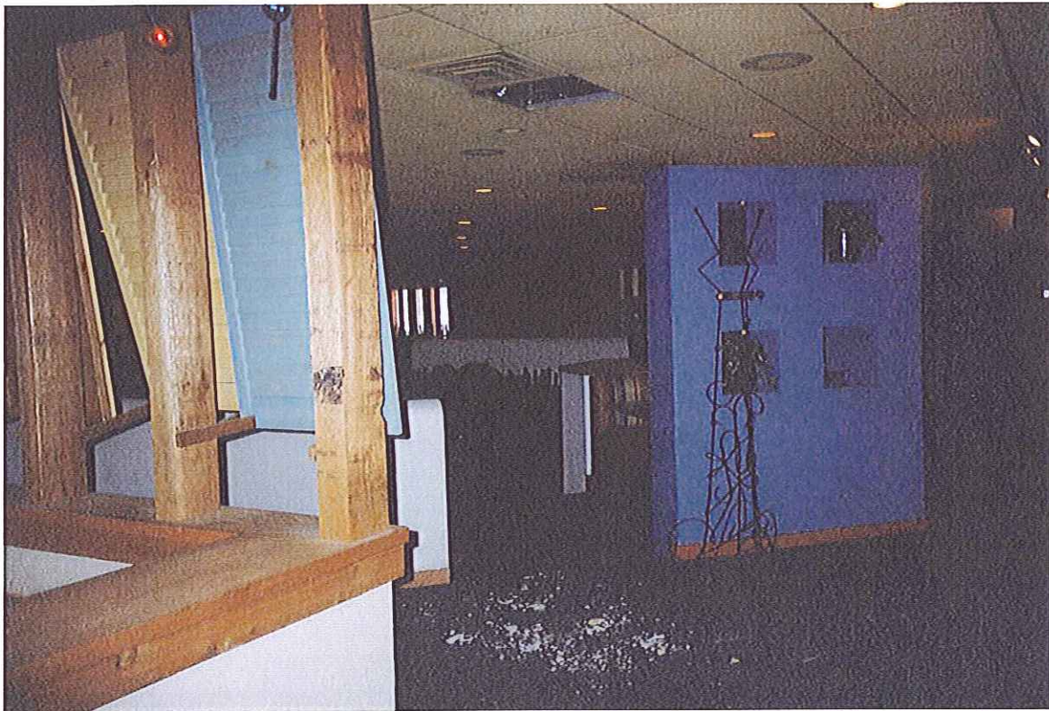
Figure 15 - Dining room area showing damaged ceiling tile on interior of the Chi Chi's Restaurant building.
