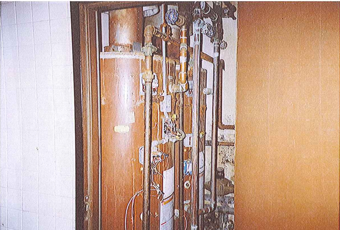
Figure 22 - Water heaters in small room adjacent to kitchen area.
