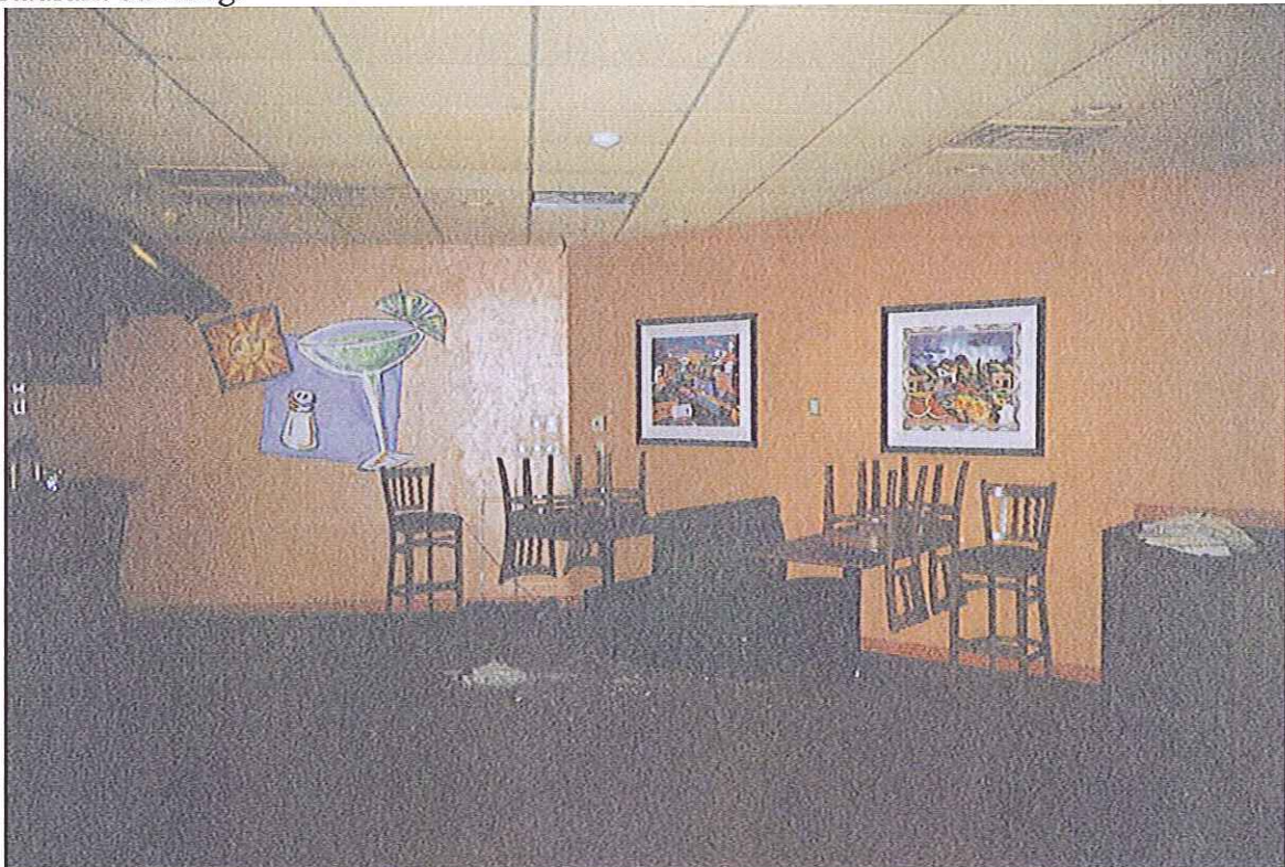
Figure 16 - Bar area showing damaged ceiling tile on interior of the Chi Chi's Restaurant building.
