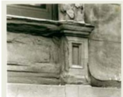
Window detail. Deteriorated brownstone before stucco repair.
