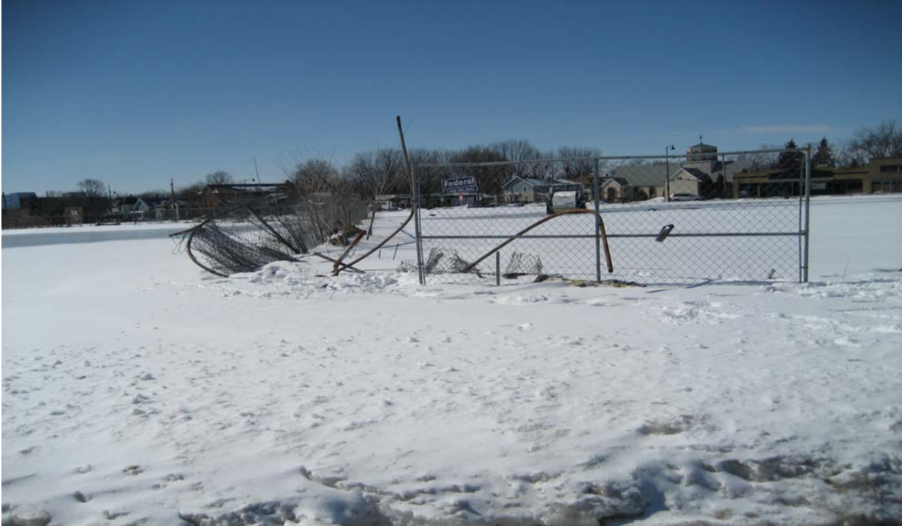
Leaning Fence March 4, 2008
