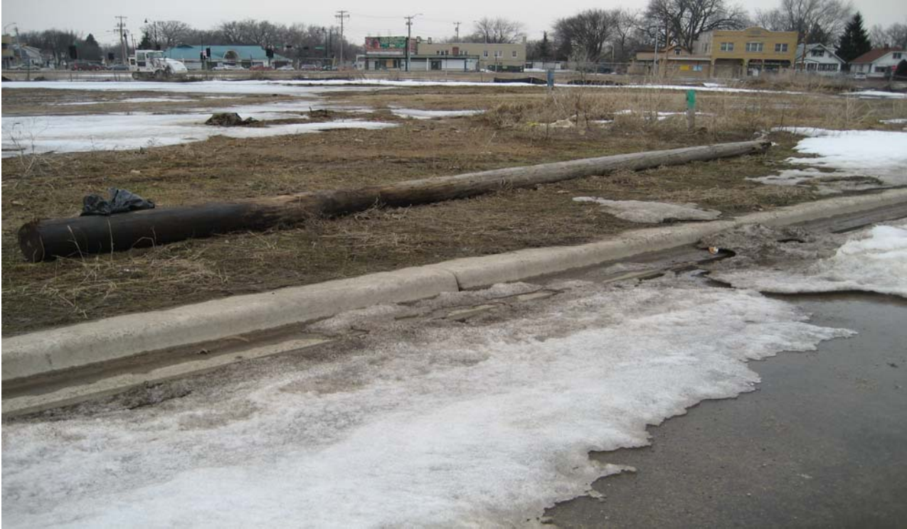
Downed & Abandoned Power Pole March 17, 2008
