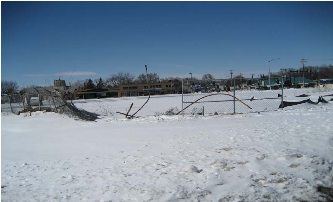
Broken Fence March 4, 2008
