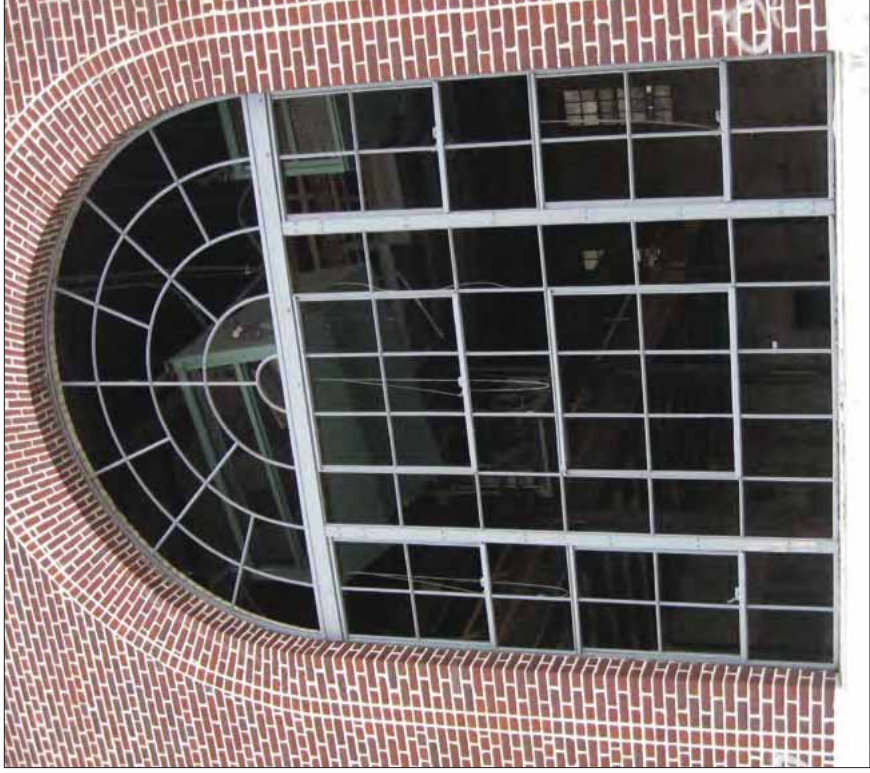
[12] This historic steel window has been cleaned, repaired, and primed in preparation for painting and reglazing.
