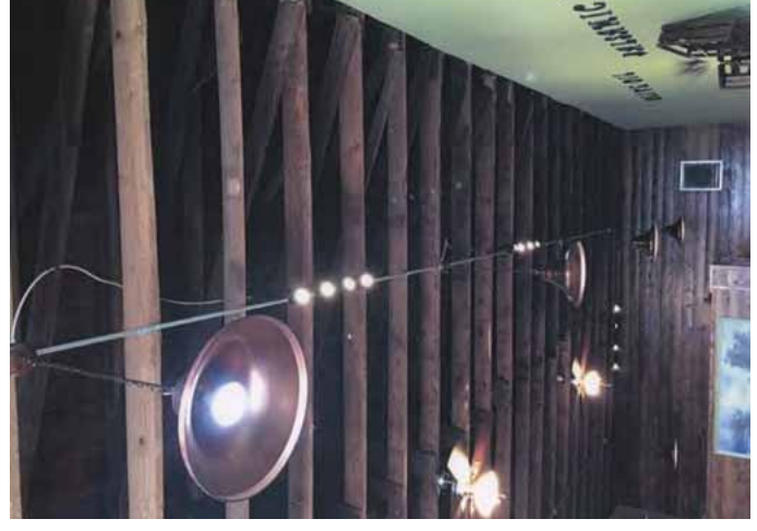
[40] Not Recommended: Removing a finished ceiling and leaving the structure exposed in a historic retail space does not meet the Standards for Rehabilitation.
