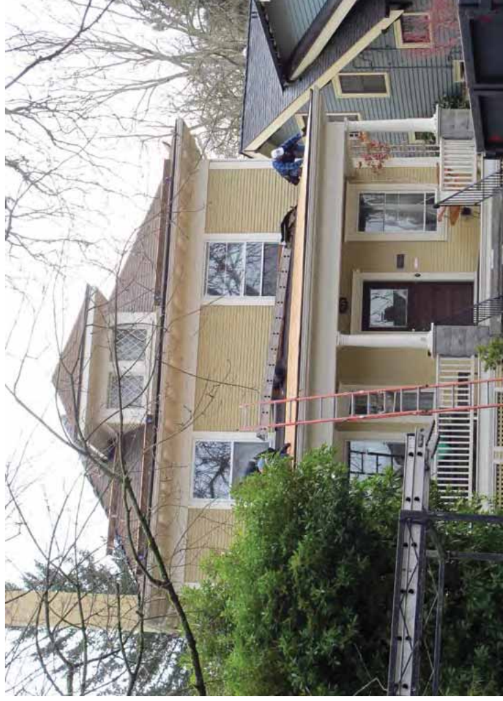
[16] The deteriorated asphalt shingles of this porch roof are being replaced in kind with matching shingles.
