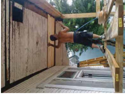
[24] Rotted boards in the beaded-board porch ceiling are being replaced with new matching beaded board.
