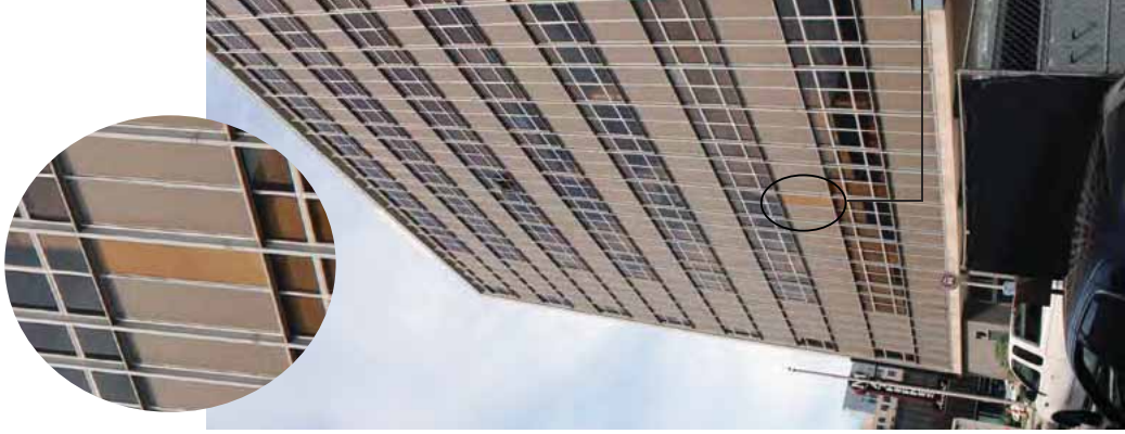
[16] Plywood provides temporary protection for an opening where a damaged spandrel panel was removed until a matching replacement panel can be installed.
