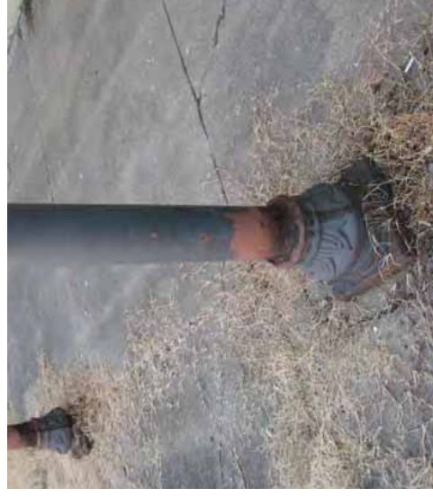
[7] (a) After the damaged portions of the base were repaired, (b) the cast-iron columns were cleaned and repainted to protect the metal from rusting.
