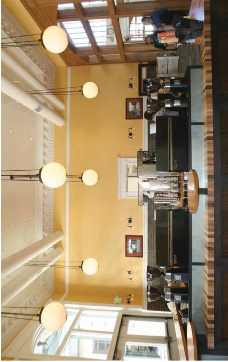
[37] Exposed and painted ducts were appropriately installed here in a retail space in Denver's historic Union Station after considering other options that would have impacted the ceiling height, or damaged or obscured the ornamental plaster crown molding. Photo: Heritage Consulting Group.
