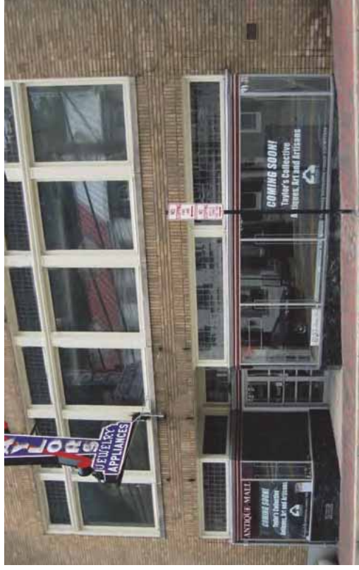
[15] Regular maintenance has helped to preserve this historic storefront, which retains all of its character-defining features, including the granite bulkhead, multi-paned transom glazing, and recessed entrance.
