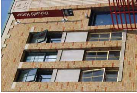
[21] The windows on the lower floor, which were too deteriorated to repair, were replaced with new steel windows matching the upper-floor historic windows that were retained.
