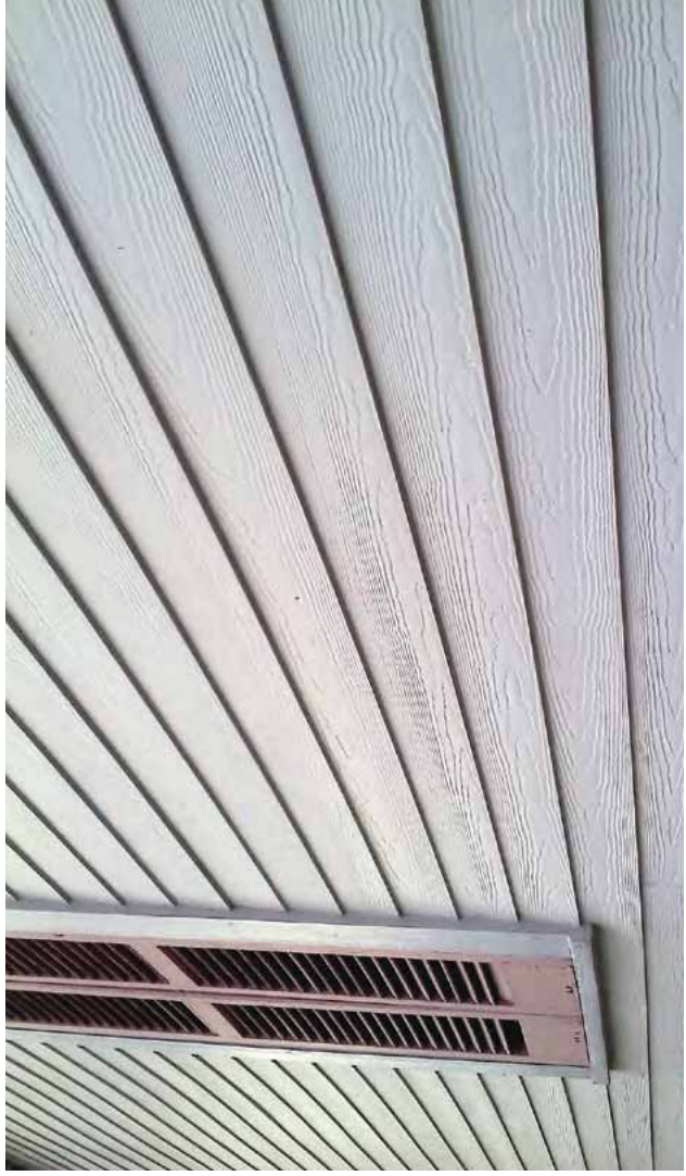
[10] Not Recommended: Cementitious siding with a raised wood-grain texture is not an appropriate material to replace historic wood siding, which has a smooth surface when painted.
