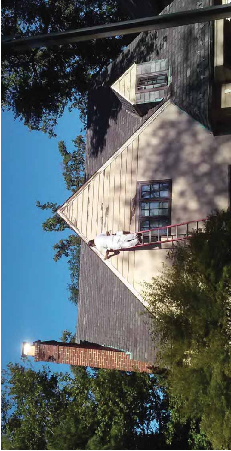
[4] Hand scraping to remove peeling paint from wood siding in preparation for repainting is an important part of regularly-scheduled maintenance.
