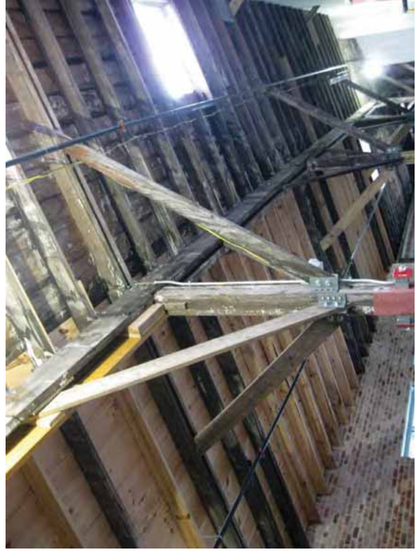
[17] New wood elements have been used selectively to replace rotted wood on the underside of the roof in this historic warehouse.
