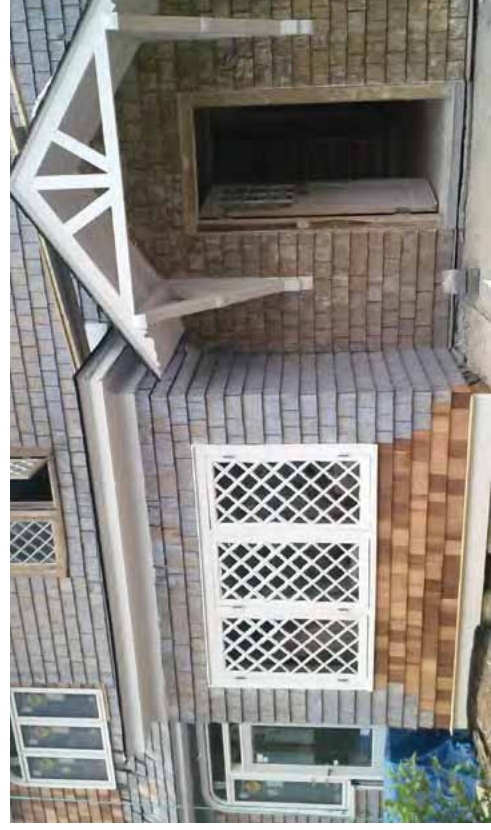
[5] Rotted wood shingles have been replaced in kind with matching wood shingles.
