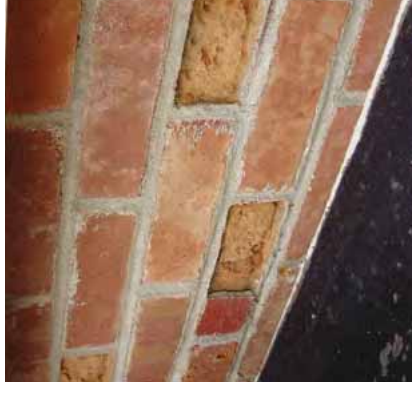
[2] Not Recommended: The use of inappropriate Portland cement mortar to repoint these soft 19th-century bricks has caused some of them to spall. Photo: Courtesy Nebraska State Historic Preservation Office.
