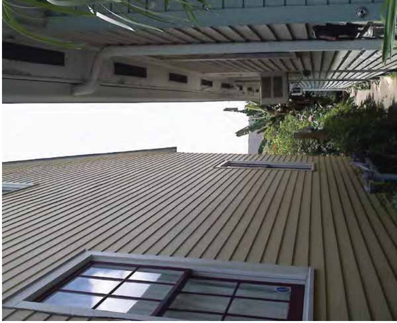
[9] Smooth-surfaced cementitious siding (left) may be used to replace deteriorated wood siding only on secondary elevations that have minimal visibility.
