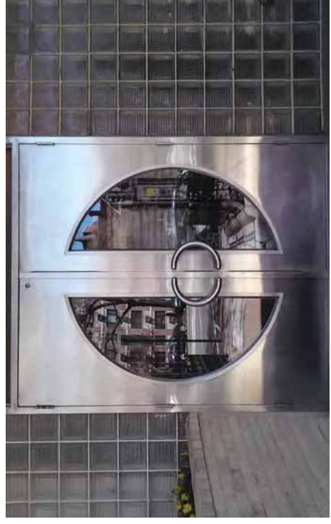
[11] The stainless steel doors at the entrance to this Art Deco apartment building are important in defining its historic character and should be retained in place.
