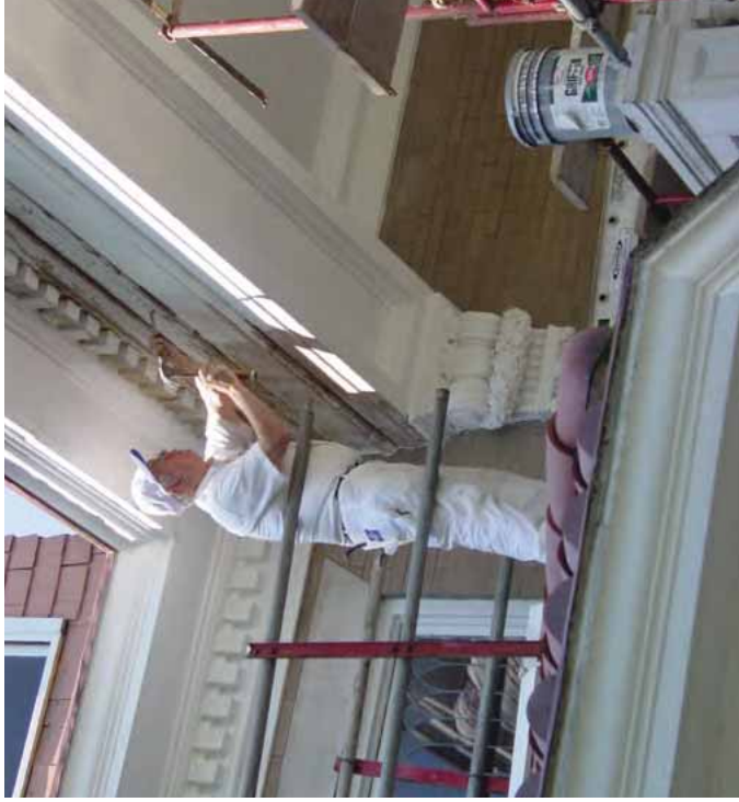
[12] Repair and limited replacement in kind to match deteriorated wood porch features is always a recommended preservation treatment.
