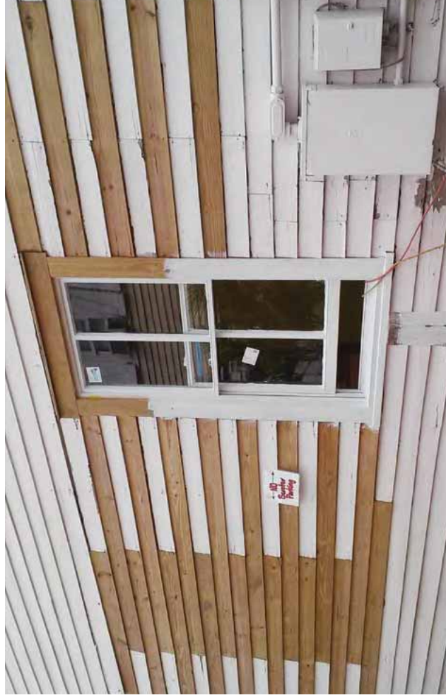
[8] Rotted clapboards have been replaced selectively with new wood siding to match the originals.
