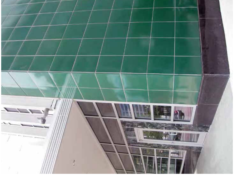
[15] New enameled-metal panels were replicated to replace the original panels, which were too deteriorated to repair, when the storefront of this early 1950s building was recreated.
