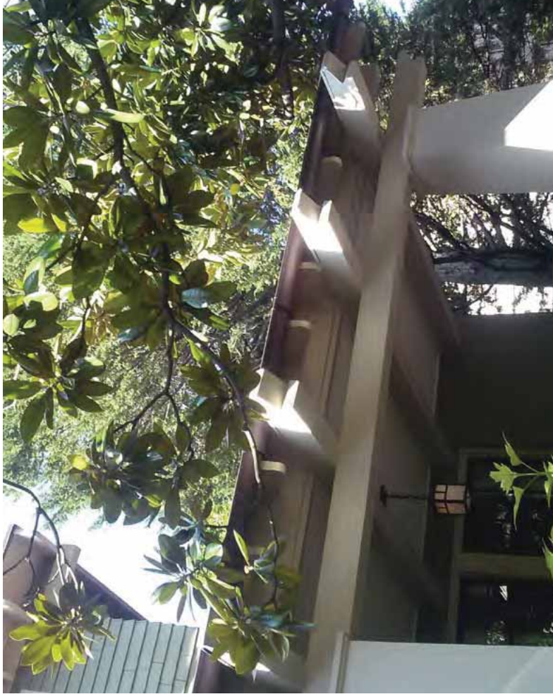
[13] It is important that exposed swallow tail porch rafters be kept painted to protect them from water damage.
