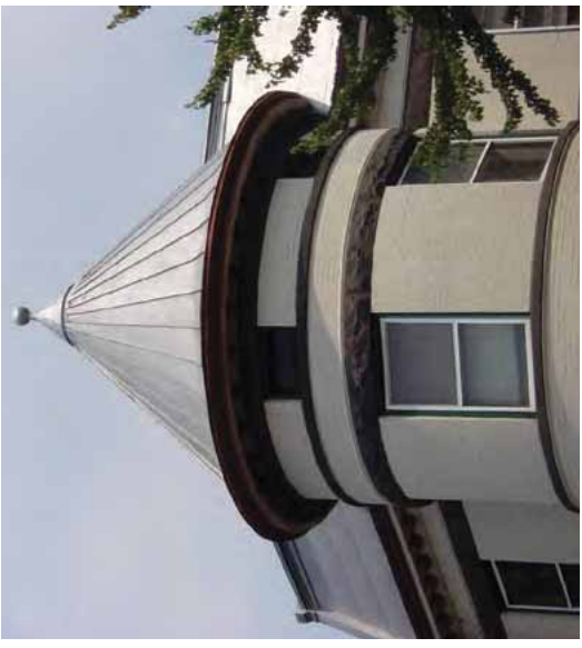
[6] A standing-seam sheet metal roof, like the one on the turret of this late 19 th century row house, must be kept painted to ensure its preservation.
