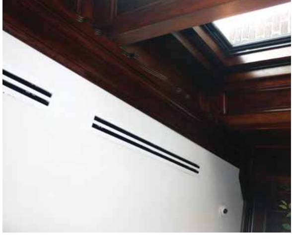
[34] The new ceiling ducts installed during the conversion of this historic office building into apartments are minimal in design and discretely placed above the windows.
