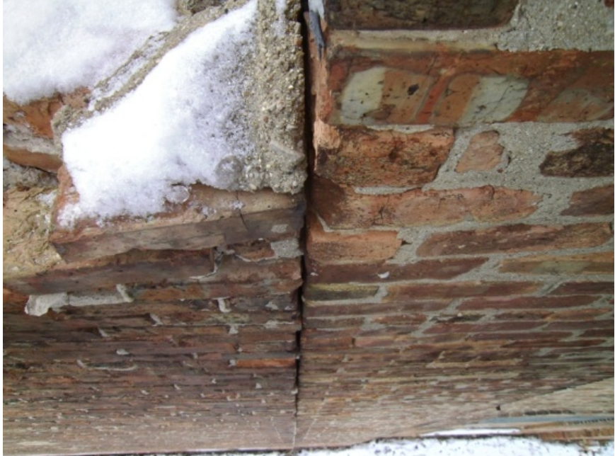
Image showing the joint on the north wall between Module D and Module E.
