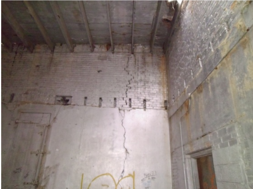
Image showing the vertical crack in the east wall at the southeast corner.
