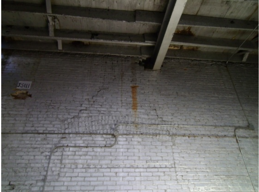
Image showing the crack at the beam to the foundation.
