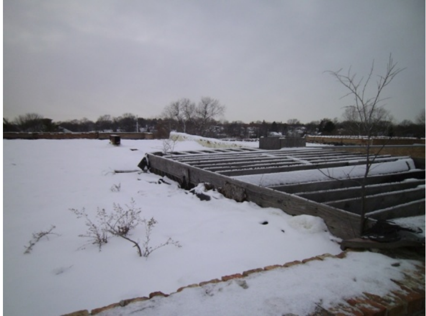
Image showing the topside of the roof. The north half of the roof appears to be partially framed with wood.
