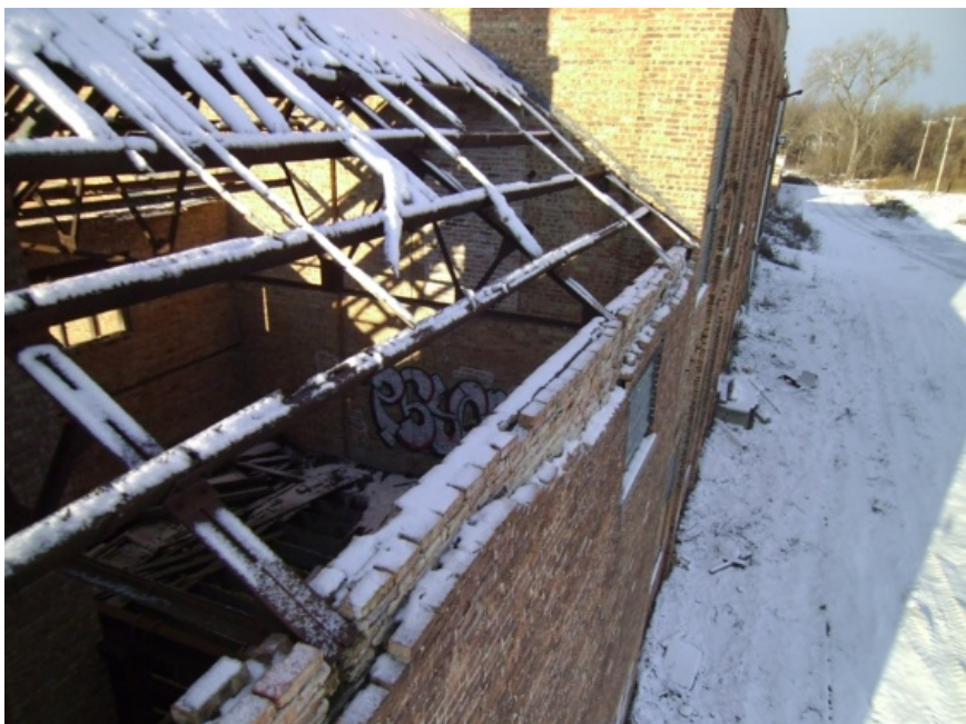
Image showing the top of the north wall. The deterioration appears to be slightly less significant than on the south wall.
