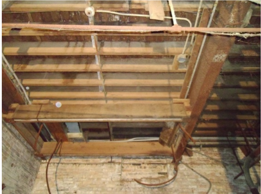
Image showing the floor construction of the second floor. The construction is similar at the third floor. Note the white mold on the floor decking near the top of the image. Other than some water staining, a significant quantity of the joists can likely be salvaged.
