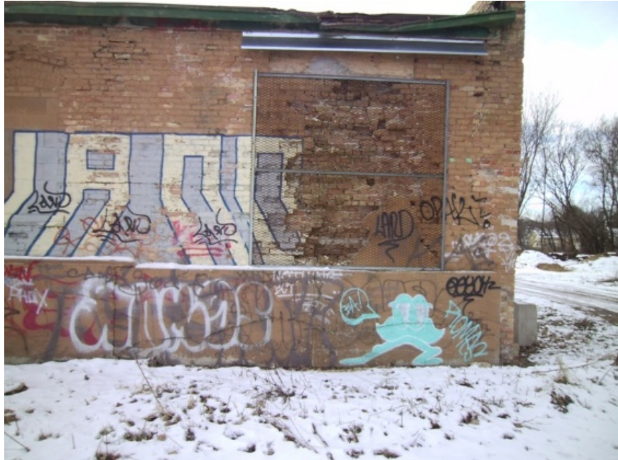
Image showing the region of wall exhibiting absent brick and eroded mortar.
