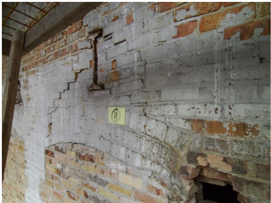
Images showing failed brick arches at a masonry walls, cracking at embedded steel beam ends and eroded masonry at an arched brick lintel.
