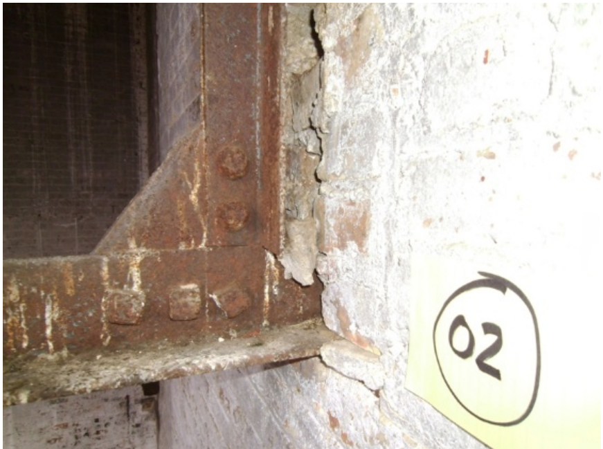
Image showing one of the truss (top) bearing locations. The bottom embedment into the wall appears to be a stabilization point. The rust appears to be only superficial.
