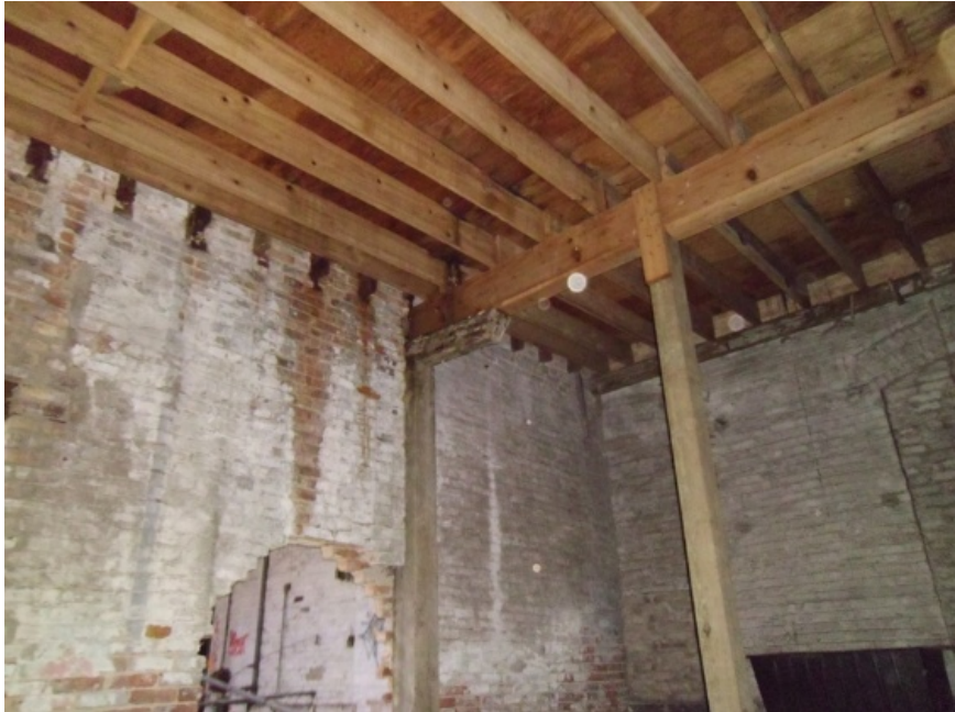
Image showing the framing at the west end. This framing is relatively new replacement framing for a section previously removed.
