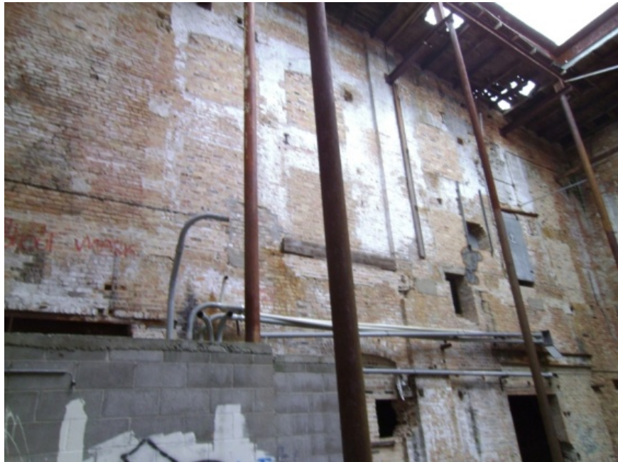
Image showing tall unstable columns to cobbled roof framing. Note the holes present in the wood sheathing.
