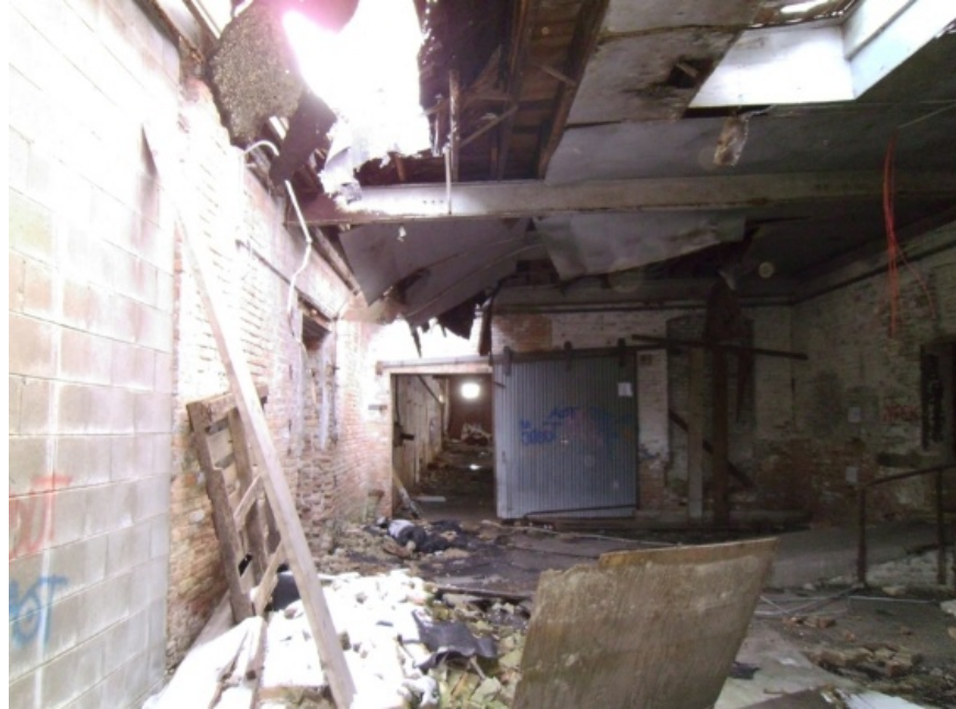
Image showing the damaged roof sections in the north end of the module. Substantial damage was noted in this region of the module.
