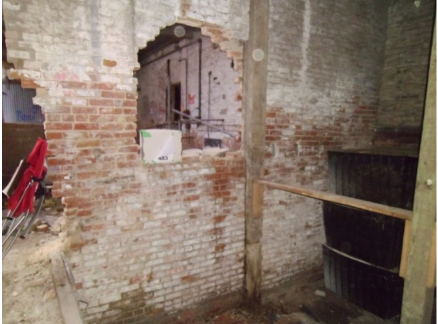
Image showing structural damage to the existing interior bearing wall.
