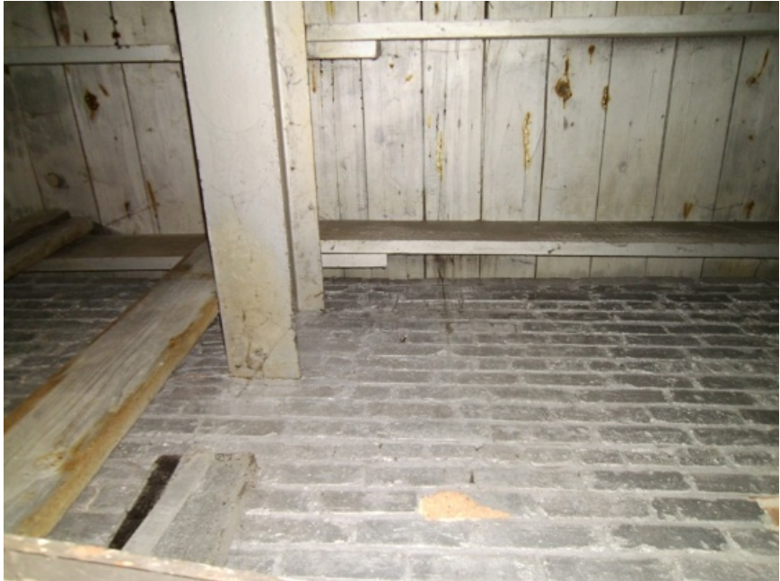
Image showing the lapped condition of joists and bearing of a steel beam in the masonry wall.
