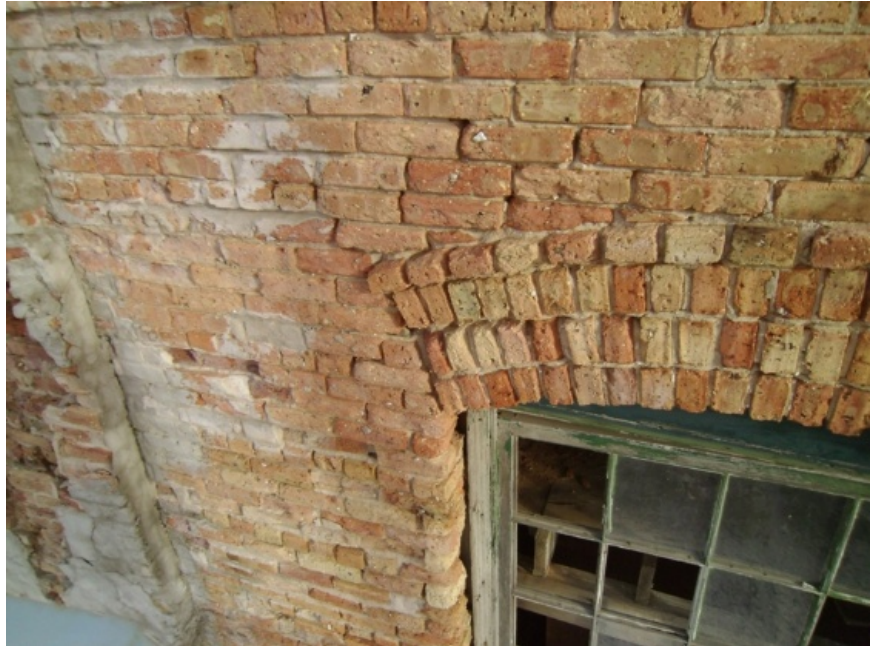
Image showing the water damage at the arched brick lintel.
