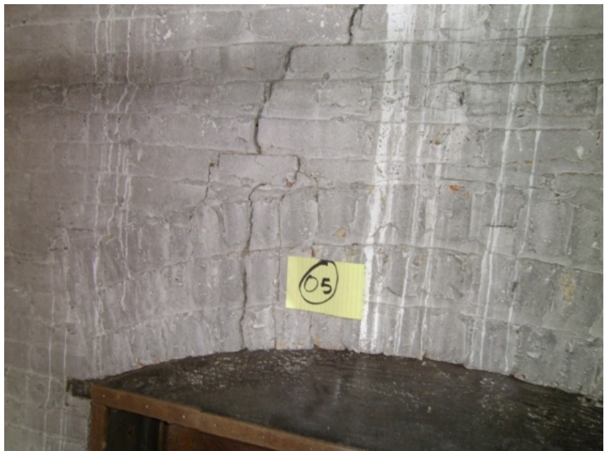
Images showing failed arched lintels of brick unit masonry, cracking at embedded steel, and brick and mortar erosion
