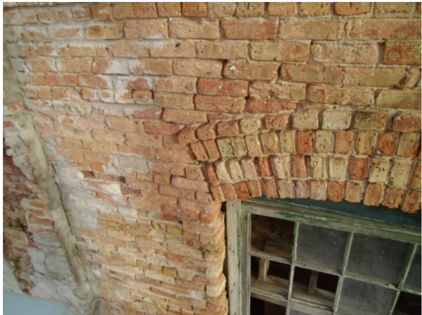
Image showing the mortar and brick erosion, exterior.
