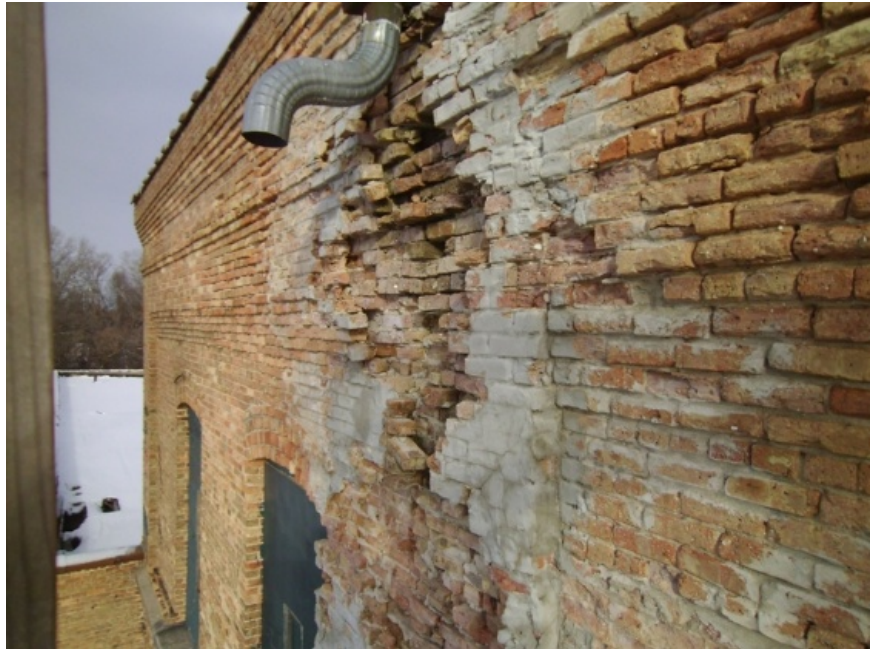
Image showing the upper section of brick deterioration from water infiltration.
