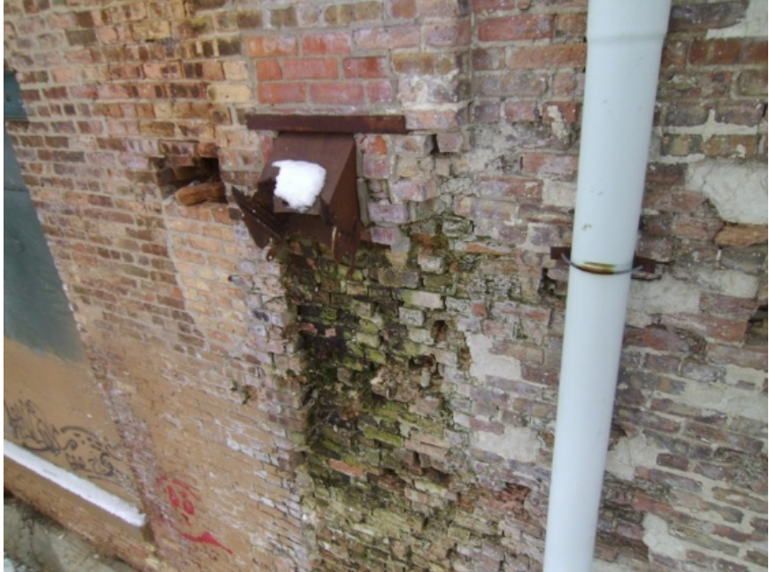
Image showing the exterior face of the north wall. This image was taken at the second floor level. A beam end behind this masonry is dislodged from its supporting masonry.
