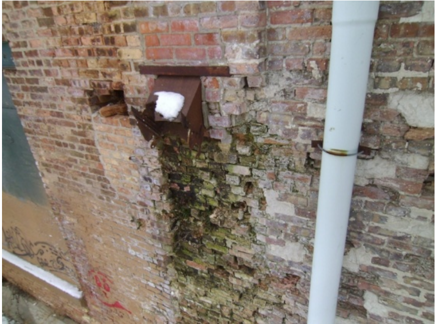
Image showing the exterior face of the north wall. This image was taken at the second floor level. The second floor beam end behind this masonry has dislodged from its supporting masonry.
