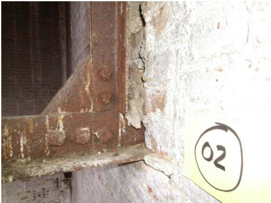
Image showing one truss (top) bearing. The bottom bearing embedment appears to be a stabilization point. The rust present appears to be superficial.
