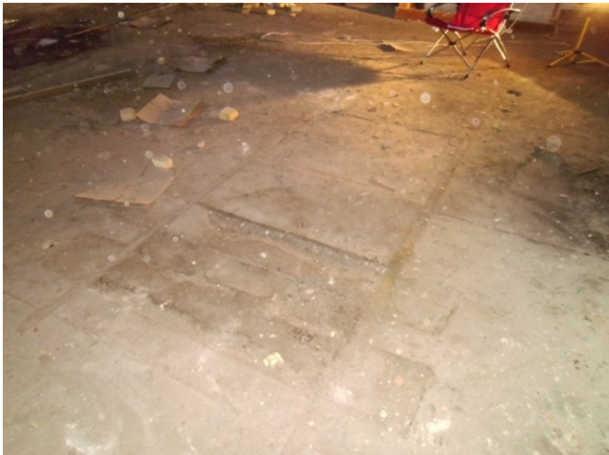
Image showing a suspected area of poorly placed concrete from the topside of the second floor.
