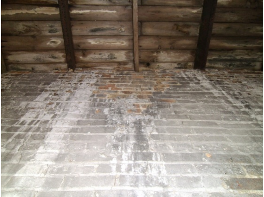
Image showing the damaged wood and steel framing bearing into the masonry walls.
