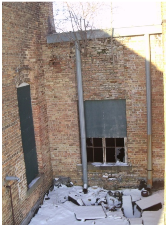
Image showing the exterior of the east wall in the region of the damage.
