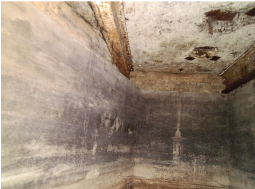
The space is a concrete confined pit with skewed walls. The space appears to have been covered in 1929 with steel beams and a reinforced concrete slab. The beams and slabs in this module appear to be in fair condition. Note the brickwork infill around the beams. The bottom of this pit is filled with stagnant water.
