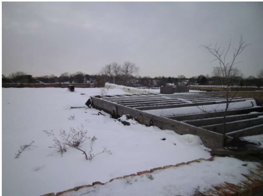
Image showing the topside of the roof at Module G. The north half of the roof appears to be partially framed with wood.
