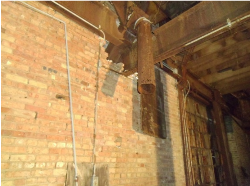
Image showing the dislodged beam end at the damaged masonry.
