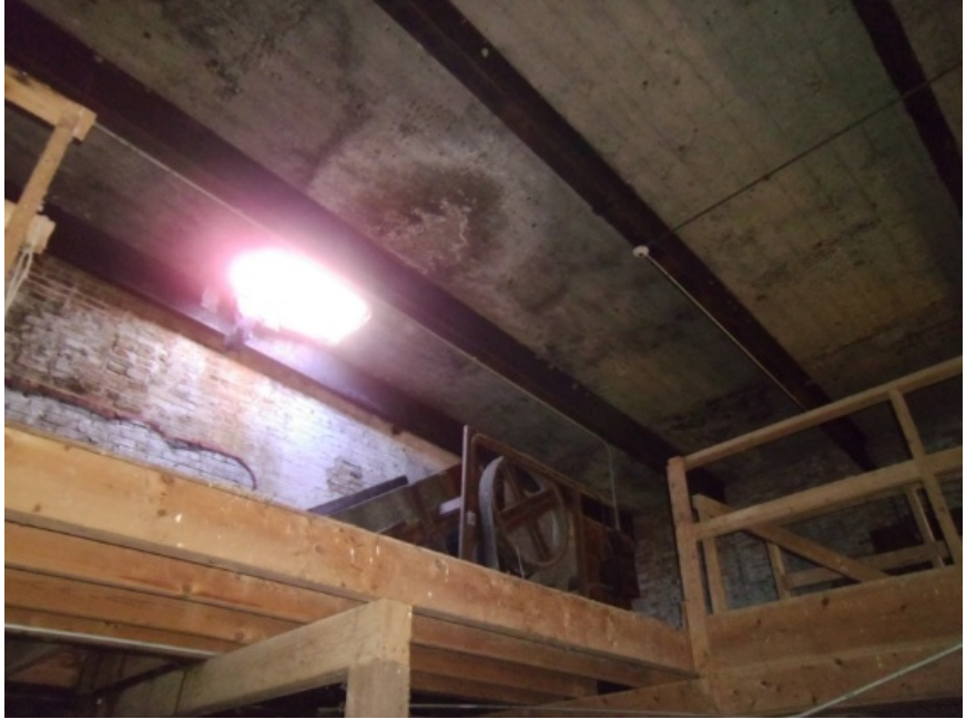
Image showing the damaged roof slab at the east end.
