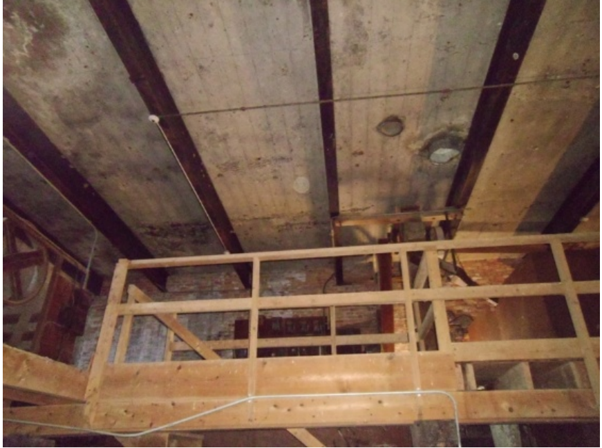
Image showing the wire mesh-reinforced concrete slab over steel beam roof structure.
