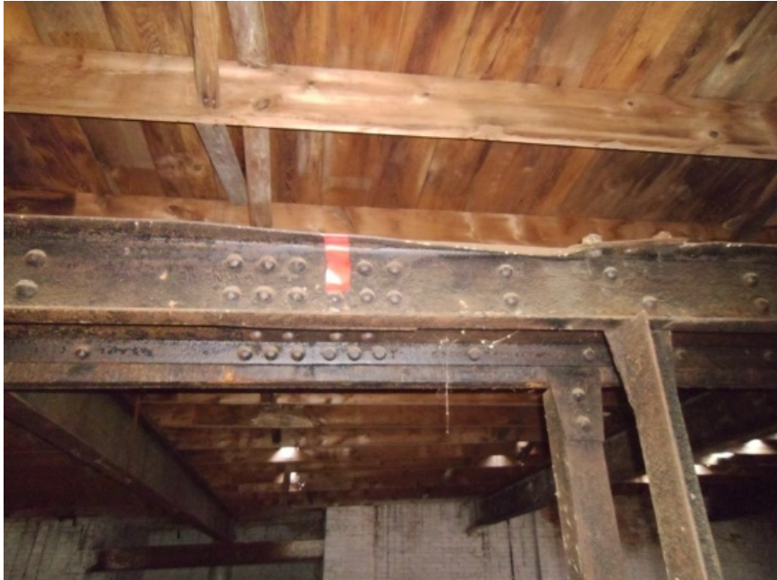
Image of a top chord that has been damaged by falling objects.
