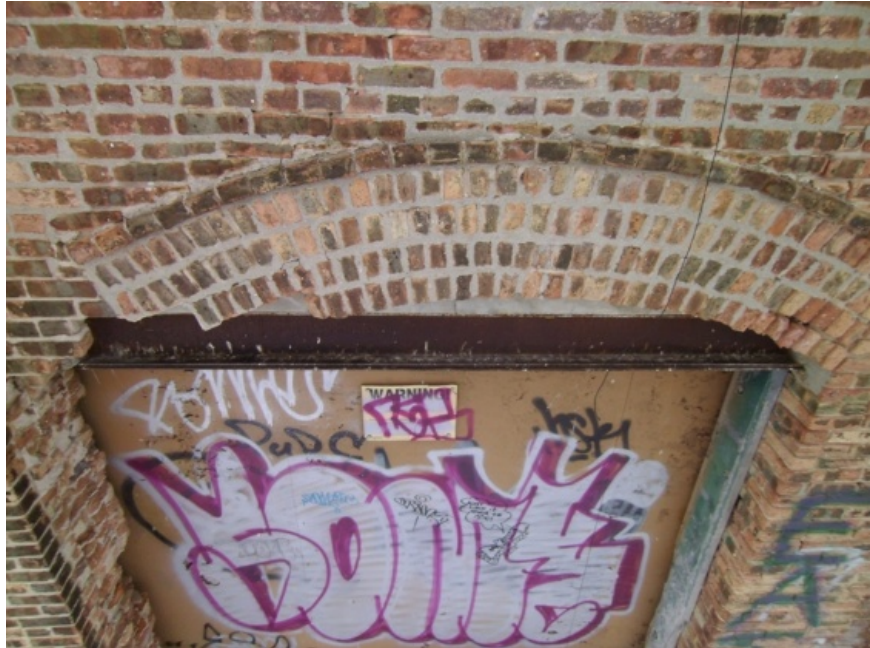
Image showing the poorly constructed lintel at the north wall. The steel supporting the masonry only supports a portion of the wall width. The bearing shown at the left is damaged.
