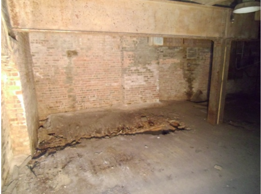
Image showing an area of the first floor collapse.
