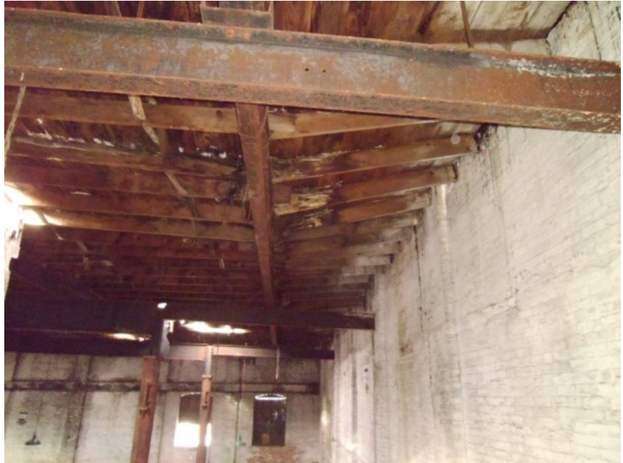
Image showing deterioration in the wood roof framing.
