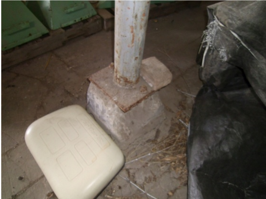
Image showing the column support at a damaged concrete pier. A portion of the bearing plate is unsupported.
