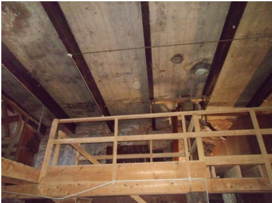
Image showing the minor openings in the roof.
