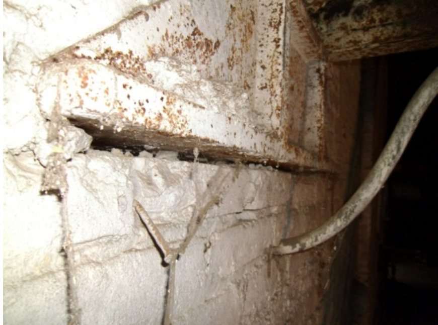
Image showing the gap between the masonry wall and the truss bearing casting.
