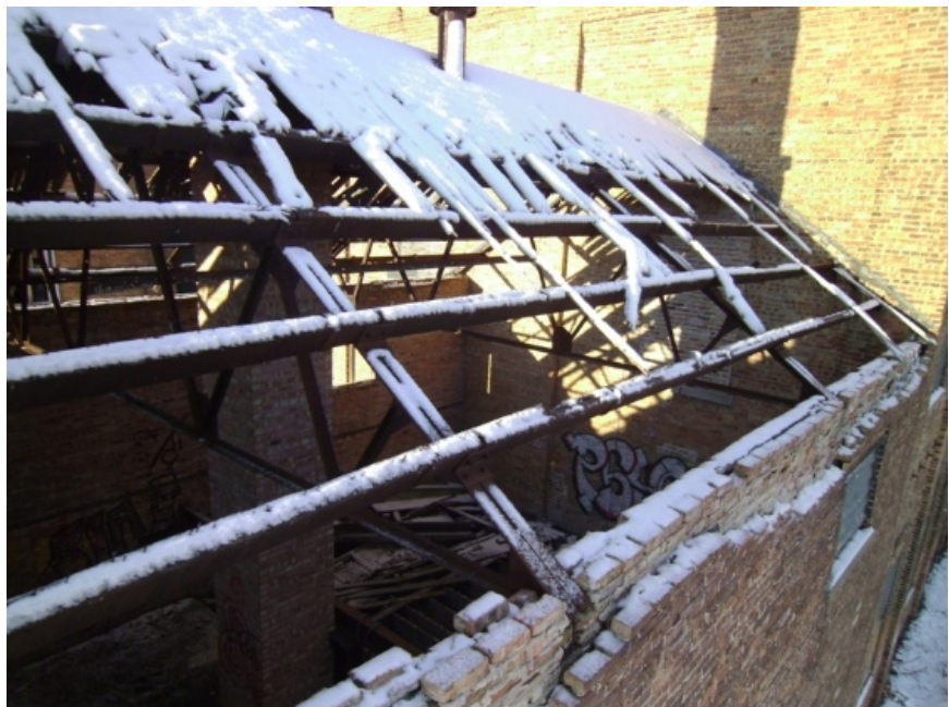
Image showing the deteriorated wood sheathing over the blocking nested in the channel purlins, and the fabricated trusses below. The truss bearing ends can be seen exposed in the damaged masonry.
