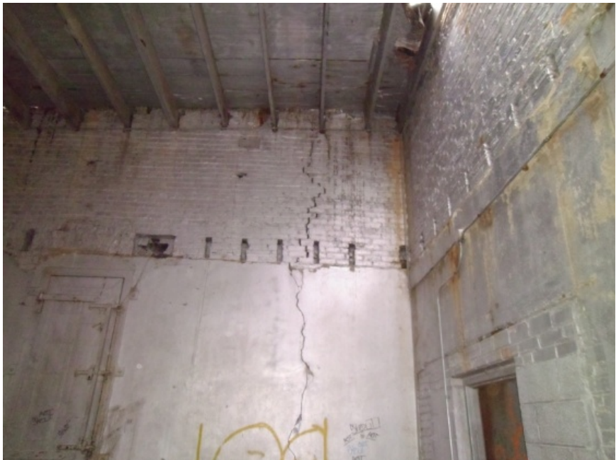
Image showing the vertical crack in the east wall at the southeast corner.
