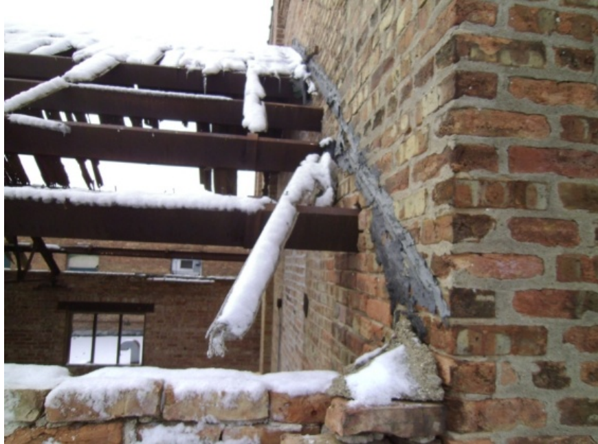
Image showing the bearing ends of Module D's steel channels into the wall of Module E
