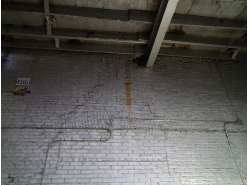
Image showing a through wall crack at a south wall beam.
