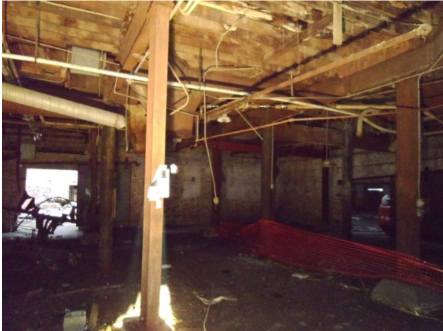
Image showing the column, beam and joist framing of Module F. Note white mold-covered joists present near the top of the image.
