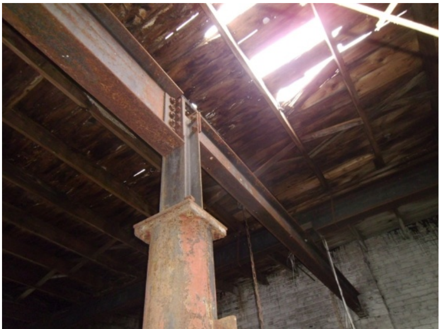
Image showing the original 1905 columns of the buildings being adapted to support the 1929 roof beams.
