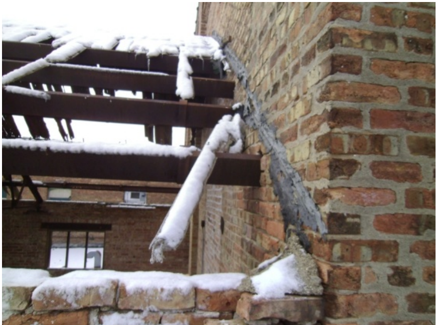
Image showing the bearing ends of the steel channels into the wall of Module E.
