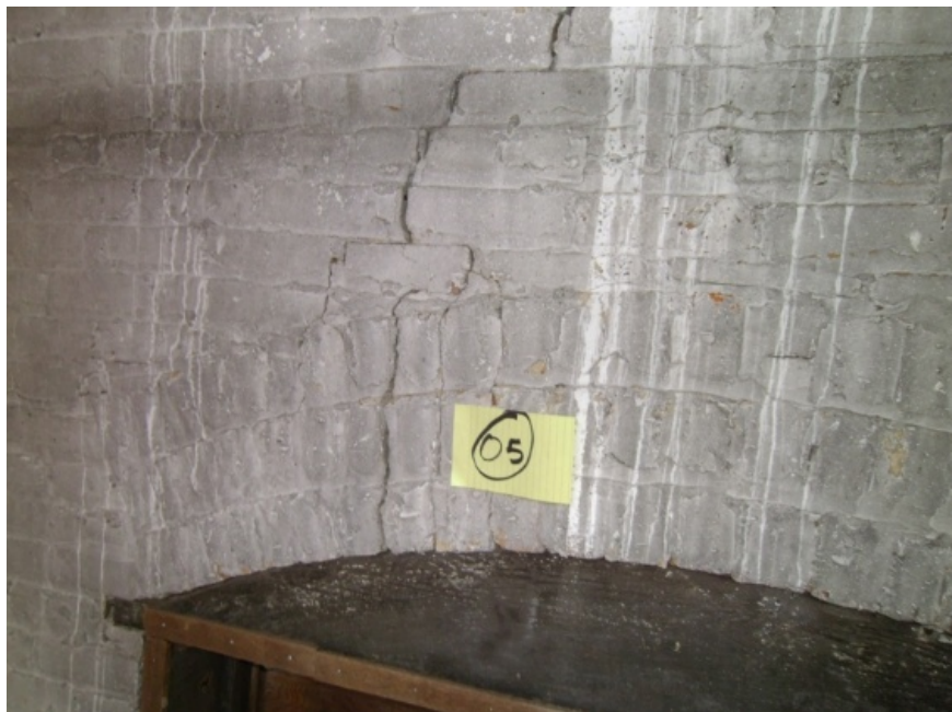
Images showing failed brick arches at a masonry walls, cracking at embedded steel beam ends and eroded masonry at an arched brick lintel.
