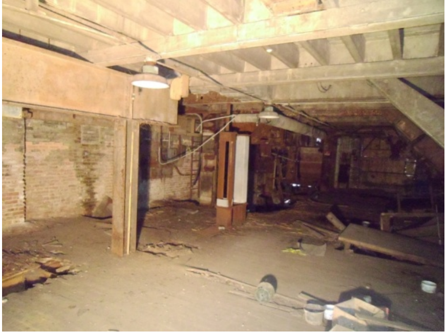
Image showing another region of Module G. This floor system is wood joist covered with a concrete slab.
