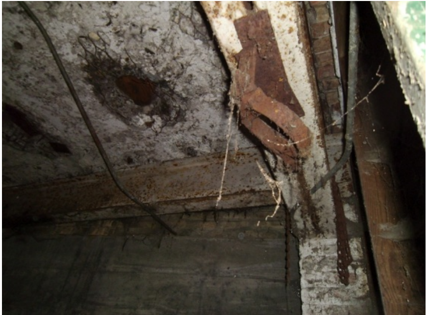
Images showing the construction of first floor. The rusted loop is an old mechanical hanger. The structural slab can be seen as well as a support beam at the left side of the image. Above the hanger loop is the lintel supporting the brickwork above.
