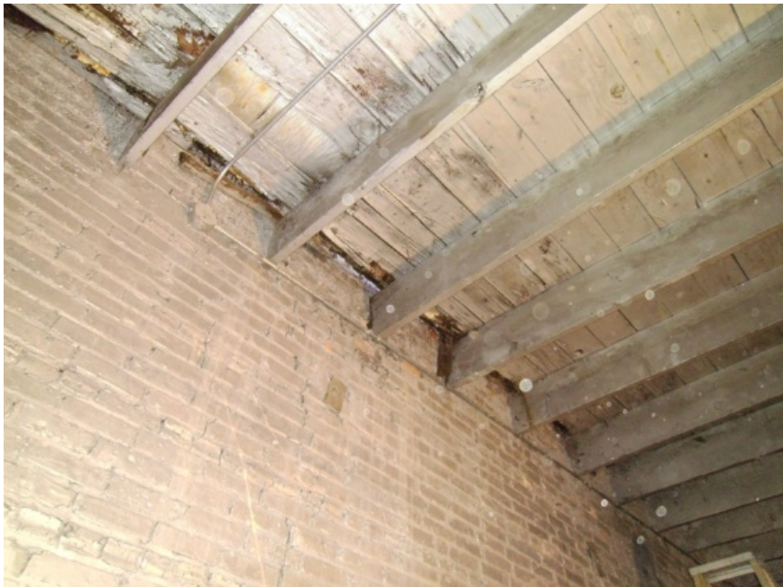
Image showing damaged roof decking along the west wall. The decking directly in contact with the wall is deteriorated. Adjacent discolored regions in the decking show the deterioration for a significant distance away from the wall. Many of the joist ends bearing in the wall have decay damage. The concealed topside surface of the decking will likely reveal significantly more damage that what can be seen in images.
