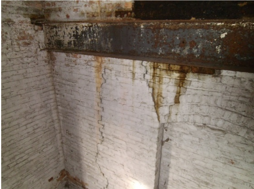
Image showing the large cracks in the walls at the southwest corner of Module A.
