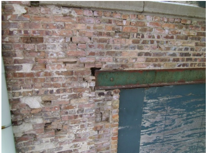
Image showing how deterioration and erosion in the masonry joints have undermined the integrity of a lintel bearing.
