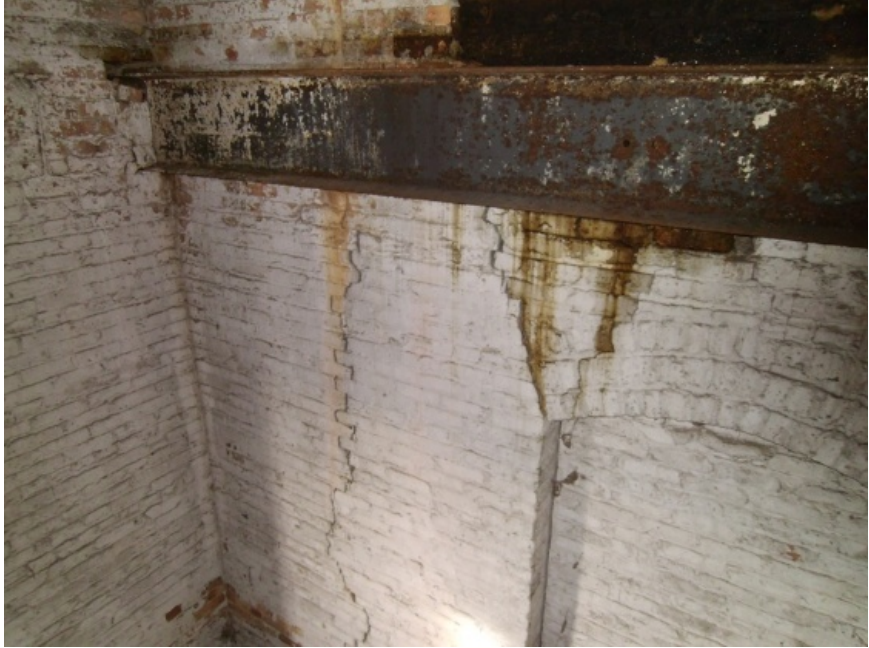
Image showing the large cracks in the walls at the southwest corner A. The steel channel will be left in place.
