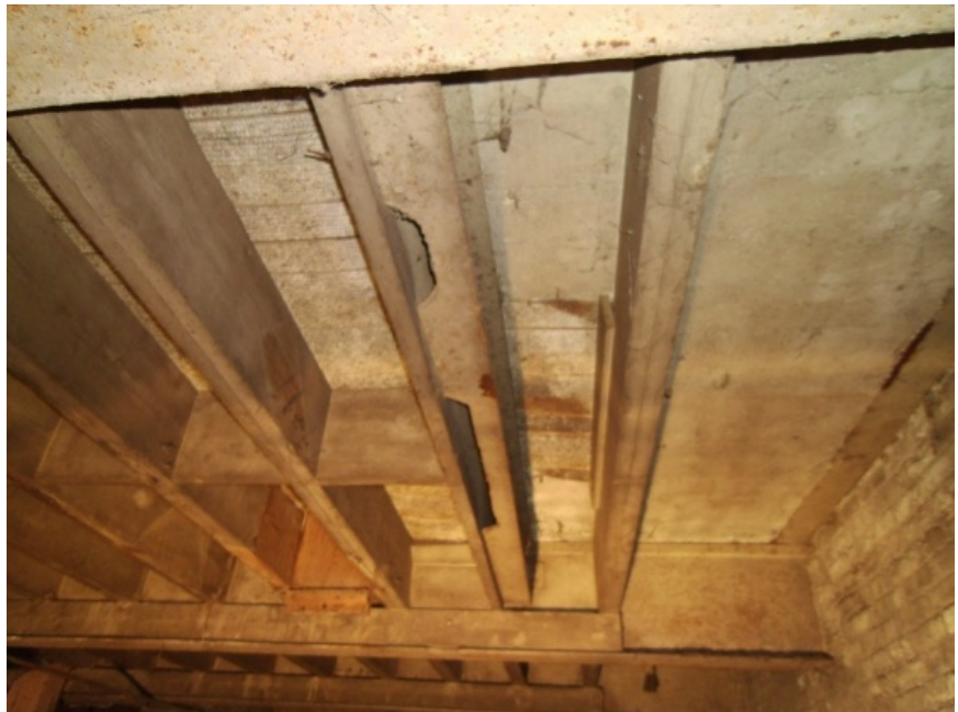
Images showing a transition from wood joist supporting concrete to reinforced concrete along the walls. The protective cover on the reinforcing mesh has fallen away in some areas exposing the mesh.
