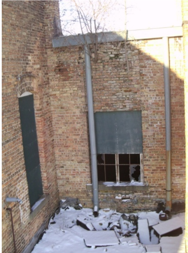
Image showing the nonfunctional downspout at the northeast wall at Module A. Note the vegetation at the wall.
