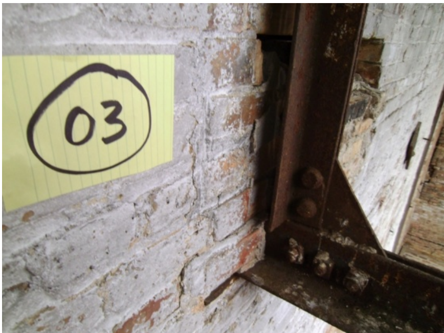
Image showing a truss bearing at the south wall. Note the cracks in the masonry suggesting that the truss is dislodged from the masonry.
