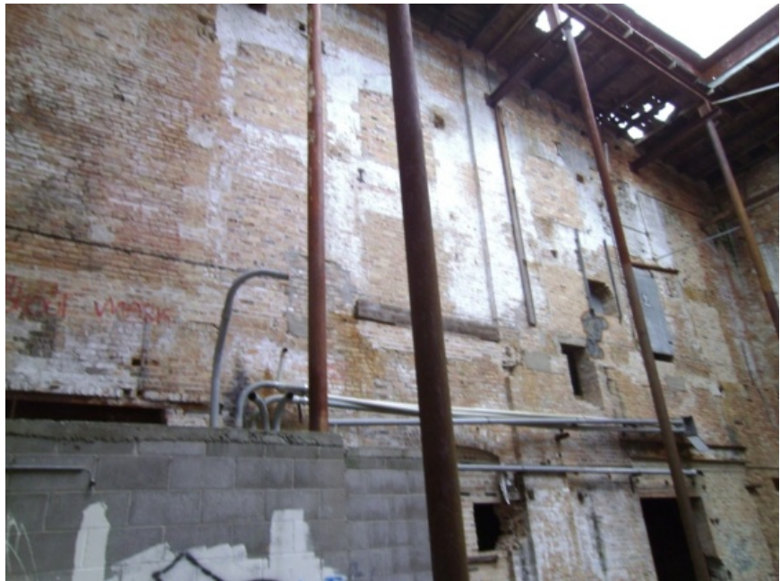
Image showing tall unstable columns. Note the holes present in the wood decking.
