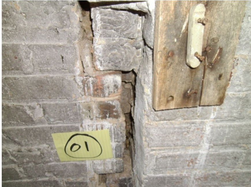
Image showing the poorly toothed joint at the south wall.
