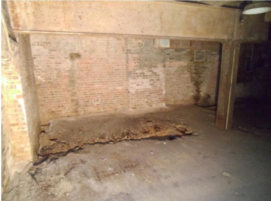
Image showing an area of the first floor collapse. Internal access to this room was not permitted.
