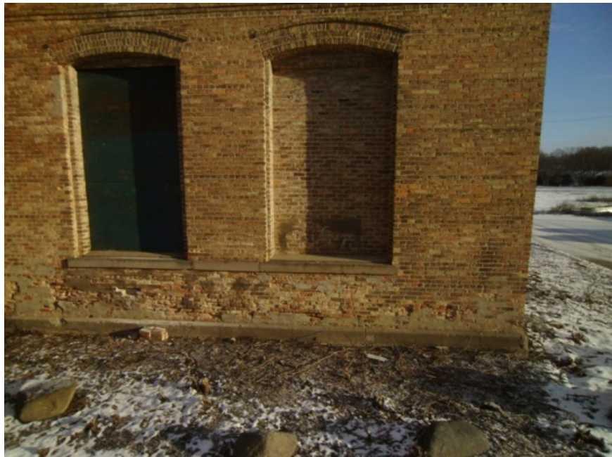
Image showing poorly performed patches at ongoing deterioration issues at the wall base.
