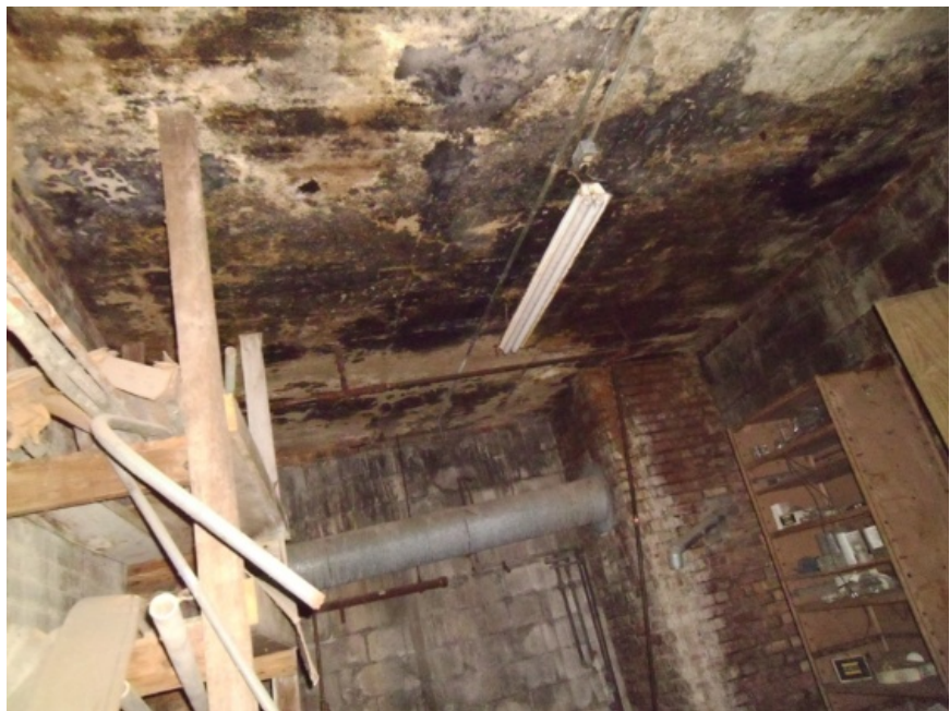
Image showing the underside of the concrete slab over the CMU vault.
