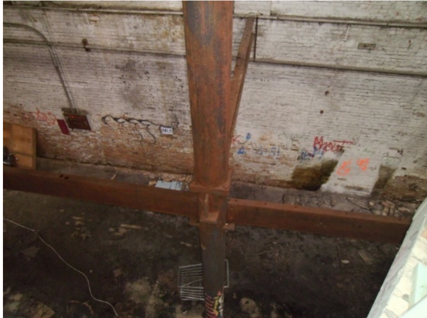
Image showing that the joints in the 1905 columns currently used to support roof structure are braced into the masonry walls.
