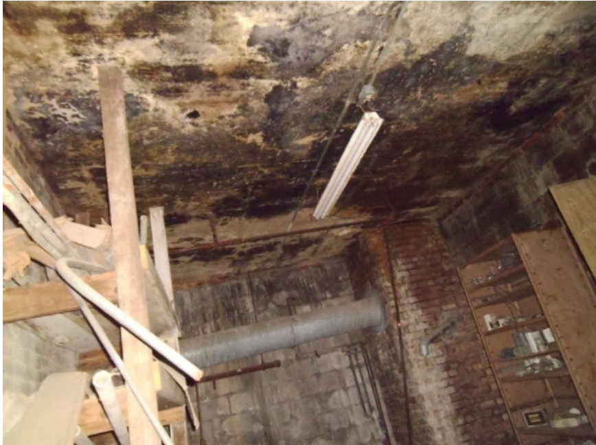
Image showing the underside of the concrete slab over the CMU vault. The stained areas are areas of water saturation and deterioration. The brick masonry at the lower right side is the bottom of the same chimney in the image above.
