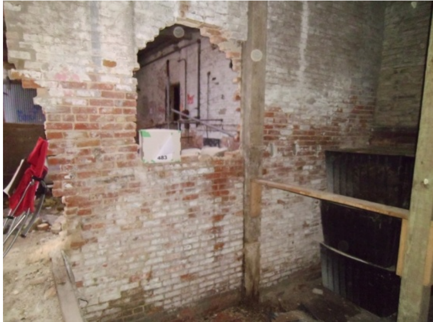
Image showing structural damage to the existing interior bearing wall. Besides missing significant sections of masonry, the red areas midway up and the green portions at the bottom are areas found to contain water damage.
