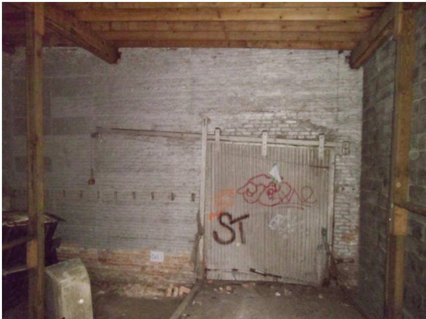
Image showing the west end of the module. Note the two beam lines supported by columns. The sliding door leads to Module J.
