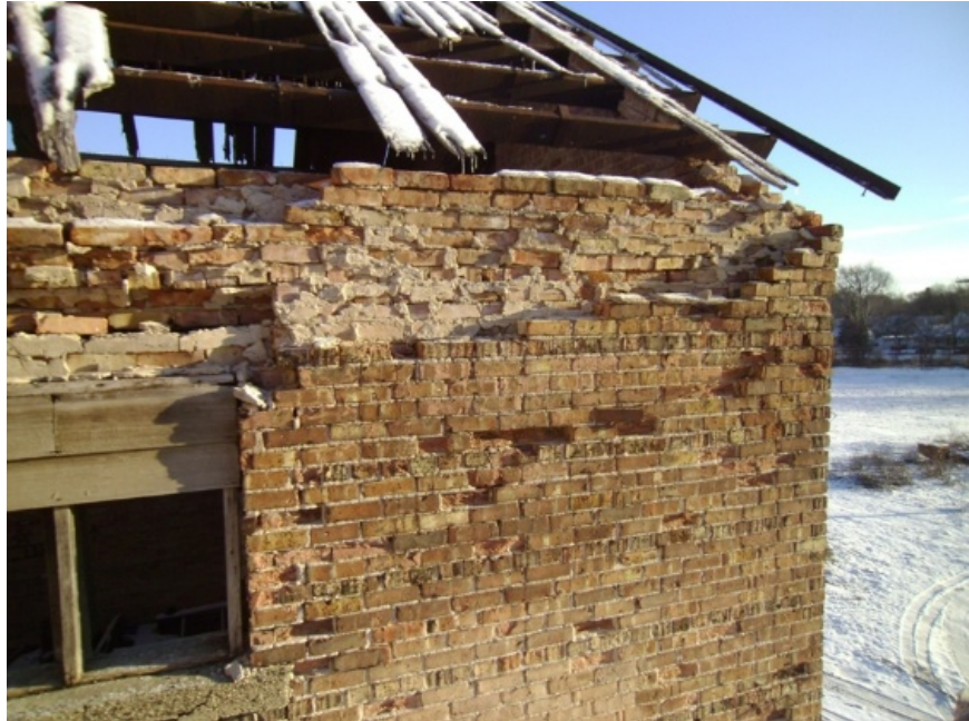
Image showing a section of the south wall. The extensive masonry deterioration extends at least to the underside of the window openings. Note the missing lintel section at the window opening.
