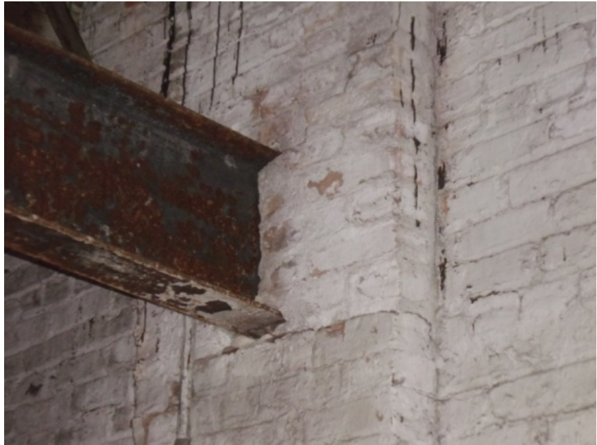
Image of a beam bearing into the masonry wall of Module A. Notice the horizontal crack below the beam and the diagonal step crack above the beam to the right.
