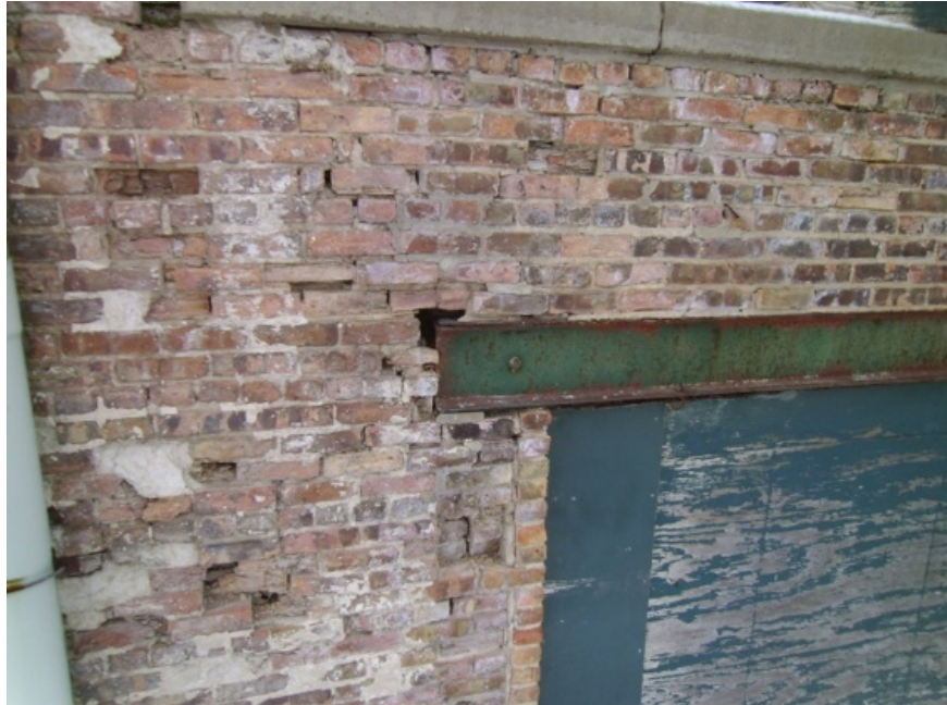
Image showing how deterioration and erosion in the masonry have undermined the integrity of a lintel's bearing.
