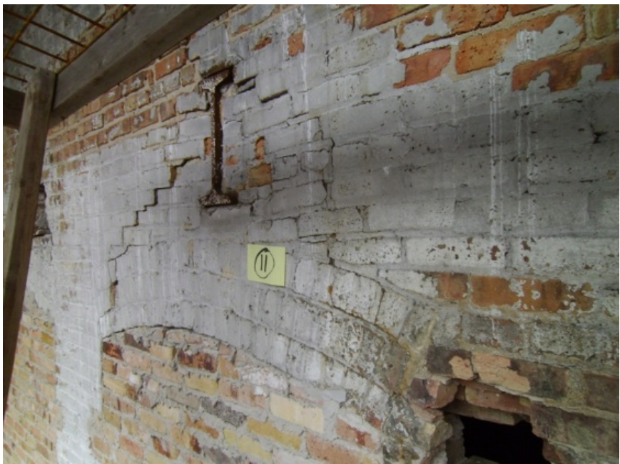
Images showing failed arched lintels of brick unit masonry, cracking at embedded steel, and brick and mortar erosion.
