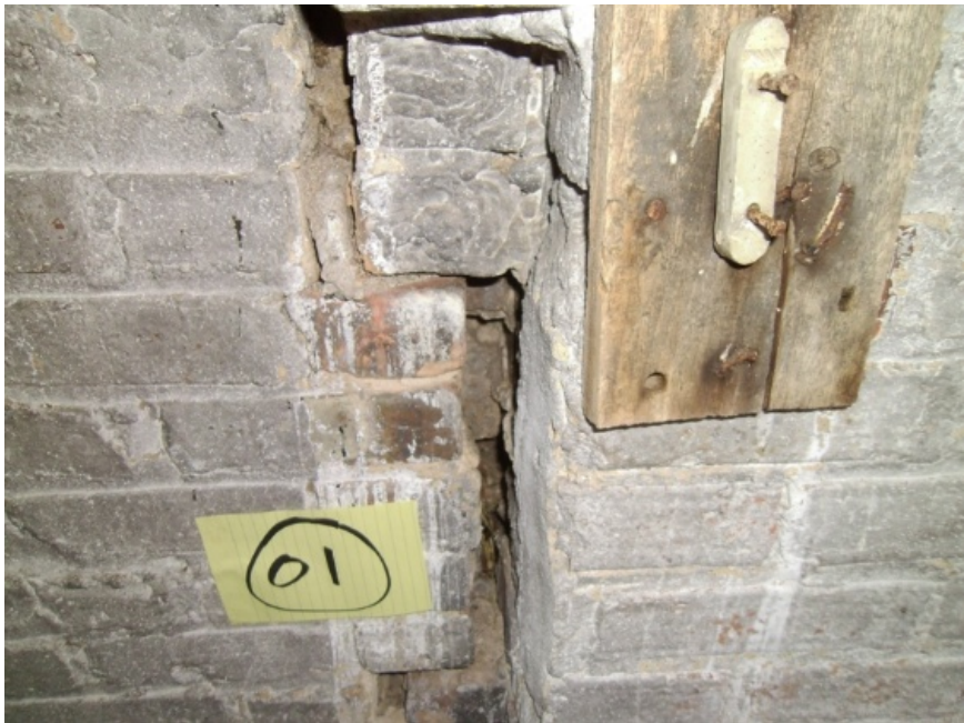
Image showing the poorly toothed interface at the south wall.
