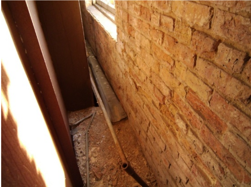
Image showing mortar and brick erosion, interior.
