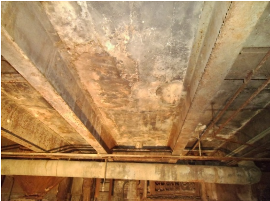
Image showing a portion of the floor construction of the second floor.
