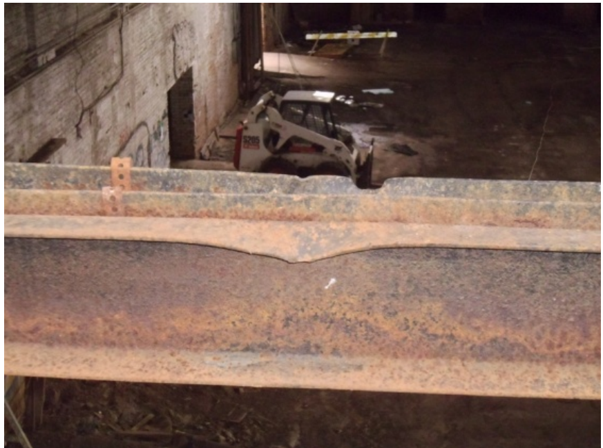
Image of a bottom chord that has been damaged by falling objects.
