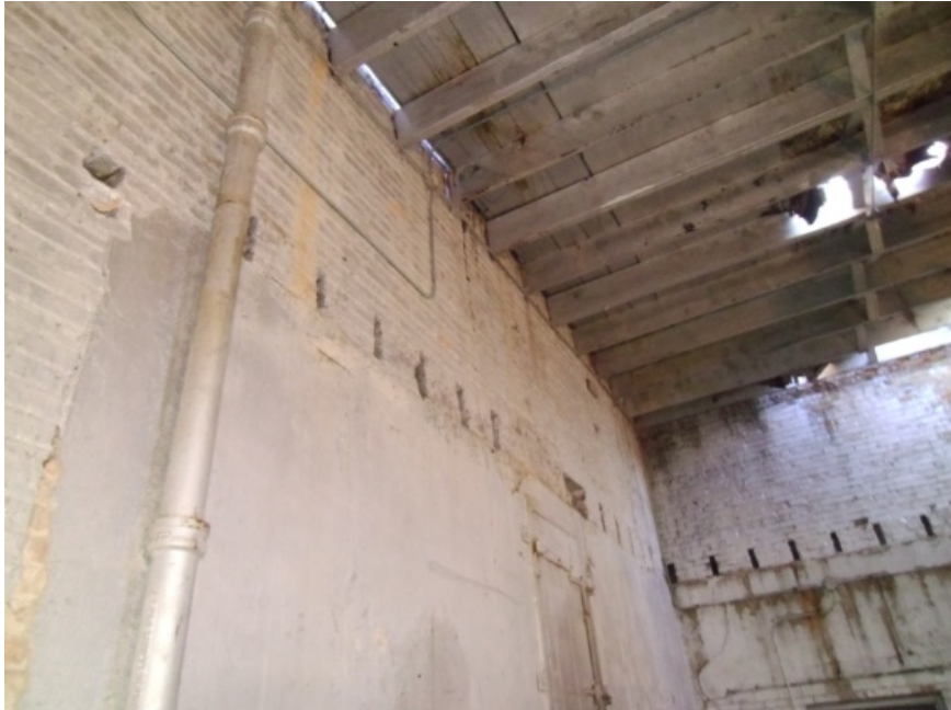
Image showing a damaged section of roof. Daylight shines through a void in the roof, along the wall: the region that had experienced fire damage.
