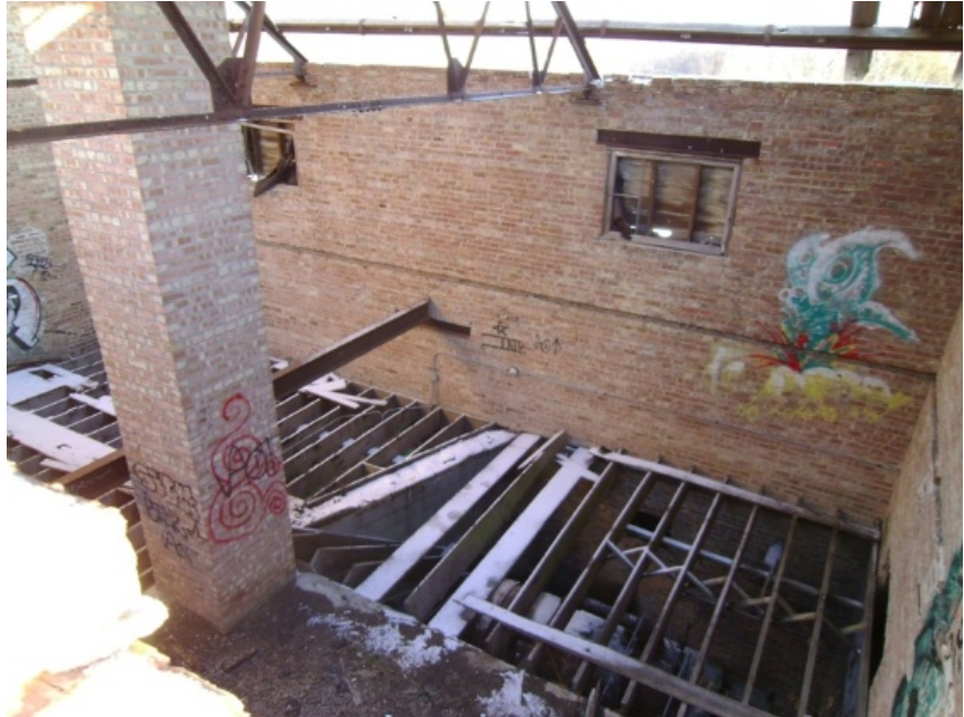
Image showing the existing wood joists of the second floor and the wall transition location 5' above.
