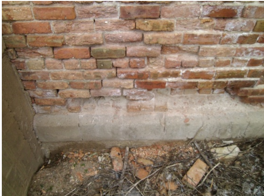
Image showing wall deterioration along its base at Module A.
