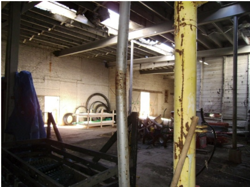
Image showing a damaged roof column. The bend has reduced the load carrying capacity of this column.
