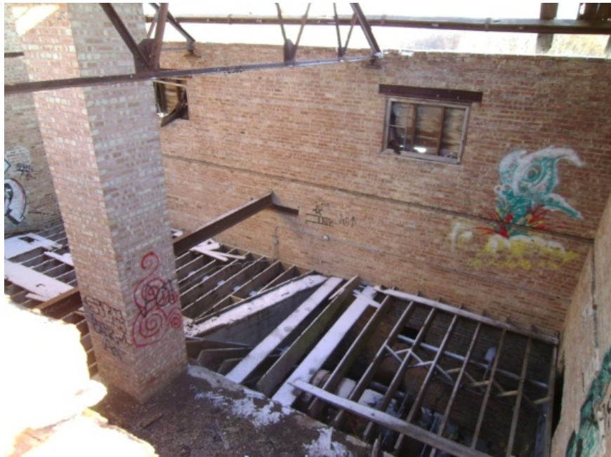
Image showing the north wall, interior side. Note the dark line below the windows. This is the change in wall thickness change from 12" to 8", back to 12"
