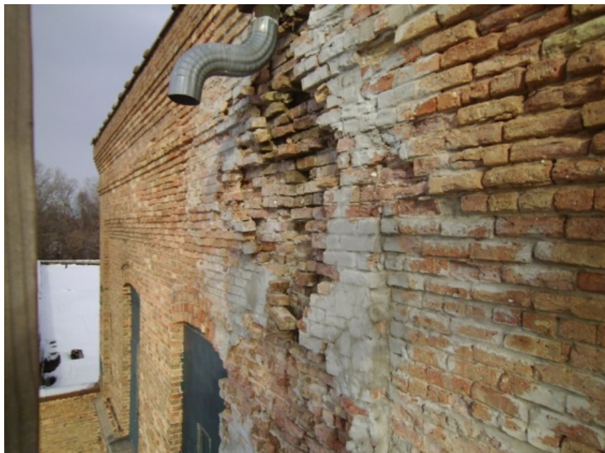
Image showing the upper section of brick deterioration from water infiltration. Large areas of missing brick and mortar can be seen. The
