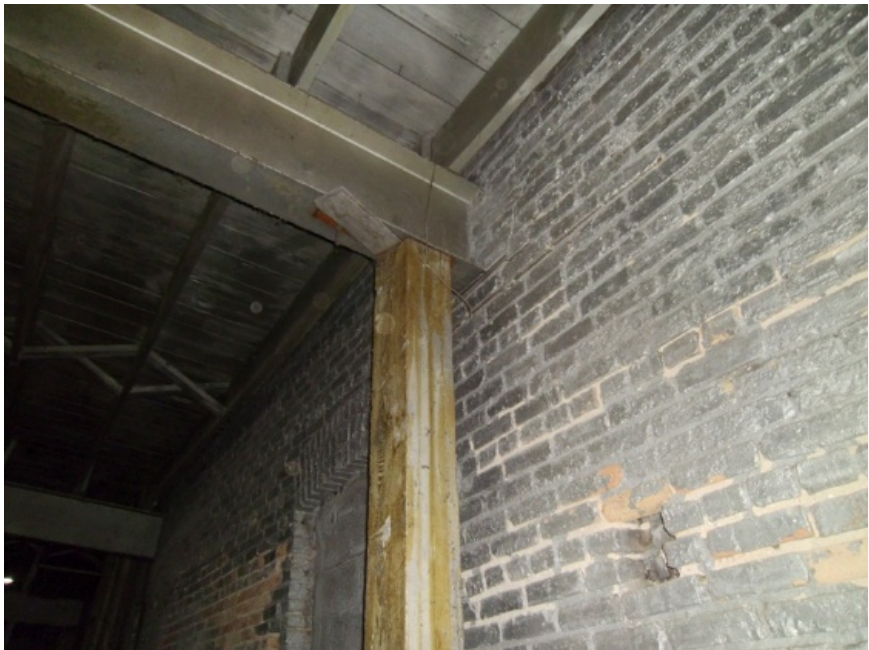
Image showing the shored end of a steel beam. Perhaps the shore has been added as a precaution in the event of a partial wall collapse.
