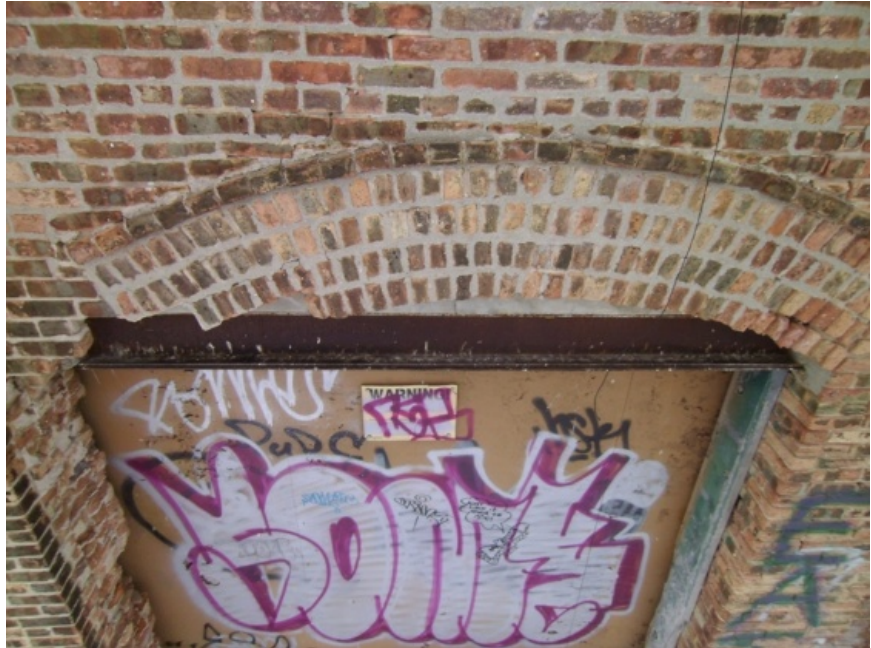
Image showing the poorly constructed steel lintel at the north wall. The steel supporting the masonry only supports a portion of the wall width. The left bearing is compromised.
