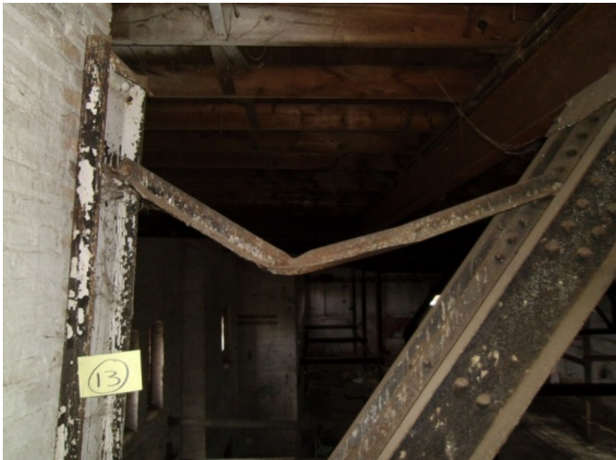
Image showing the bent stabilizer from the truss to the masonry wall.
