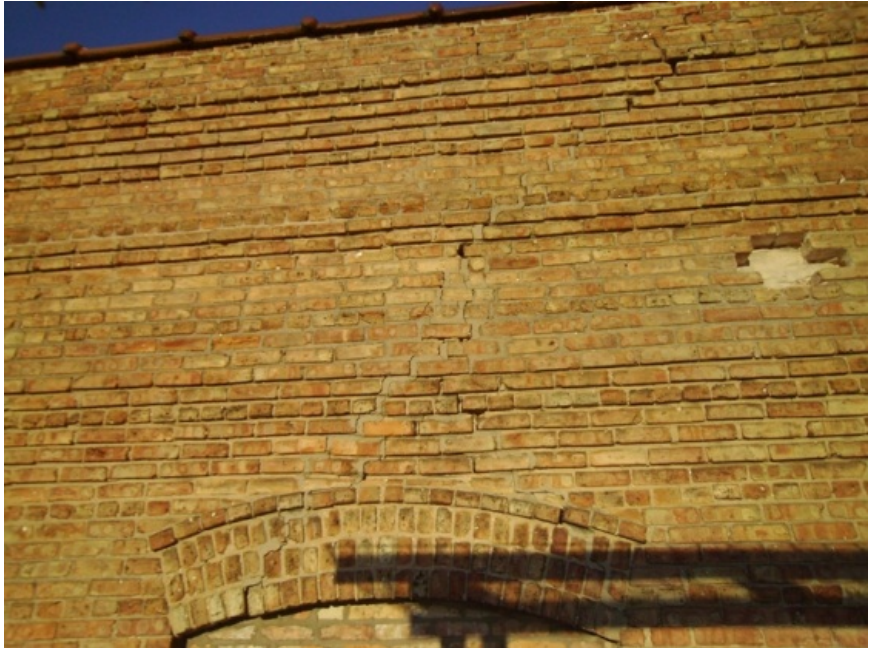
Image showing a stepped structural crack from a second level lintel to the roof.
