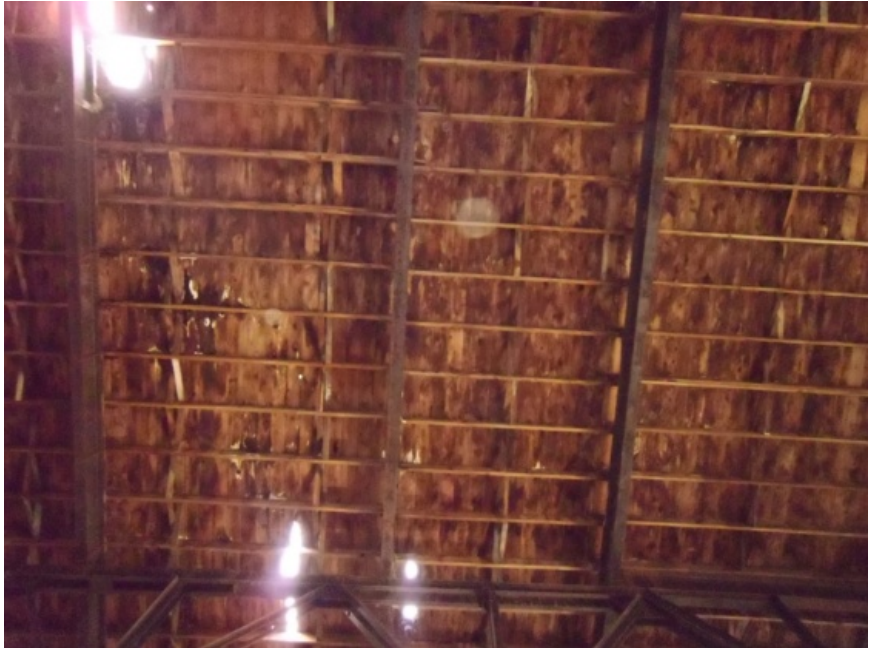
Image showing a view of the underside of the deteriorated wood roof framing at Module A.
