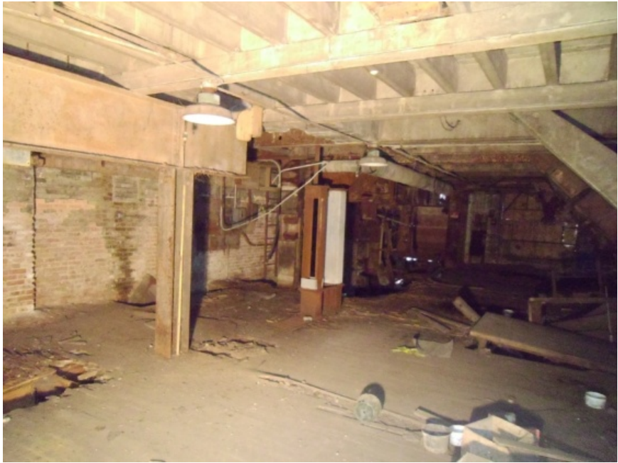
Image showing another region of Module G. This floor system is wood joist covered with a concrete slab. The framing appears to be in good condition.
