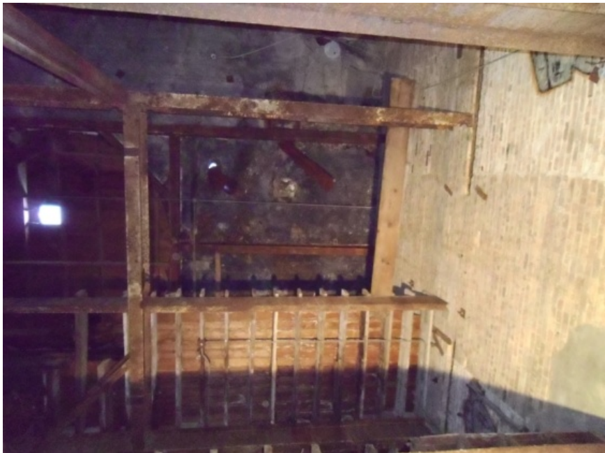
Image looking upwards at the roof framing. The wood framing at the bottom of the image is the third floor. Steel beams and columns support the wood framing.
