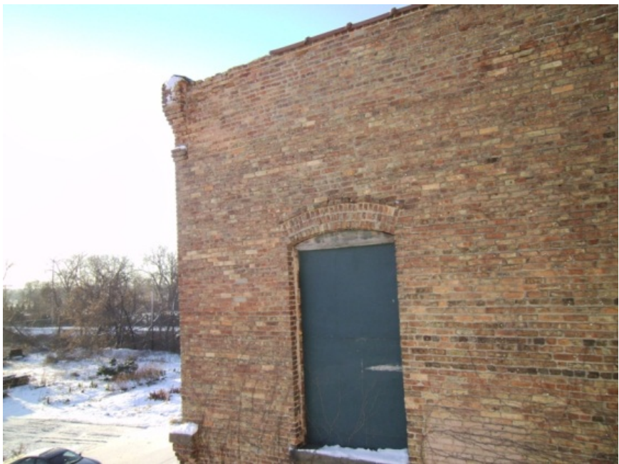
Image from the north at the second floor northeast corner of Module B. A section of parapet has lost its cap and allowed moisture to migrate into the corner of the building.
