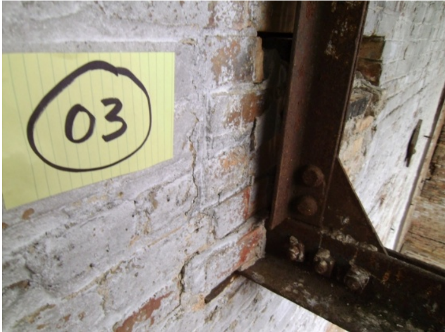
Image showing a truss bearing at the south wall. Note the cracks in the masonry suggesting that the truss is being tugged out of the masonry.
