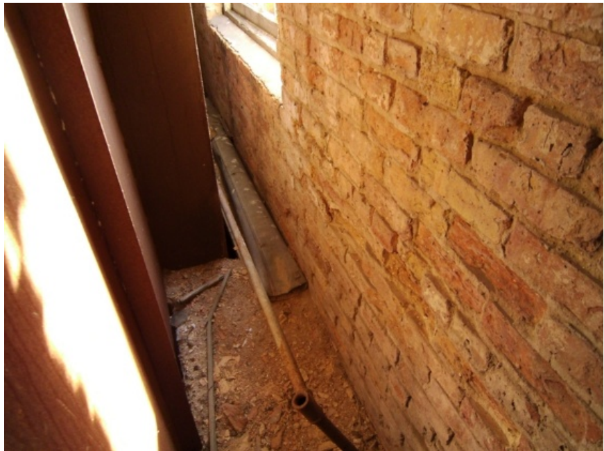
Image showing the interior mortar erosion and brick damage.
