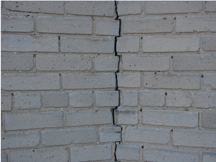
Figure 6. Vertical cracking at an obtuse corner in the brick party wall.
