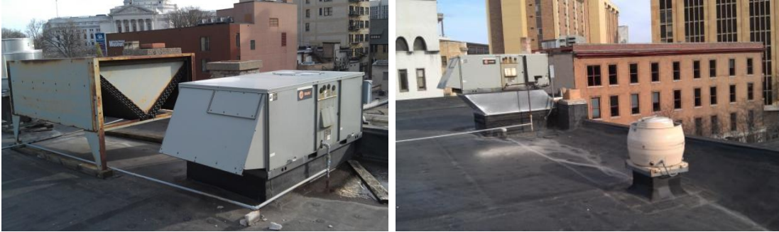
Existing rooftop equipment
