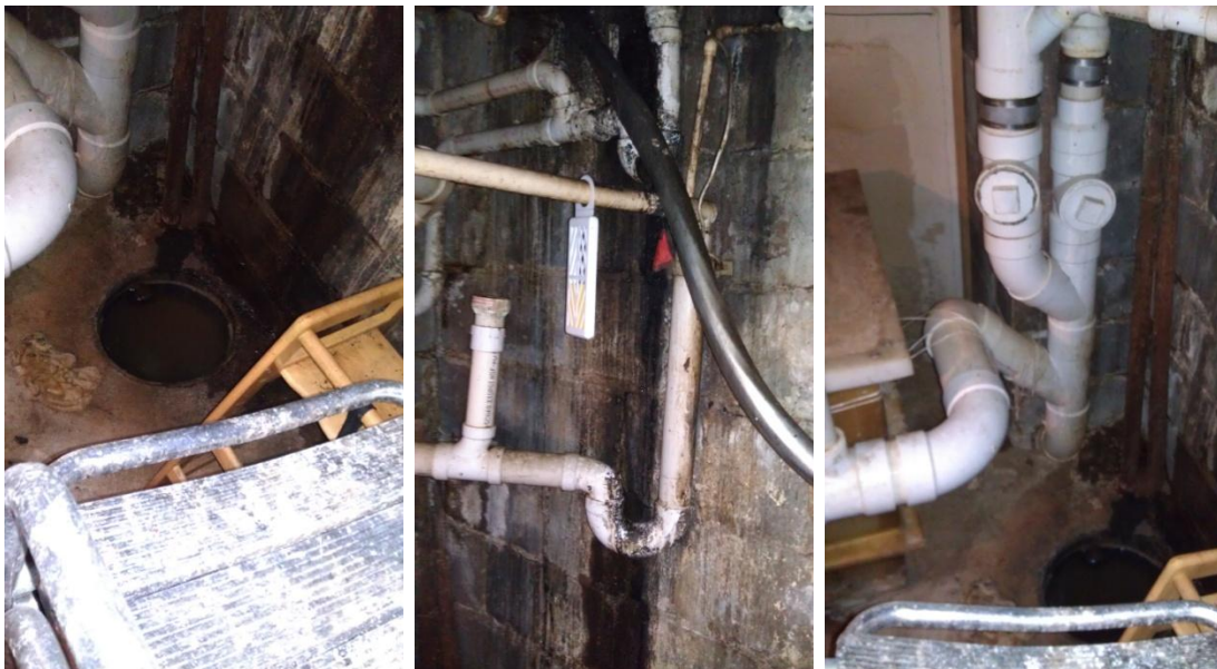
Poor condition of sanitary piping
