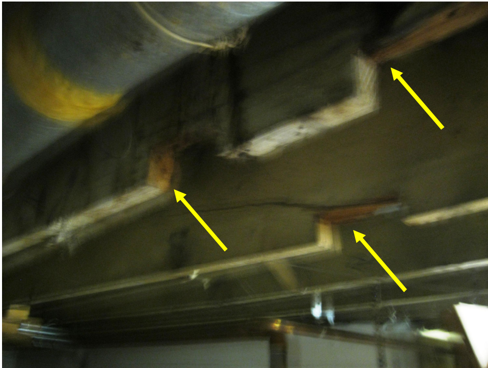
Photo 6 – Notched 1 st floor joists
