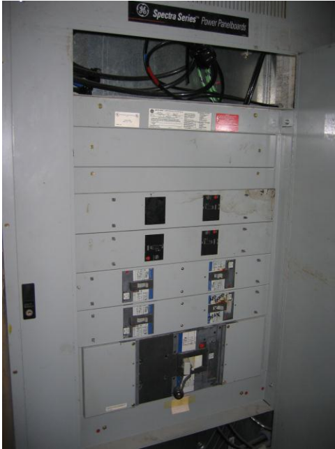
Distribution panel in the basement.
