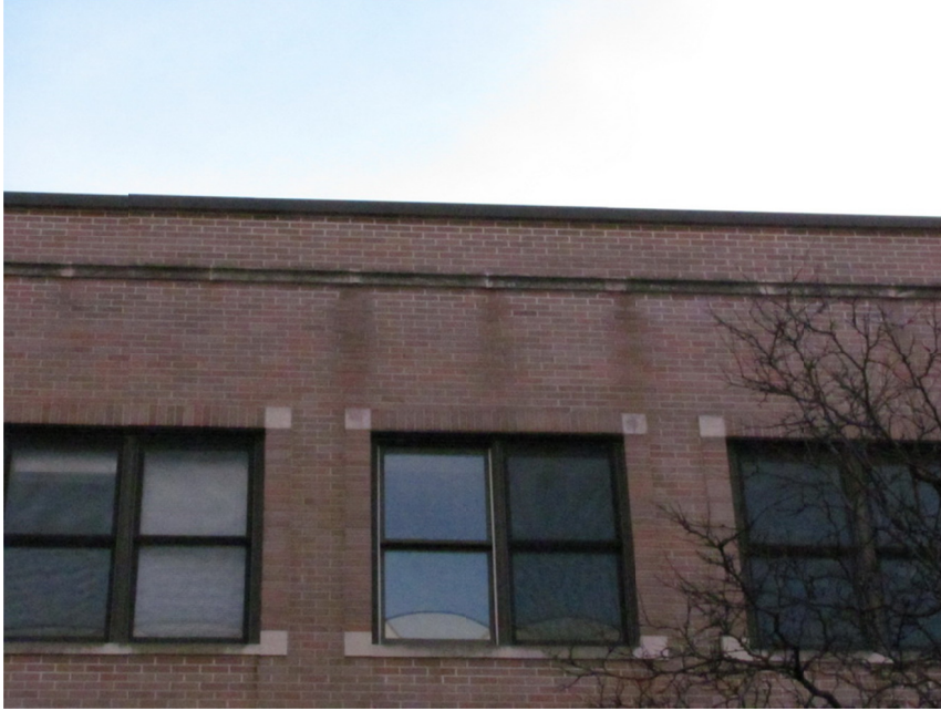
Figure 3. Water rundown staining below the stringcourse at the parapet wall.
