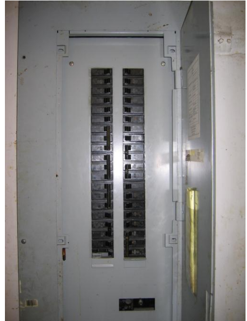
Electrical panel on 1 st floor restaurant.
