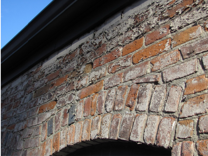
Figure 13. Remnants of a previous coating on the masonry were observed.
