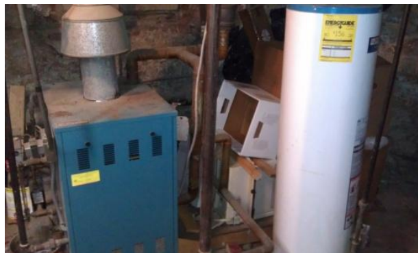
Hot water boiler and water heater
