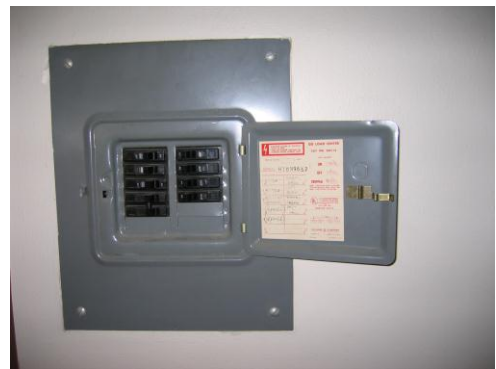
Electrical panel 125 1/2 State Street (2 nd floor apartment).
