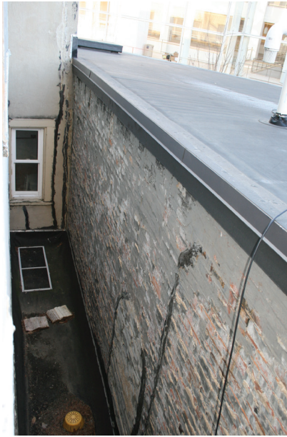
Exterior: View of side wall (party wall) between 125 state street and 121-123 State Street
