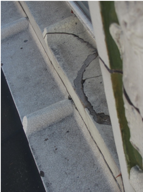
Figure 3. One cracked terra cotta window sill.
