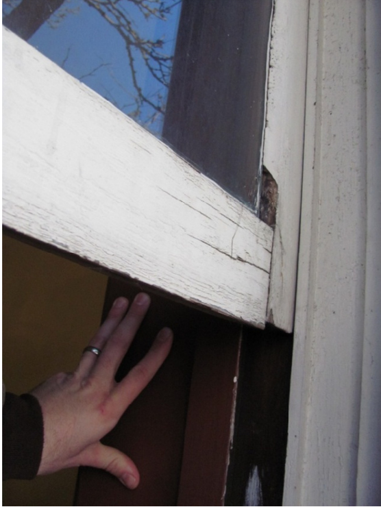
Figure 8. The wood windows are in fair condition, with some wood decay and displacement of window sash joinery.
