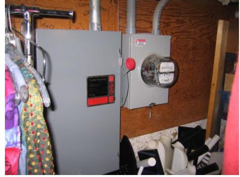
Basement electrical meter and disconnect.
