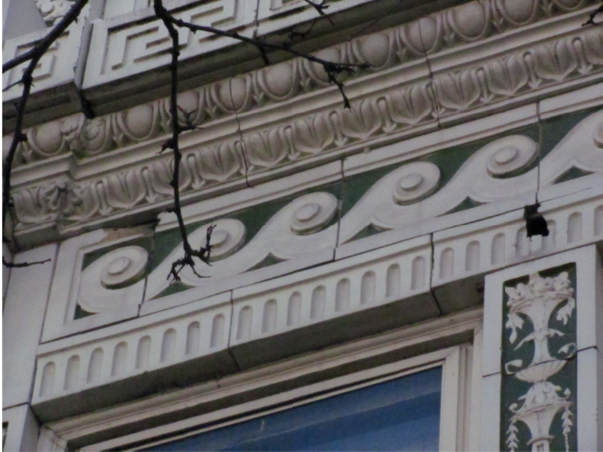
Figure 4. One unit with a hole and one spalled unit.
