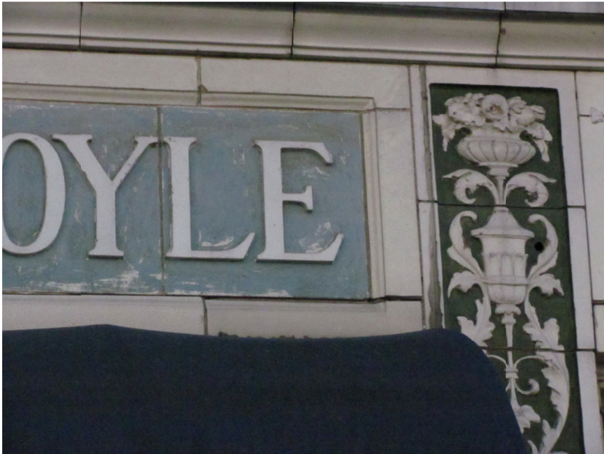
Figure 5. One displaced unit above the first floor storefront.
