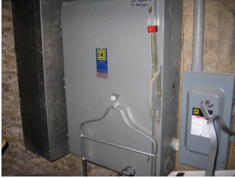
Building main disconnect.
