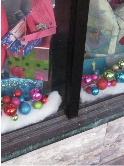
Figure 6. An aluminum mullion has been added at the center of the storefront at the first floor of the State Street facade.
