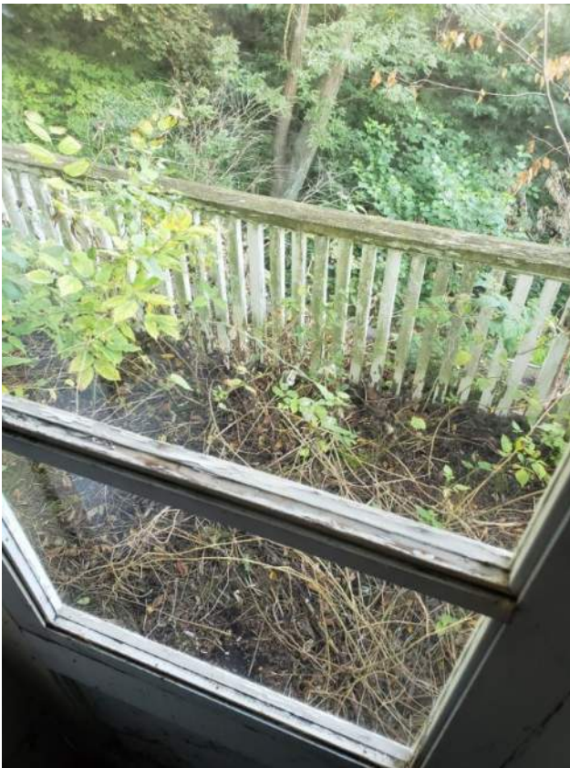
Upper Porch (above Kitchen) – excessive lack of maintenance has caused vegetative growth producing significant water damage to Kitchen below.
