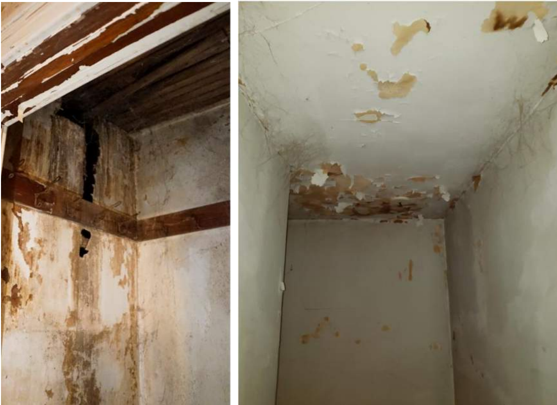
Upper Bedroom & Hall – evidence of moisture intrusion causing failing paint and palaster
