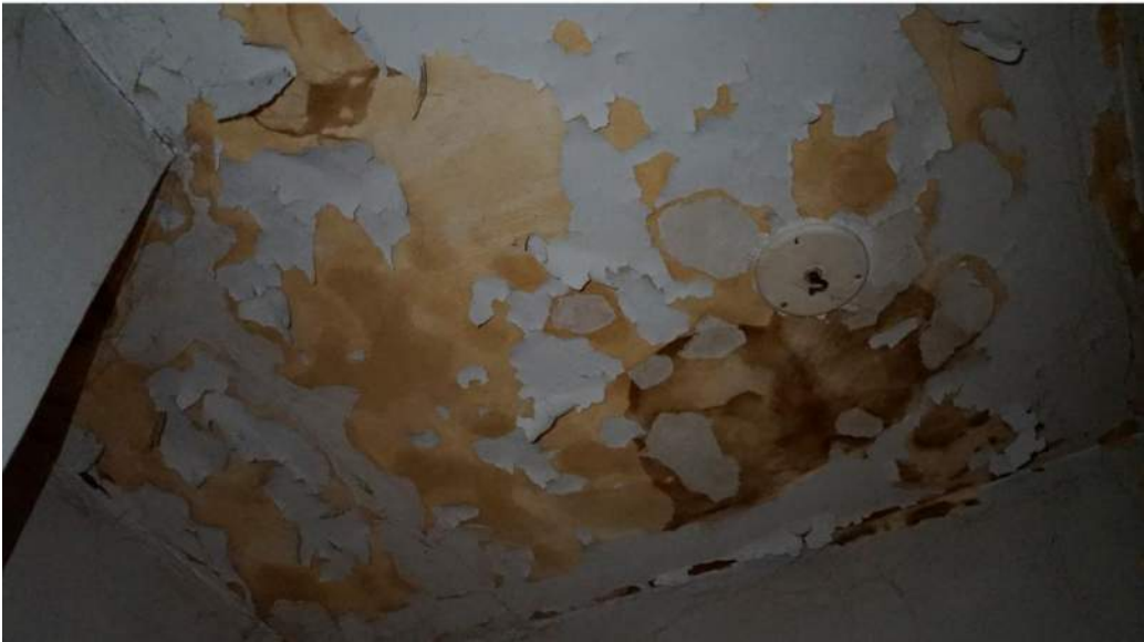
Upper Bedroom – evidence of moisture intrusion causing failing paint and plaster
