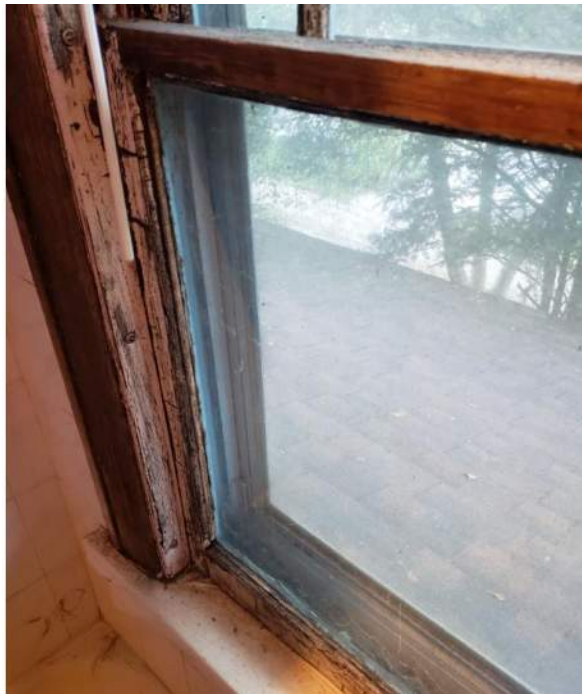
Windows – all the windows of the house are single paned and dry rotted.
