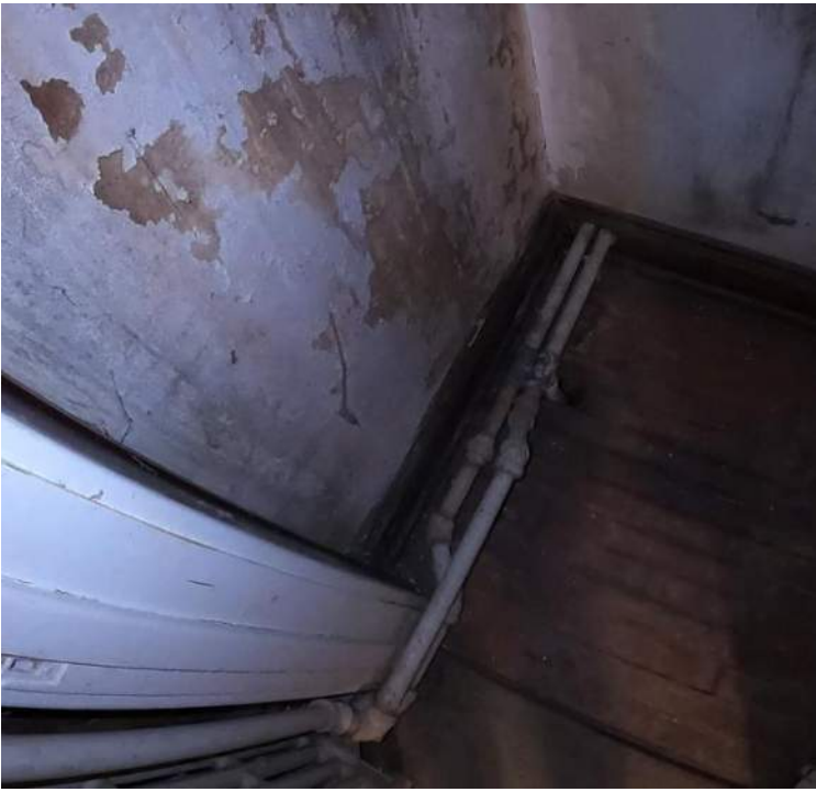
Upper Floor – wood floors are damaged and past their life, exposed pipes through-out.
