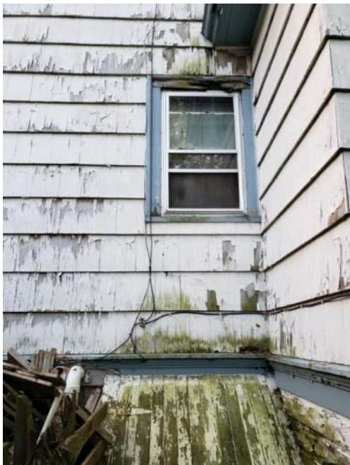
Exterior at Main Level Kitchen – wood rot
