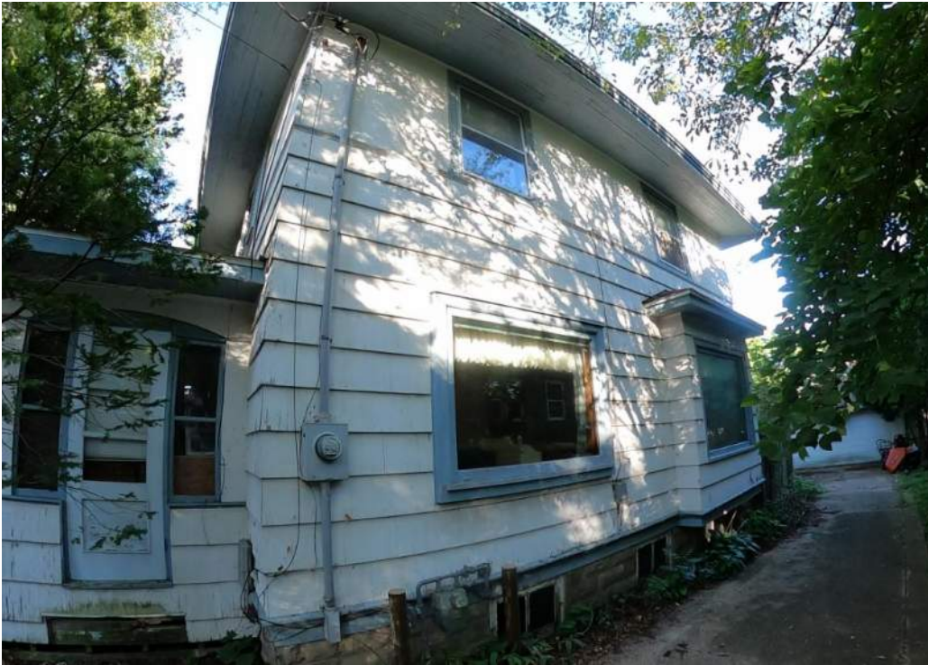
Side of House - Garage Side (north) – The windows are deteriorated and rotten, cedar is in a tired state and is not reusable, foundation is in an acceptable condition, however moisture migrates into basement during rain events, Basement ceiling is low. Overhead Electrical Line. Location of Gas meter.
