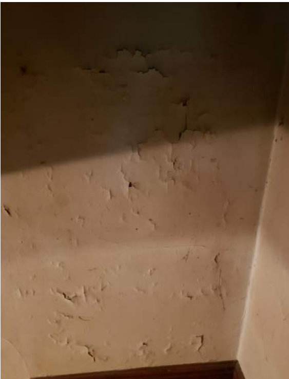
Exterior wall at stair – moisture penetrating through wall due to inadequate flashing
