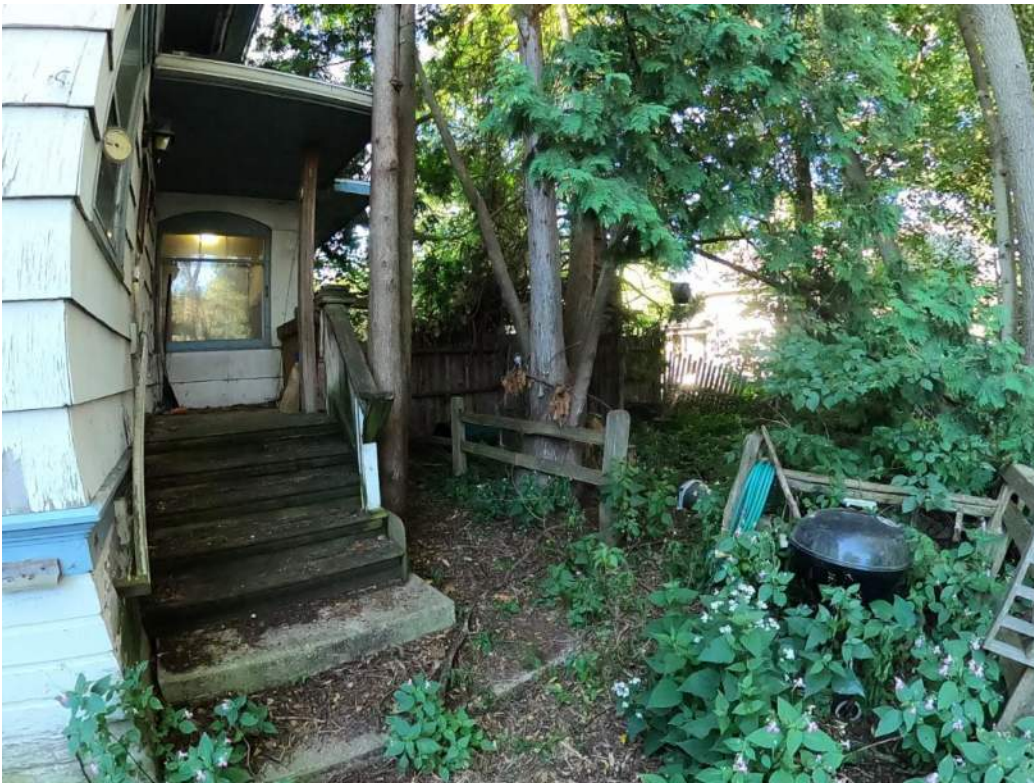
Side Porch – evidence of moisture intrusion at the roof, deteriorated stairs and railing. The side porch walls and roof are undersized structurally and roof is leaking.
