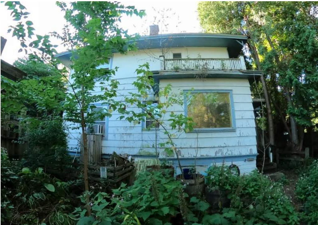
Exterior Rear Elevation – Exterior is cedar , evidence of significant water infiltration and lack of maintenance. The area with the picture window is the kitchen. Failing moisture barriers at the upper porch floor/roof has caused significant water damage and mold on the addition and existing exterior wall.
