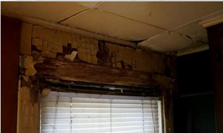
Main Level Kitchen – evidence of moisture intrusion causing falling ceiling, rotted window head and mold. See attached images of porch causing water damage. The kitchen addition requires complete removal.
