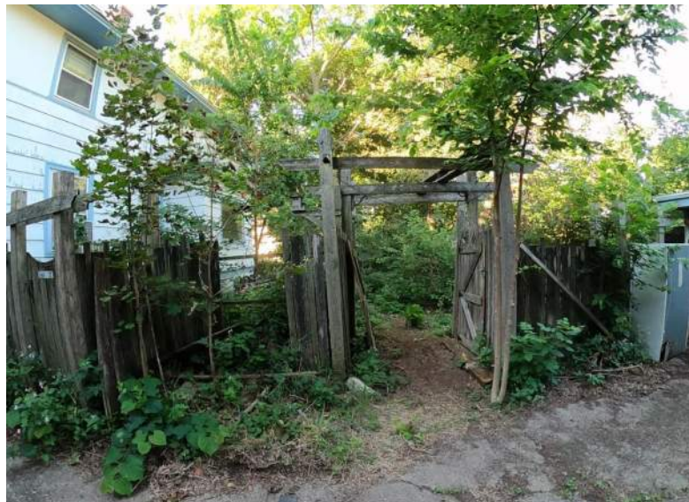
Rear yard – fence structure is deteriorated, needs removal
