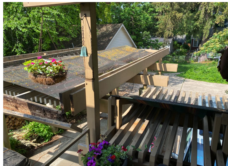
ROTTING STRUCTURE, CANVAS ROOF, NO GUTTER OR RAIN WATER MANAGEMENT.
