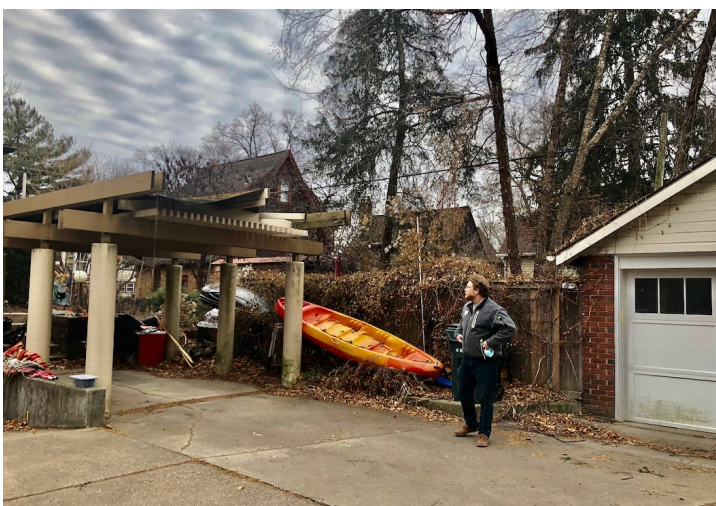
CARPORT ADDED IN THE 80'S. THE ROOF IS CANVAS AND THE WOOD STRUCTURE IS ROTTED BEYOND REPAIR AND WOULD REQUIRE CONSTRUCTION. CONCRETE COLUMNS IMPEDE CAR-DOOR CLEARANCE. LOCATION OF THIS CAR PORT RESTRICTS PEDESTRIAN ACCESS TO THE BACK DOOR ENTRY OF THE HOUSE.
