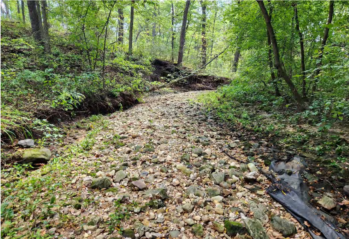
Figure 3. Bank and bluff erosion observed in the armored lower segment of Pennito Creek. Note large bar of mobile bedload and exposed underlying geotextile fabric (photo Inter-Fluve).
