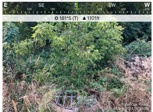
Photo #6 Photo point 3, culvert with box elder trees in riprap on the southwest side of the infiltration basin.
