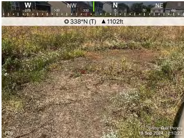
Photo #15 Photo point 8, view north-northwest toward the western portion of the infiltration basin
