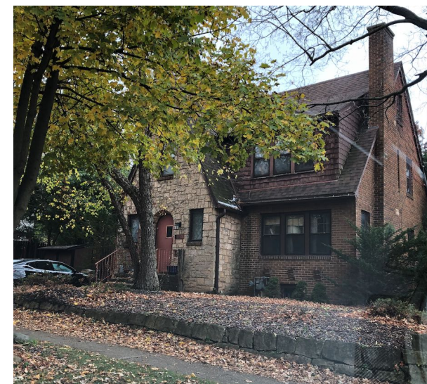
122 N. ALLEN ST - DEMONSTRATES SHED DORMER ON STEEP SLOPE OF SECOND LEVEL ROOF TO PROVIDE HABITABLE SPACE UNDER THE ROOFLINE. DORMER IS CLAD IN WOOD MATERIAL.
