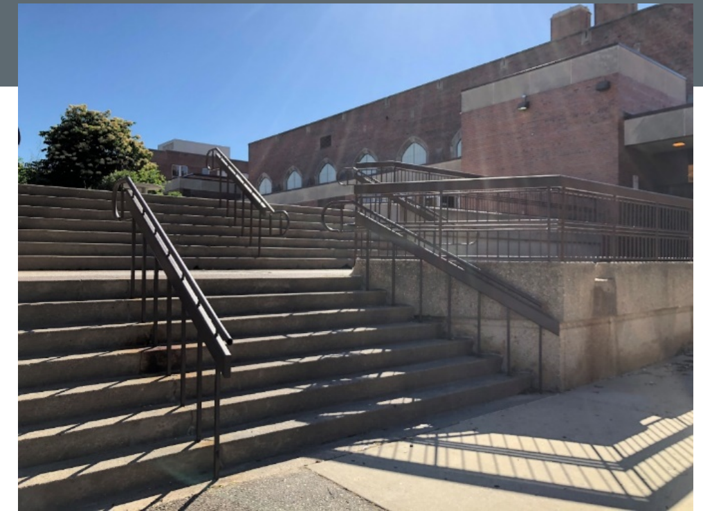
View of stairs to Plaza that are to be removed for addition.
