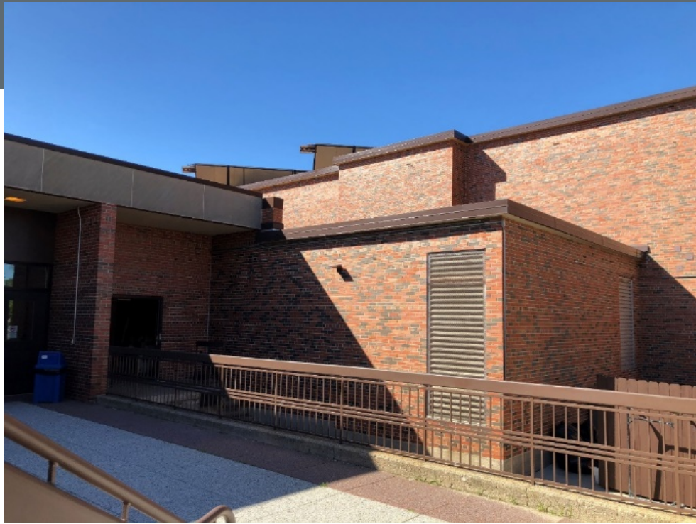
Standing on Plaza looking at site of addition. View of existing louvers on the locker room wall, pool beyond.
