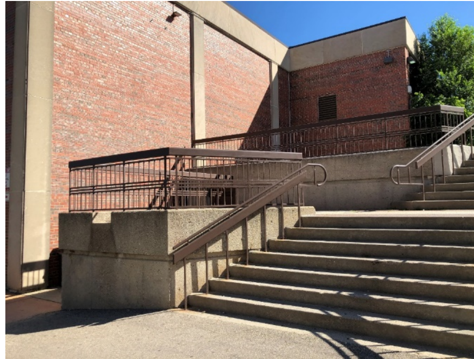
View of stairs to Plaza that are to be removed for addition, Fieldhouse beyond.
