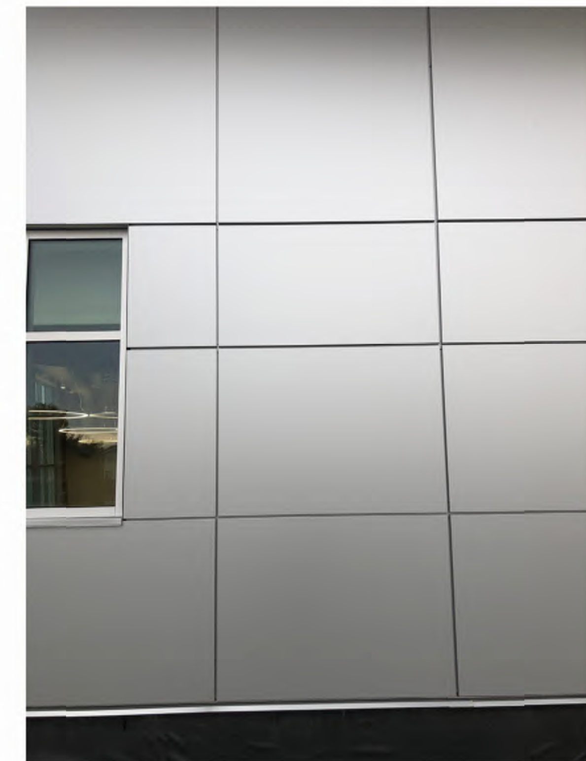
METAL WALL PANEL, COLOR SHALL BE CLEAR ANODIZED AS MANUFACTURED BY ALPOLIC MATERIALS
