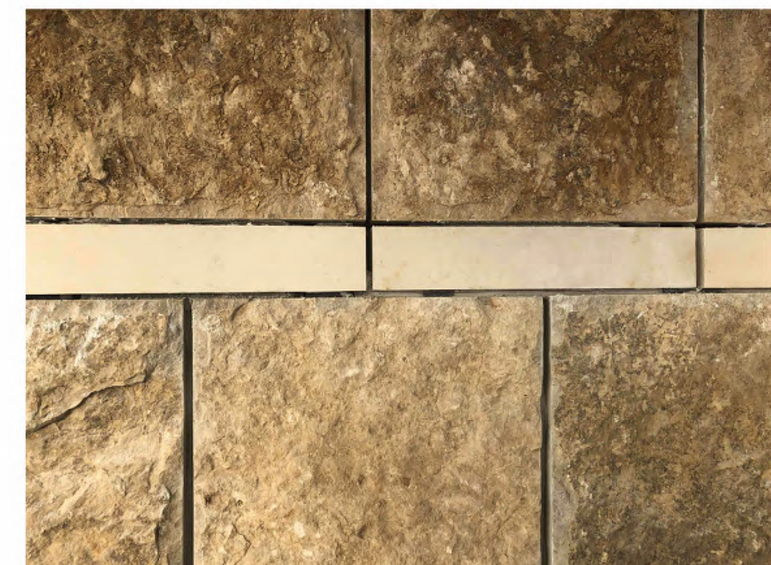
STONE VENEER, MAIN PANELS SHALL BE LIMESTONE WITH A BED FACE FINISH, COLOR SHALL BE PRAIRIE BUFF/GOLD, NOMINAL SIZE 3'-8" HIGH BY 1'-8" WIDE. ACCENT PANELS SHALL BE LIMESTONE WITH A HONED FINISH, COLOR SHALL BE AURORA BUFF, NOMINAL SIZE 4" HIGH BY 1'-8" WIDE AS MANUFACTURED BY QUARRA STONE COMPANY
