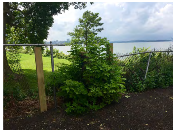
Gap in Fence
