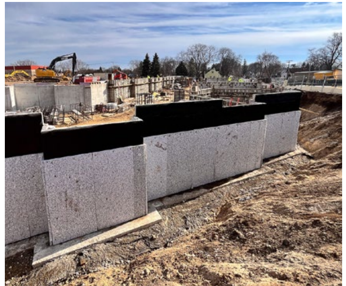
RISE Madison under construction at the former Gardner Baking site on East Washington Avenue
