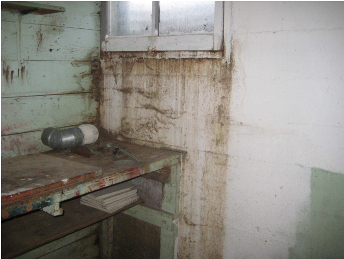
LEAKING WINDOW WELLS
