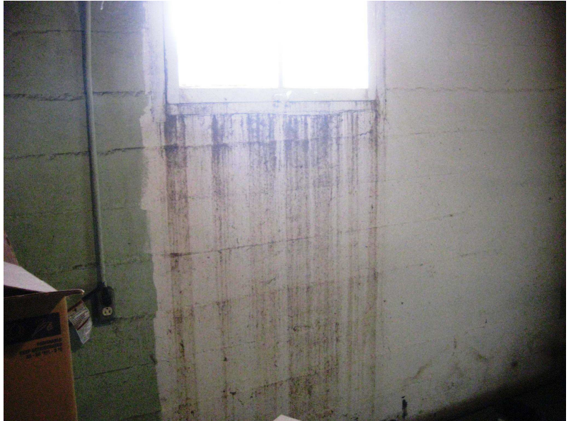
LEAKING WINDOW WELLS @ BASEMENT
