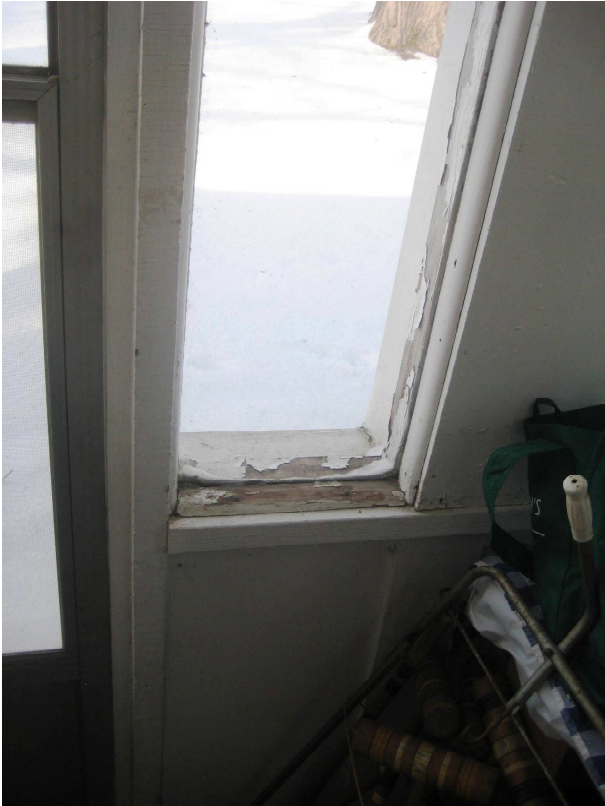
INTERIOR WINDOW CONDITION
