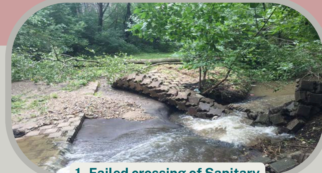
1- Failed crossing of Sanitary access path near Randolph Dr and Tree Ln
