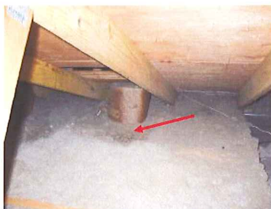
Kitchen fan exhaust is not properly venting to the exterior of home. Insulation has been displaced and R-value is very low. Bottom picture shows where moisture has leaked onto insulation, this area is above moisture stains in kitchen.
