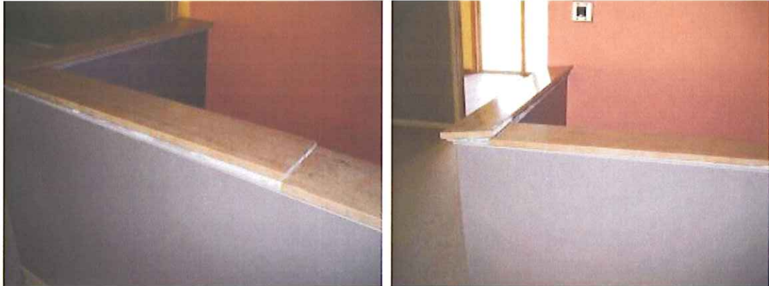
Granite slabs on top of basement stairs are not properly secured down and could be possibly knocked off and down staircase.
