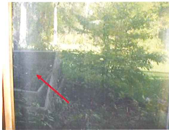
Windows on west wall in basement have failed thermo pane seals allowing moisture in between glass panels.
