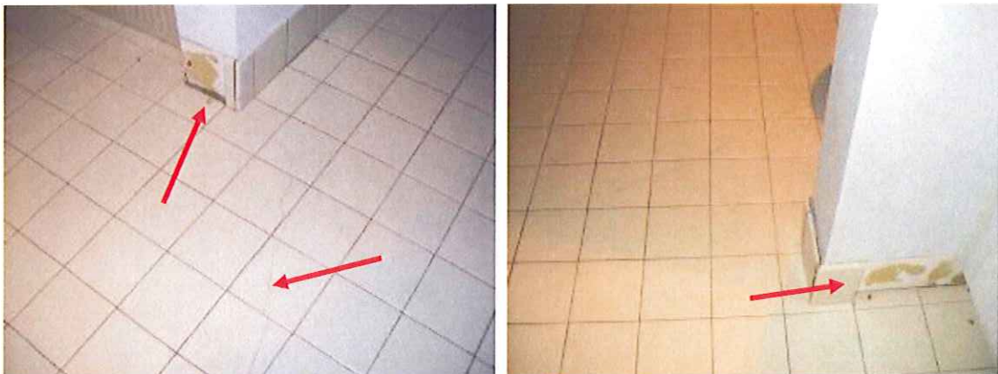
Missing wall tiles and cracked floor tiles in basement bathroom.
