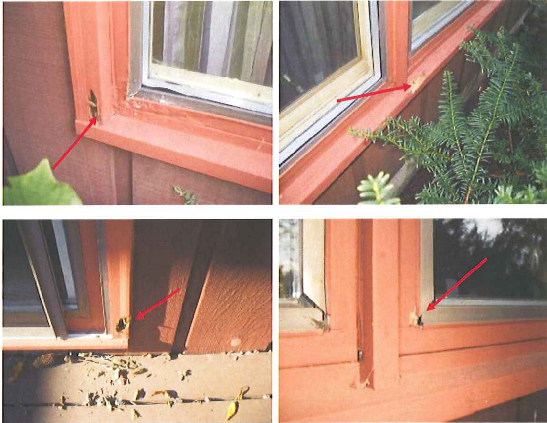
Wood rot around window sills, frames and patio door frames. Wood was painted over to hide wood rot. Majority of windows and door frames are in need of replacement.
