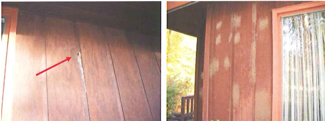
LP T-11 siding manufacturer has had a class action lawsuit against them due to premature rotting and warping of wood. Siding has been damaged over the years by woodpeckers and has large holes in it; recommend replacement.
