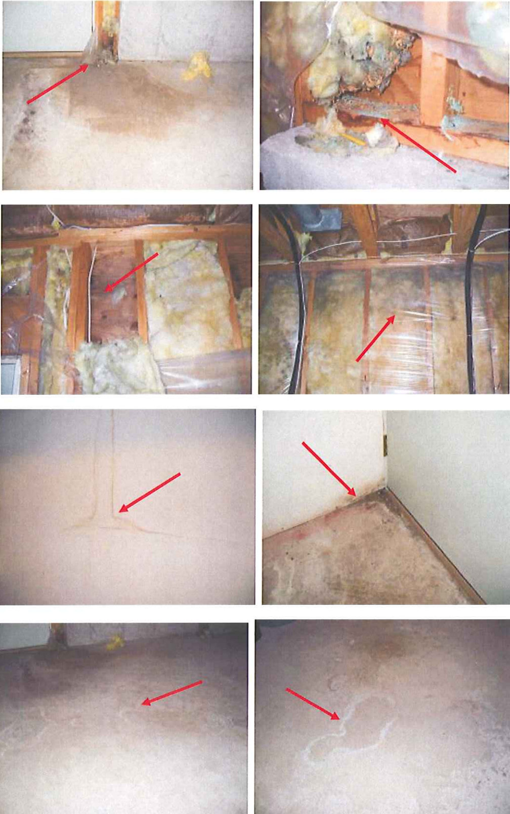
Areas of water seepage on floor, moisture damage and possible mold growth on insulation, walls and floor in furnace room.
