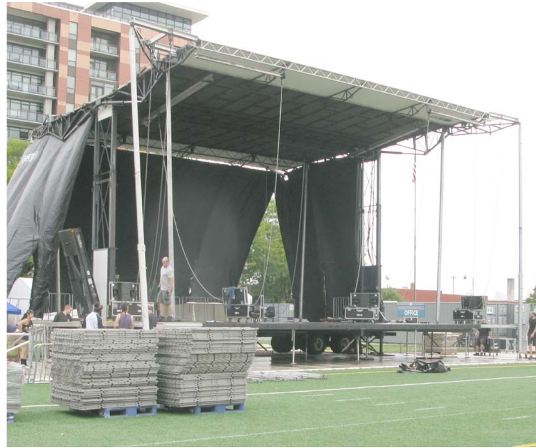
07 CURRENT CONCERT LOAD-IN AND OUT REQUIRES PAVING
