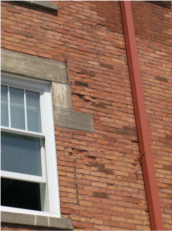
Picture 5961: Typical damaged brick
