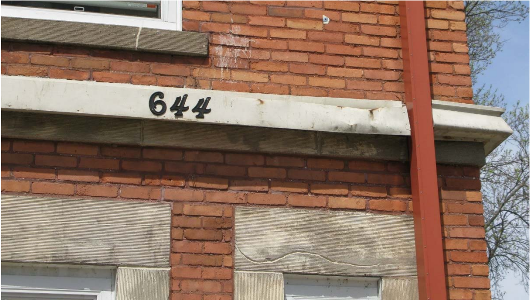
Picture 5977: Damaged non-original metal banding
