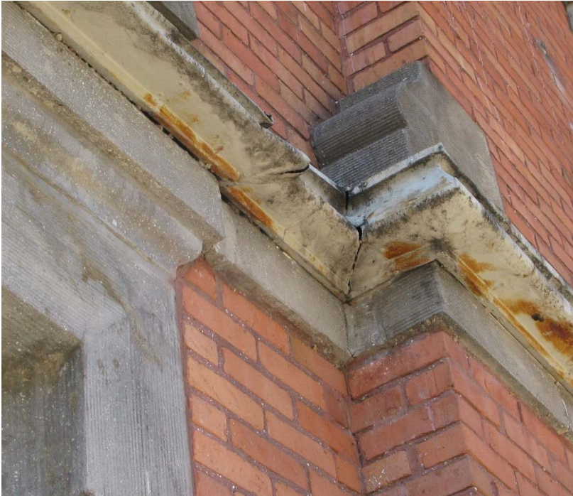
Picture 5913: Damaged original metal banding
