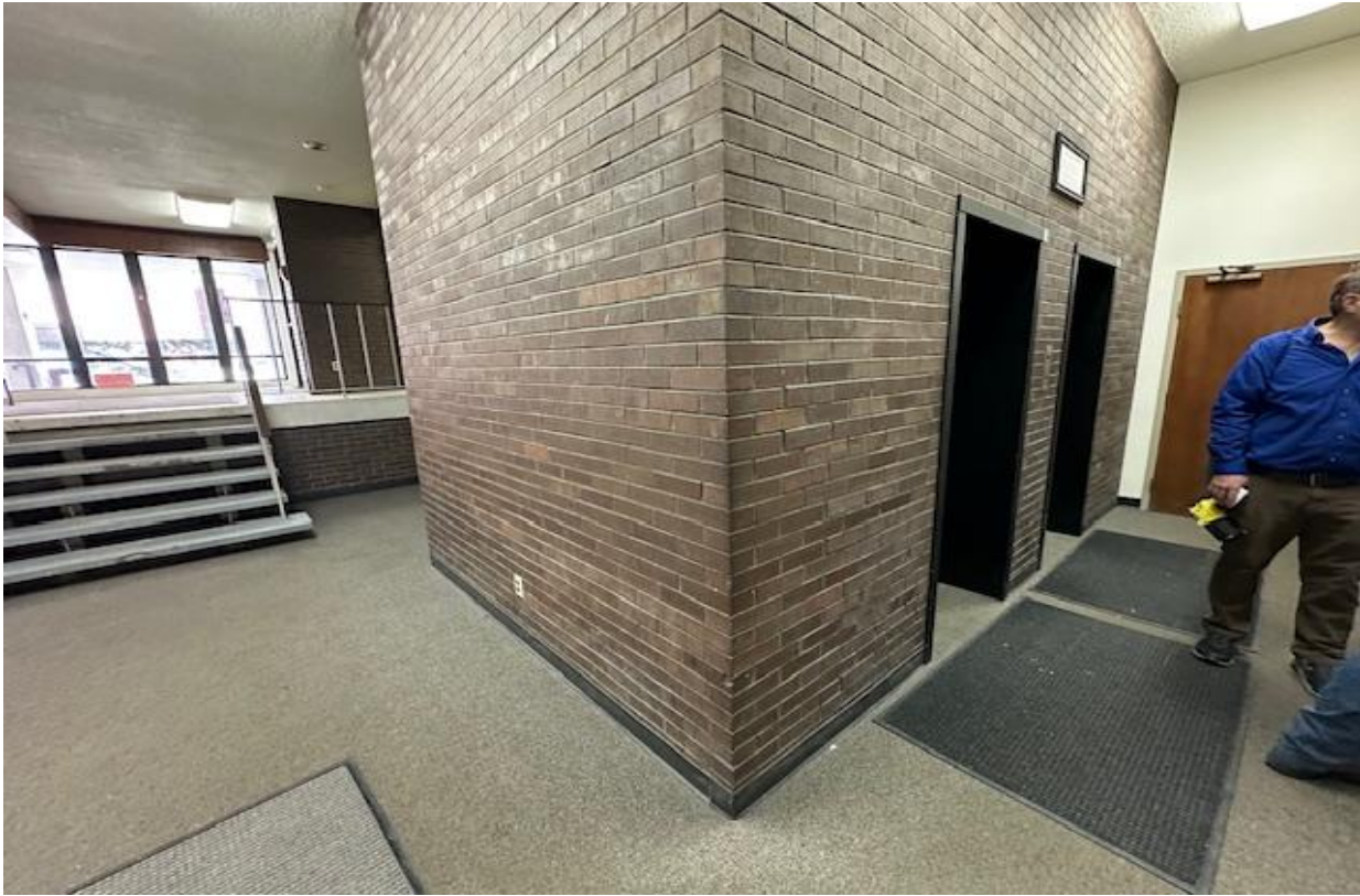
Insufficient available space for LULA elevator between vestibule lobby and first floor.
