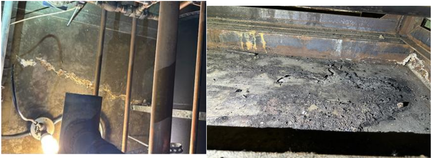
Calcification at underside of penthouse roof / Spalling of penthouse floor deck - Roof deck.
