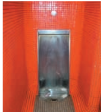
Stainless fixture and hidden valves in the Auditorium Park men's restroom.
