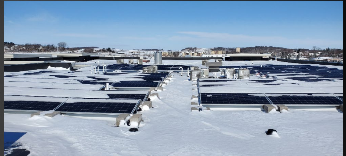
Pictured: One of JT Klein's rooftop solar panel arrays
