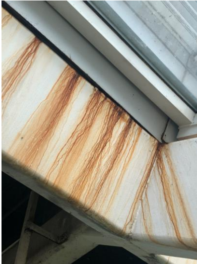
“Tear staining” of surface rust on the structural tubular steel.
