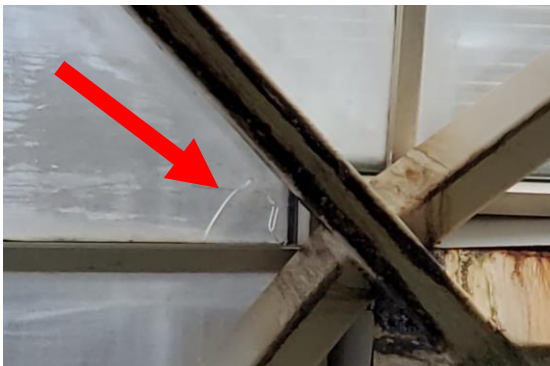
Cracked glass near cupola
