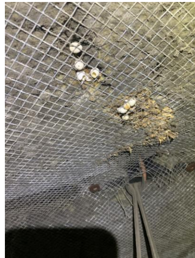
Mushrooms growing in the cupola insulation.
