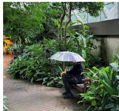
Failed sealant, raining inside
