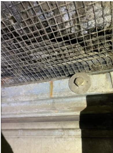
Moldy, deteriorating insulation in the cupola roof.
