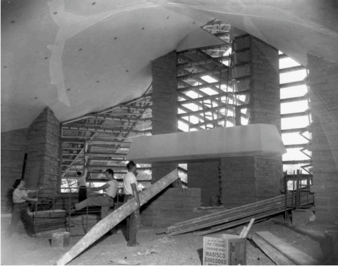
August 19, 1951 before: Unitarian Meeting House Construction. Image ID: WHi-26534 Photo by John Newhouse.
