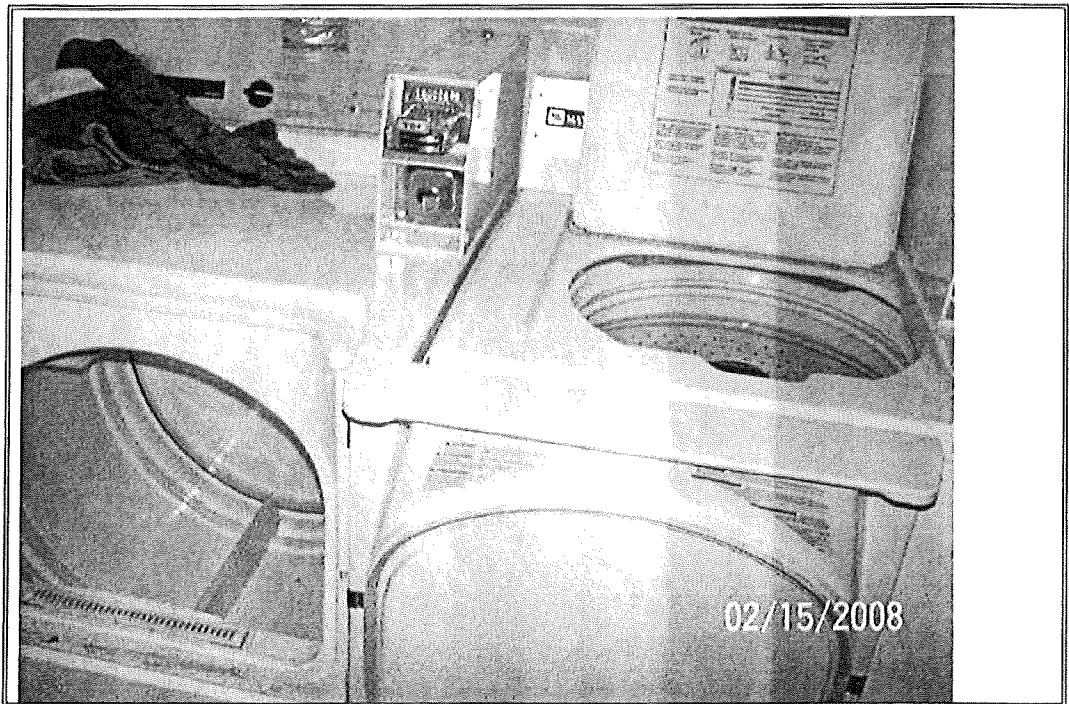
Photograph Number 30: Typical second and / or third floor laundry provisions.
