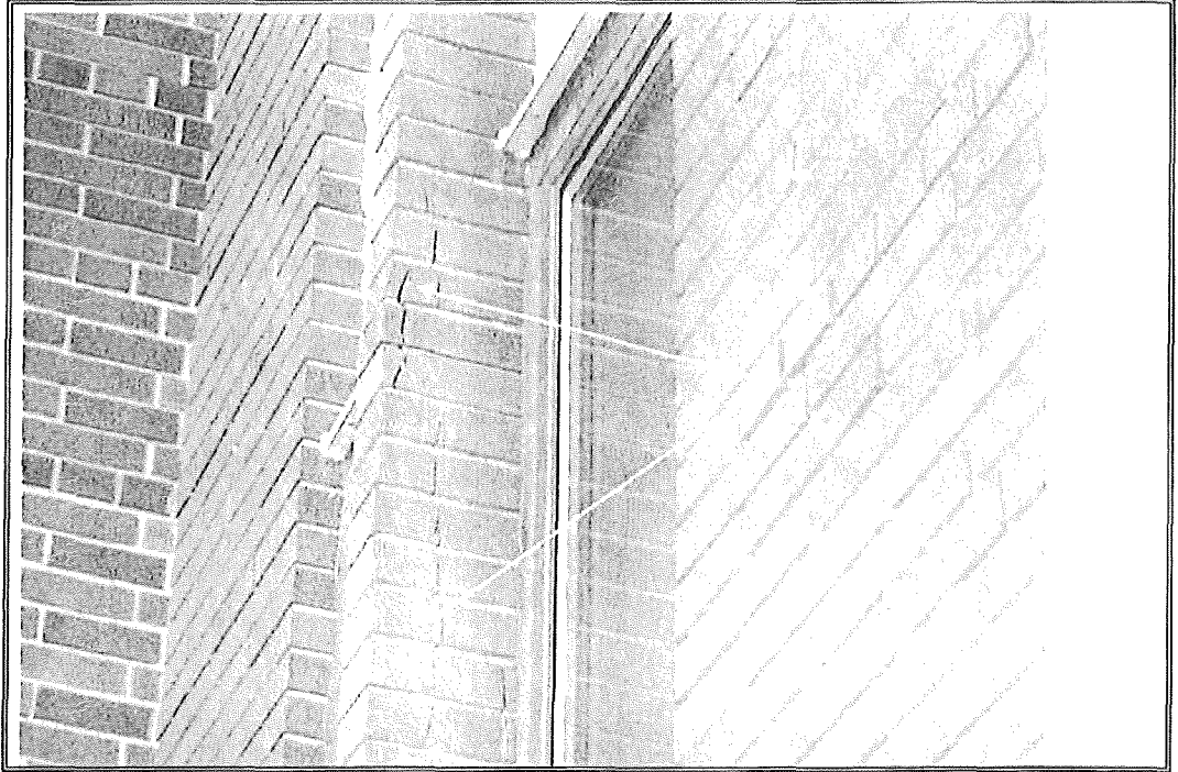
Photograph Number 9: Masonry veneer cracks and spalling.
