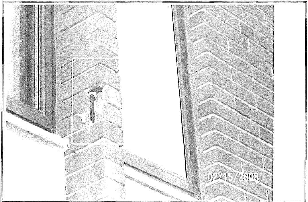
Photograph Number 10: Masonry veneer cracks and spalling.
