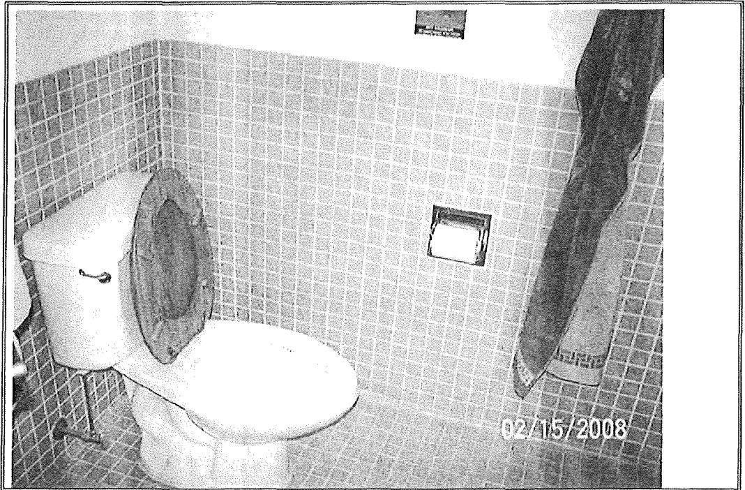
Photograph Number 33: Typical resident room ( suite ) bathroom provisions.
