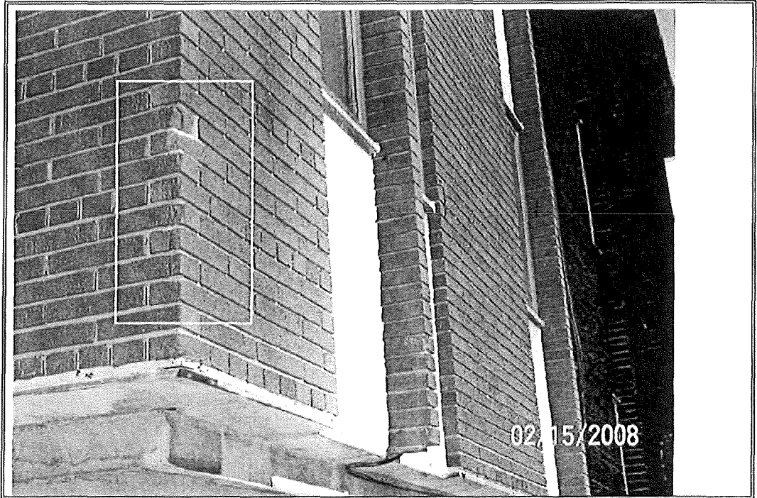
Photograph Number 13: Masonry veneer cracks and spalling.
