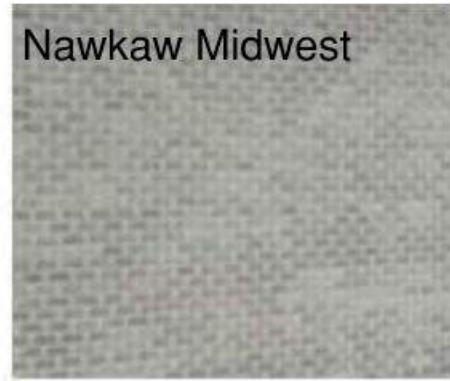
Existing Brick - Stained
