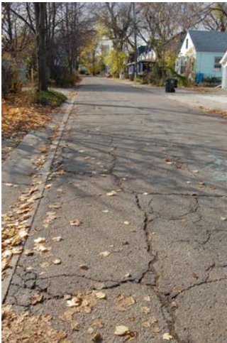
Curtis Ct looking Southwest (Deteriorating)
