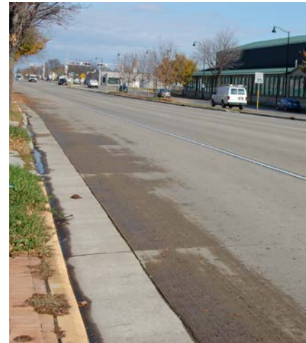
Washington at Baldwin looking Southwest (Good)
