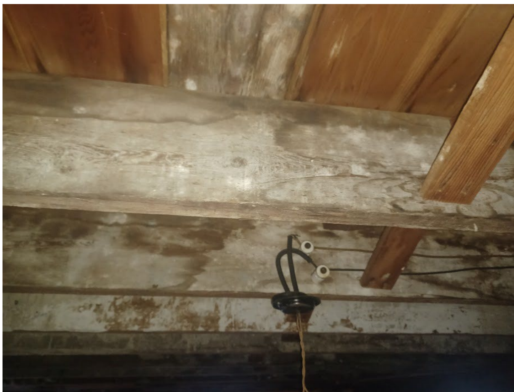
Photo 10. Molded support beams in upstairs storage, "knob and tube" wiring remnant
