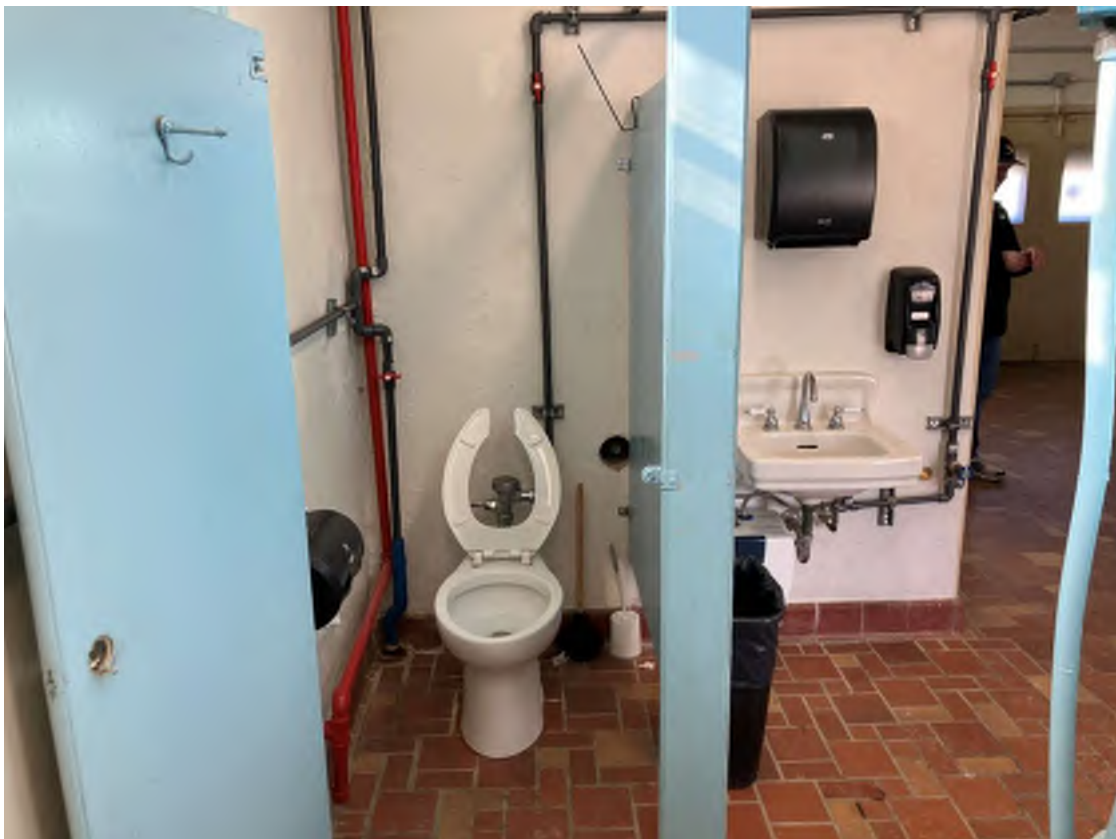
Interior of existing Wellhouse.
