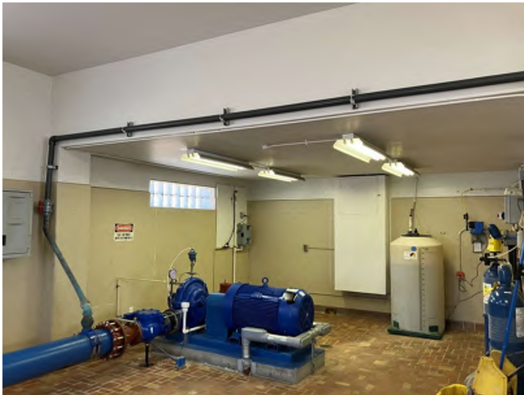
Interior of existing Wellhouse.
