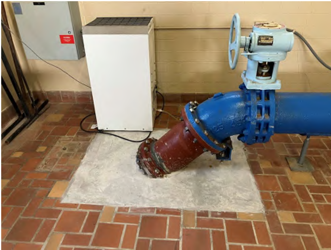
Interior of existing Wellhouse.
