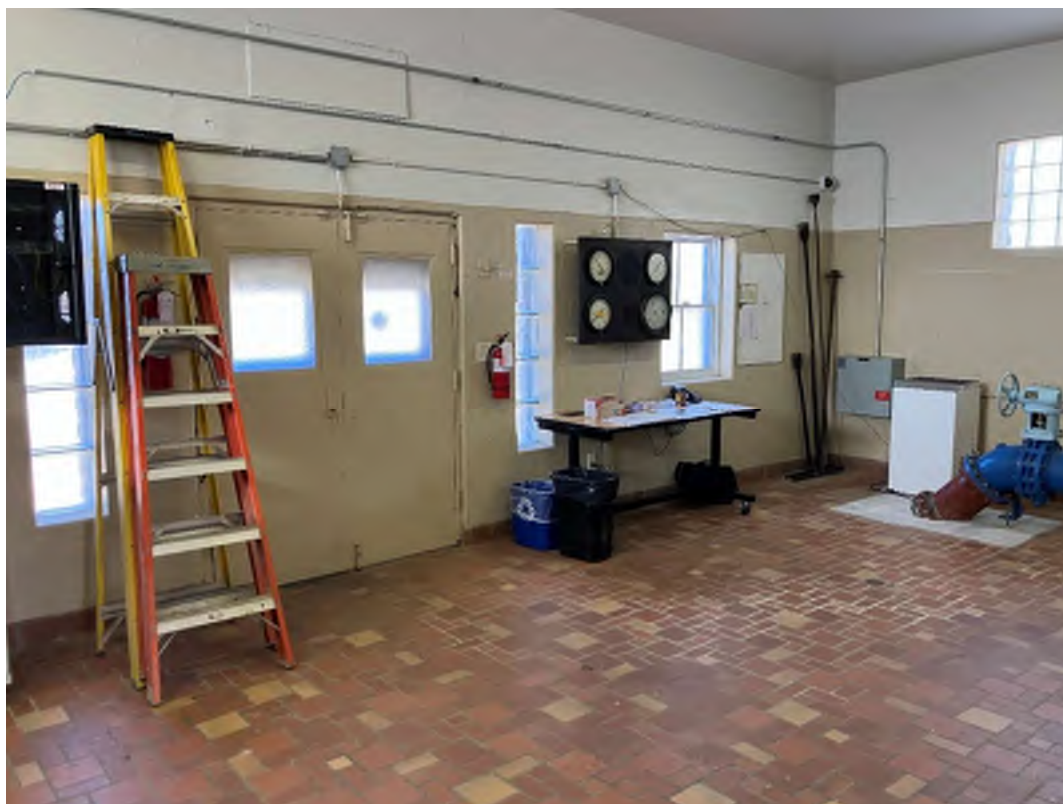
Interior of existing Wellhouse.
