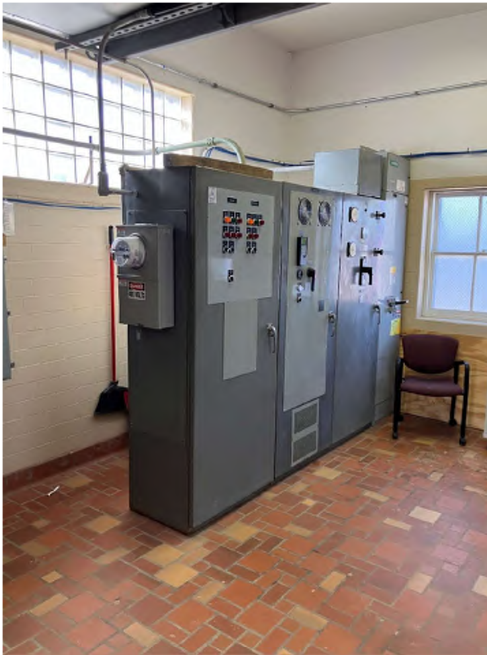
Interior of existing Wellhouse.
